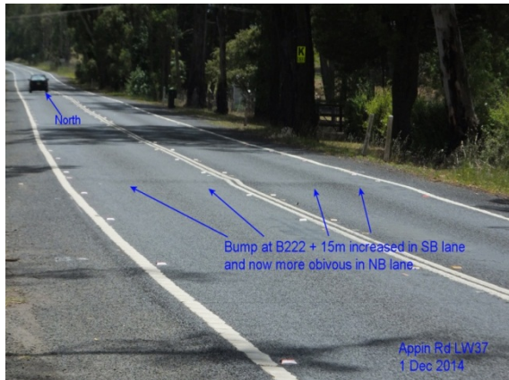
Photo 1: Bump at B222 + 15m, 1/12/2014 (Photo courtesy of Colin Dove).
