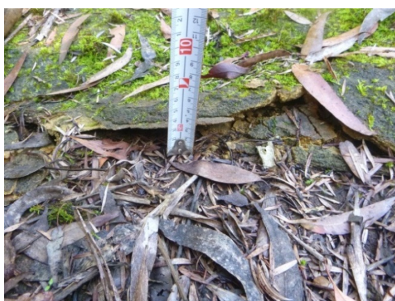
Photo 4: WCA5_LW36_001, fracturing and uplift of rock bed.
