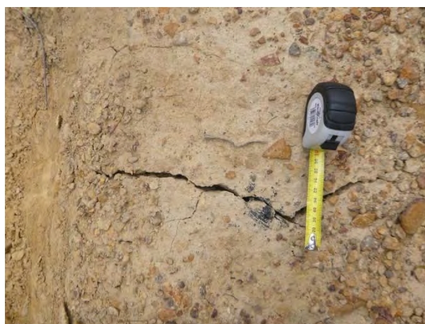
Photo 2: WCA5_LW38_006 – Soil crack at its widest point. Taken on 25/9/15
