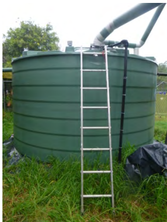
Photo 3: Outlet point/storage tank and sample point (12/06/13)
