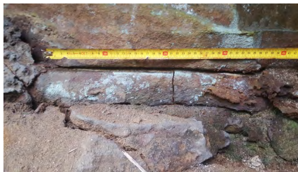
Photo 3: WCA5_LW38_010 – Fracture to base of rock outcropping. Taken on 17/02/16.
