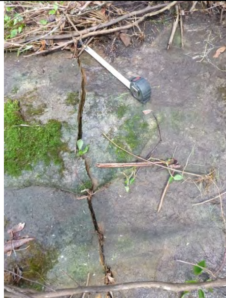
Photo 30: WCA5_LW38_001- upstream section of fracturing, extending in to sediment. Taken on 24/04/2015
