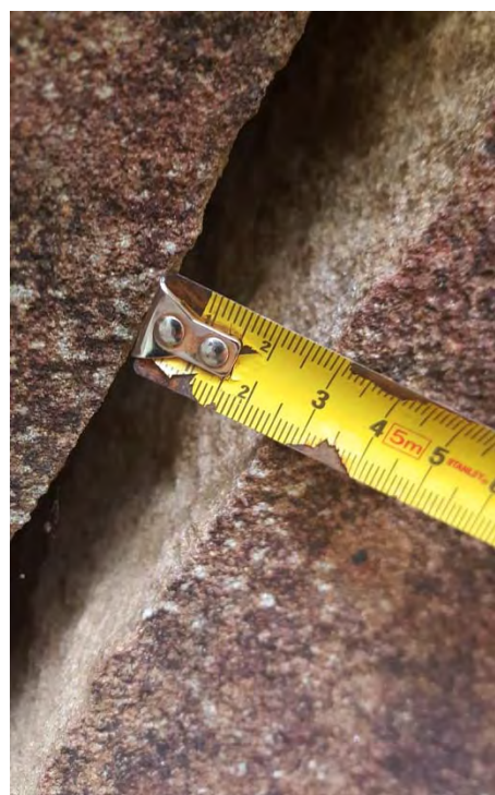
Photo 2: WA5_LW38_010 – vertical fracture. Taken on 17/02/16.
