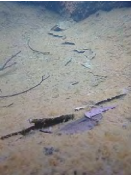
Photo 8: WCA5_LW38_005 – Fracturing and uplift on tributary GR108. Taken on 20/08/2015.
