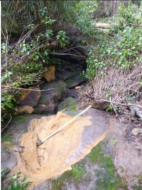
Photo 27: WCA5_LW38_001- fracturing and dislodged fragments, looking downstream. Taken on 24/04/2015
