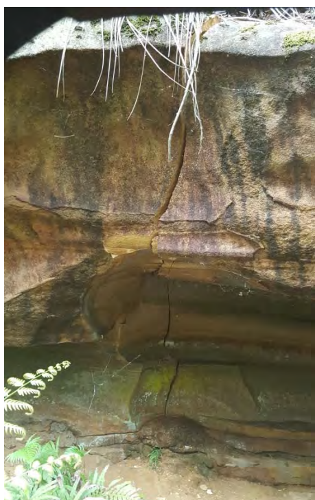
Photo 1: WCA5_LW38_010 – Vertical fracturing to rock outcrop adjacent to GR110. Taken on 17/02/16.
