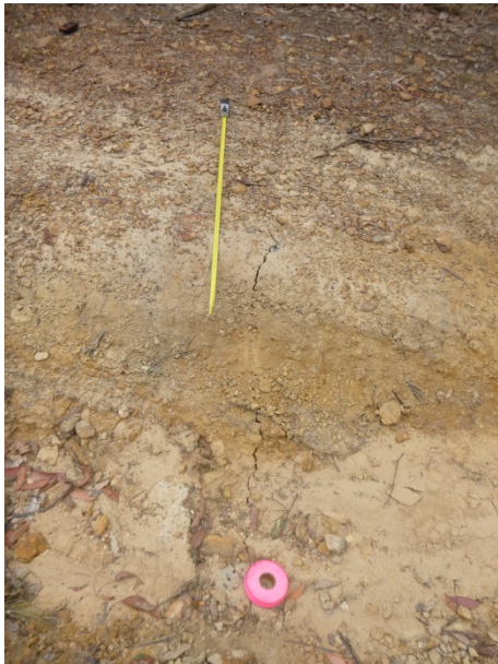
Photo 12: WCA5_LW38_006, soil crack looking across the access track. Taken on 25/09/15.
