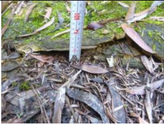
Photo 3: WCA5_LW36_001, fracturing and uplift of rock bed at GR104_Pool 1 looking south. Taken on 19/06/2014.
