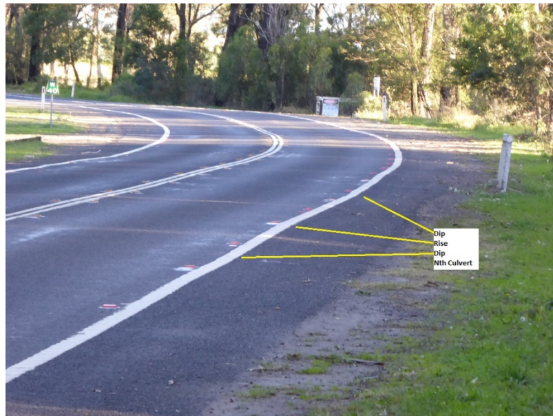
Fig. 3.3 Cracking in road shoulder at B230 + 19m, 4 th December 2014 (Courtesy of Colin Dove)
