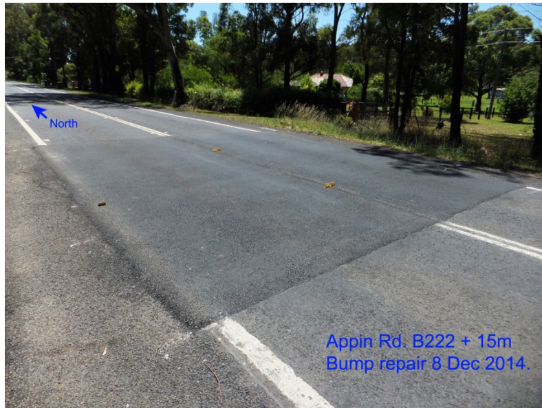
Fig. 3.2 Pavement repair at B222 + 15m, 8 th December 2014 (Courtesy of Colin Dove)
