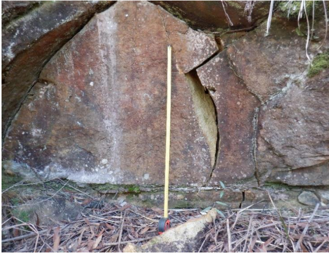
Photo 15: DA3B_LW18_013, Rock fracturing and rock fragmentation, northern slope of LA2 valley. Taken 16/8/2022.
