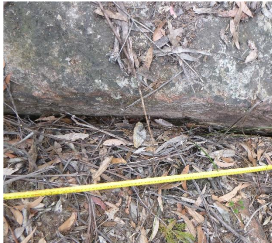
Photo 7: DA3B_LW18_005, Displacement between rock/soil and soil cracking west of Fire Road 6A. Taken 30/6/2022.
