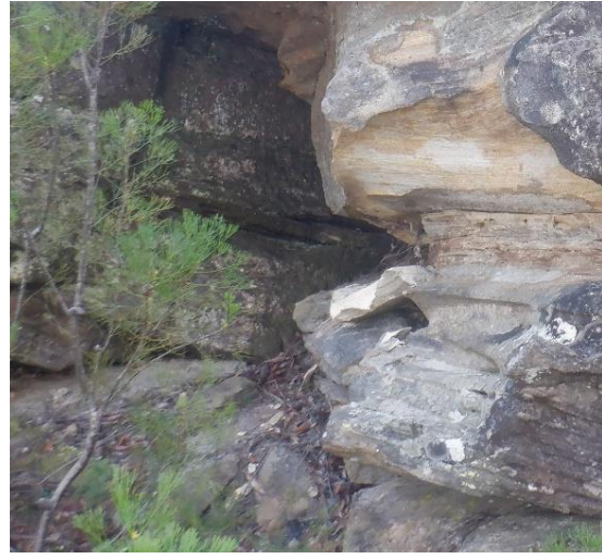
Photo 13: DA3B_LW18_011, Rockfall to 4m high rock outcrop, west of Fire Road 6A. Taken on 10/06/2022.
