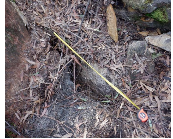
Photo 11: DA3B_LW18_009, rock fracturing, displacement and fragmentation in bushland near NDC1. Taken on 09/06/2022.
