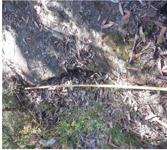
Photo 4: DA3B_LW18_002, Rock fracturing and soil cracking west of Fire Road 6A. Taken on 31/01/2022.
