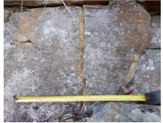
Photo 17: DA3B_LW18_015, Rock fracturing, northern slope of LA2 valley. Taken 16/8/2022.
