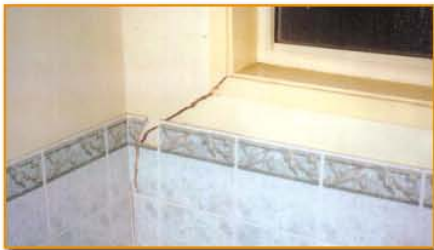
▲ Subsidence has caused internal cracking.
