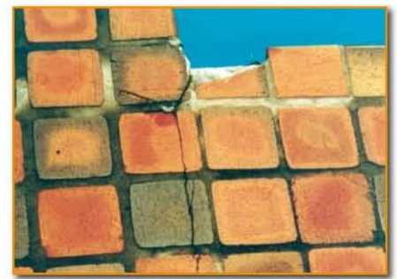
No expansion joint in pavers ▲
