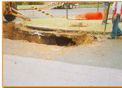
▲ Potholes from old abandoned mining are repaired by the Board where they present a public or private danger.
