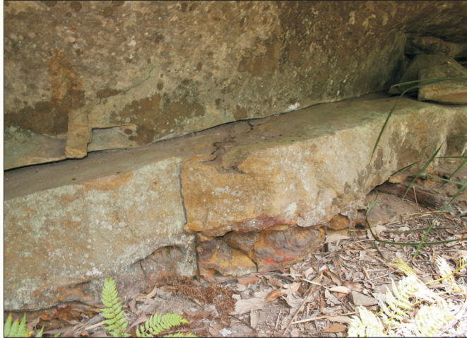
Plate 7a: Site D4 - Opening of Existing Crack in Rear Wall
