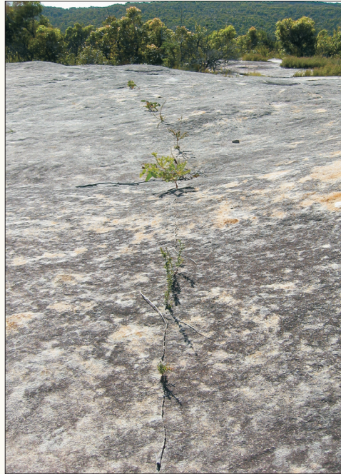
Plate 4: Site FRC 57 - Crack in Sandstone Platform
