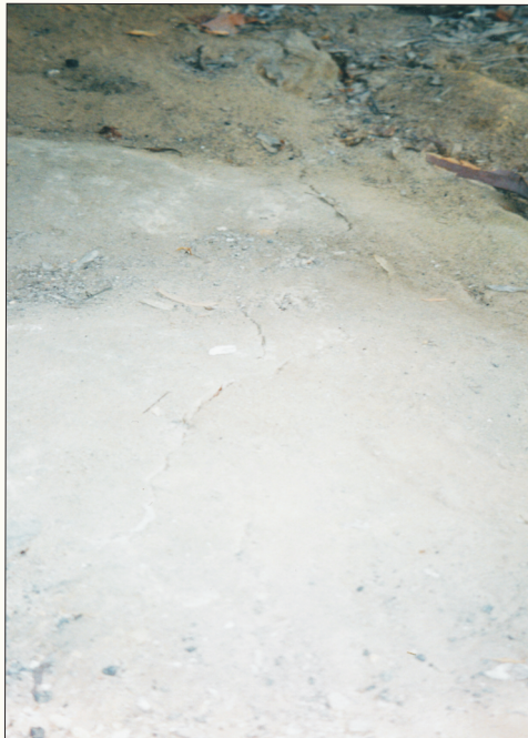
Plate 6b: Site 990 - Cracking in Floor of Shelter
