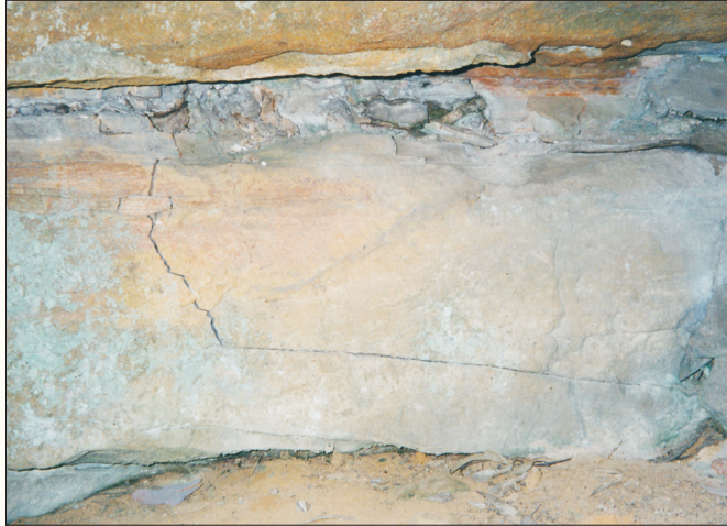
Plate 6a: Site 990 - Cracking in Rear Wall
