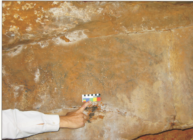
Plate 3b: Site FRC 49 - Cracking in Rear Wall
