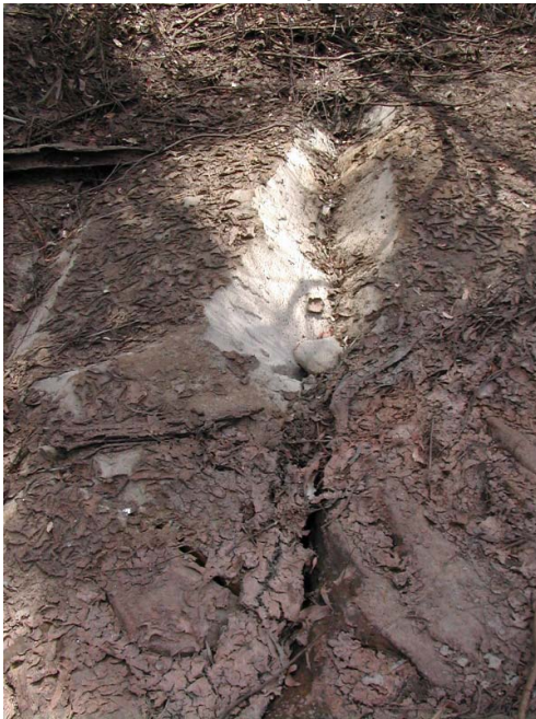
Figures 2a and 2b – Cracking of Rocks Under A Stream Because of the Mines
