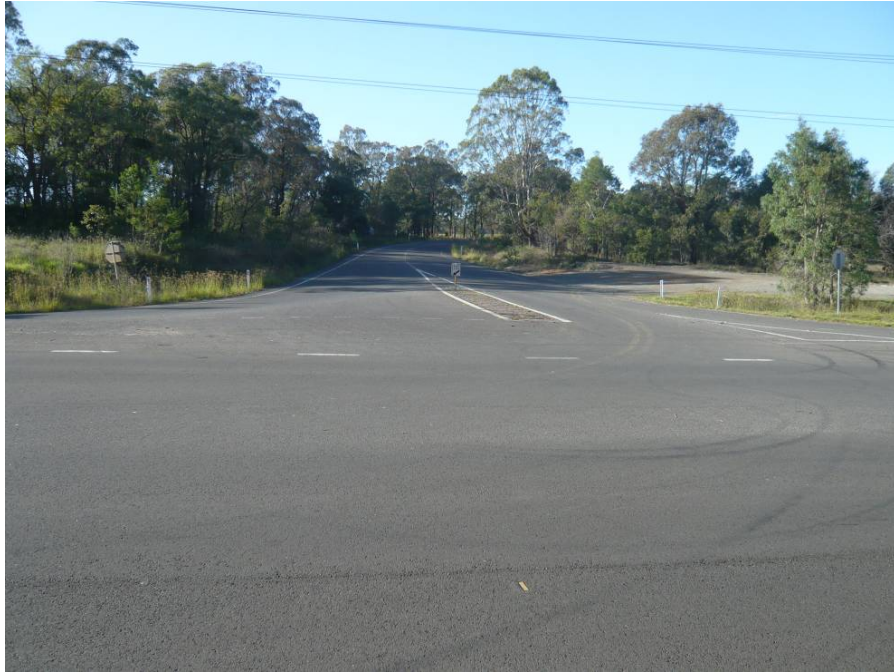
View looking south along Macarthur Road from its intersection with Wilton Road.
