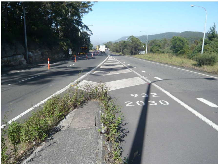
View looking south at the interchange of southbound lanes of Appin Road and Mount Ousley Road.
