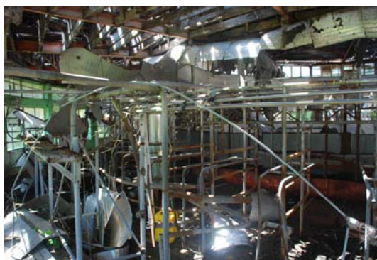
Rotolactor showing collapsing roof structure. Photo: M. Pearson 2008
