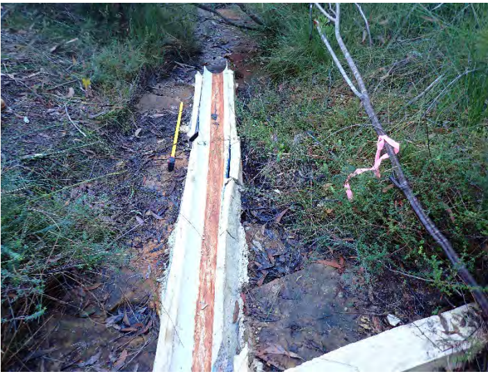
Photo 3: DA3C_LW21_014 , damage to concrete footing of flow monitoring site WC20S2. Taken on 11/07/2023.
