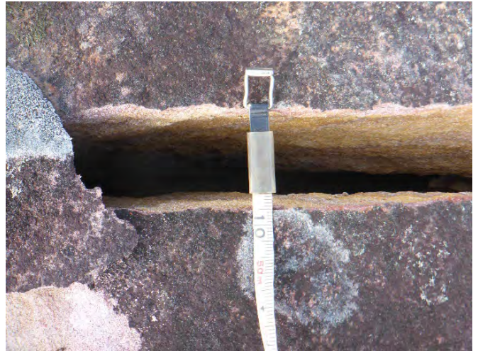
Photo 13: DA3C_LW21_004, rock fracture width. Taken on 06/06/2023
