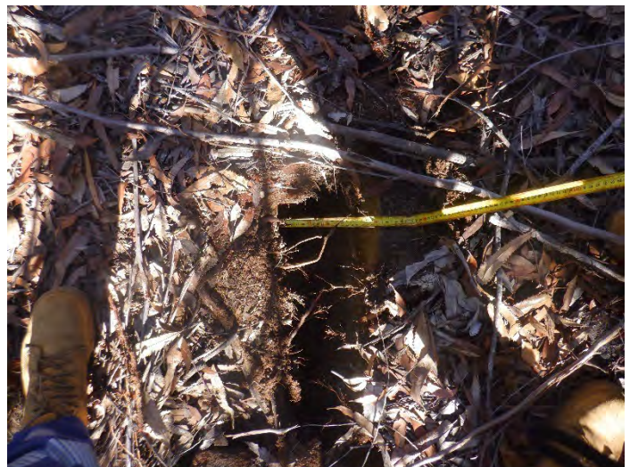
Photo 8: DA3C_LW21_010 , maximum width of the rock fracture. Taken on 19/06/2023.
