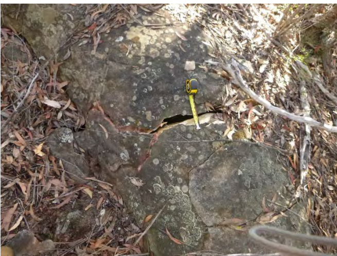
Photo 1: DA3C_LW21_005 , fracture to rock outcrop. Taken on 15/06/2023.
