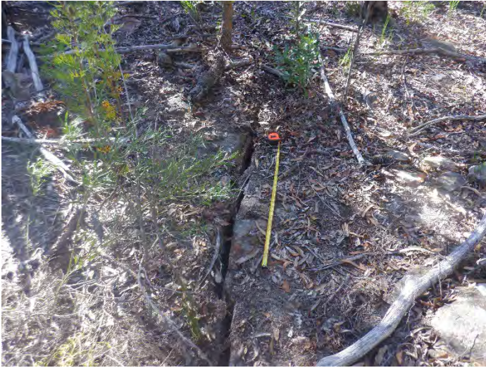
Photo 10: DA3C_LW21_011, section of rock fracturing. Taken on 19/06/2023.
