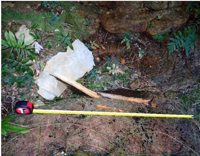
Photo 7: DA3C_LW21_016, fragments of rockfall from step. Taken on 11/07/2023.
