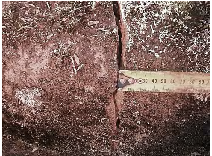
Photo 5: DA3C_LW21_009 , maximum width of the rock fracture. Taken on 19/06/2023.
