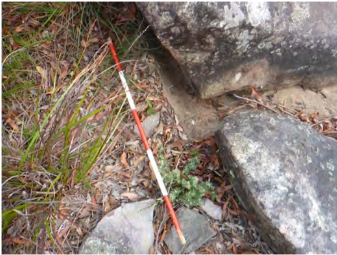
Photo 5: DA3C_LW21_002, showing rock movement on largest fracture. Taken on 6/06/2023.
