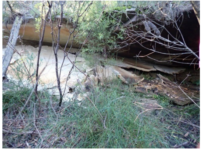
Photo 77: DA3C_LW21_016 , looking at the rockfall. Taken on 26/07/2023.
