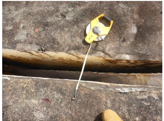
Photo 43: DA3C_LW21_003, width of rock fracture. Taken on 06/06/2023.
