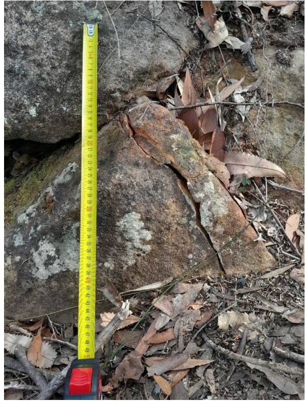
Photo 108: DA3C_LW21_031, overview of rock fracture. Taken: 12/09/2023. Note - measurement tape set to 0.5m for scale.
