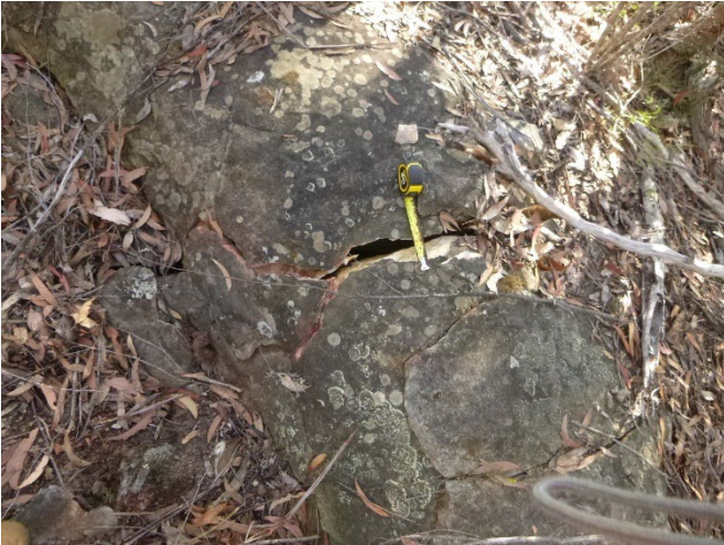
Photo 48: DA3C_LW21_005 , fracture to rock outcrop. Taken on 15/06/2023.
