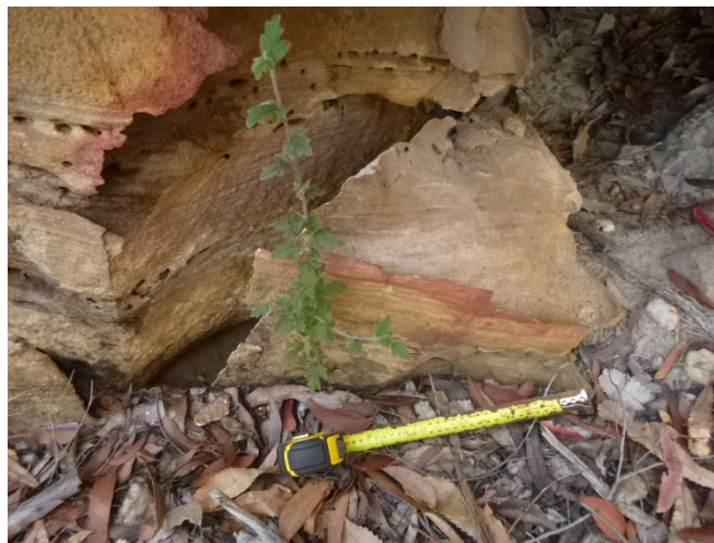
Photo 54: DA3C_LW21_007, rock fall. Taken on 15/06/2023.
