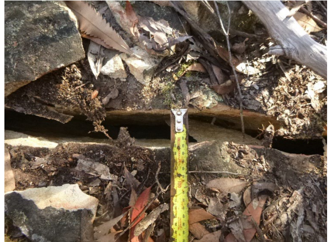
Photo 49: DA3C_LW21_005 , showing width of rock fracture. Taken on 15/06/2023.
