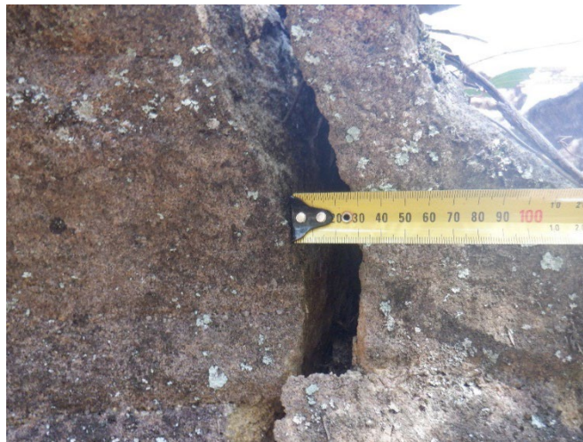
Photo 83: DA3C_LW21_019, looking at the width of the rock fracture. Taken on 1/08/2023.
