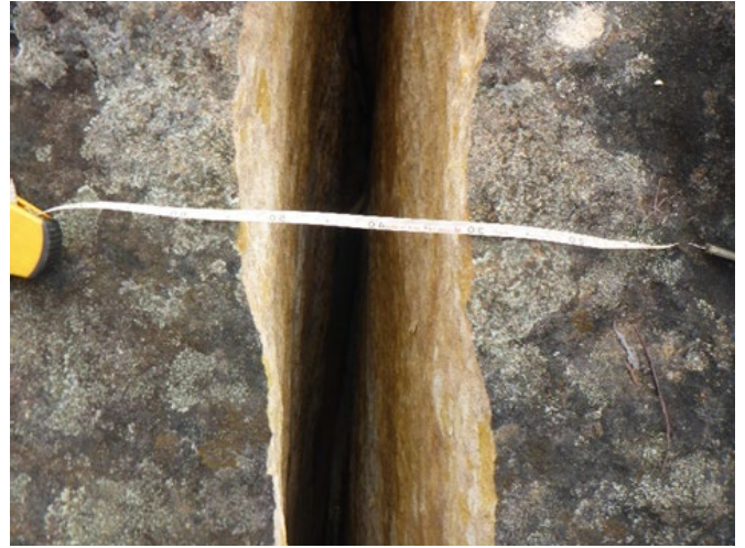
Photo 38: DA3C_LW21_002, showing maximum rock fracture width. Taken on 06/06/2023.
