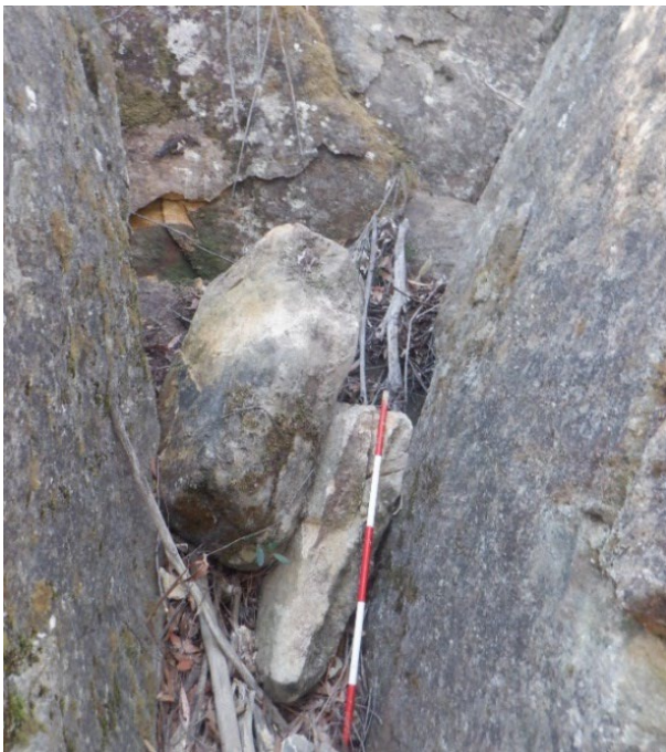
Photo 97: DA3C_LW21_026, section of rock fracture and rockfall. Taken 06/09/2023.
