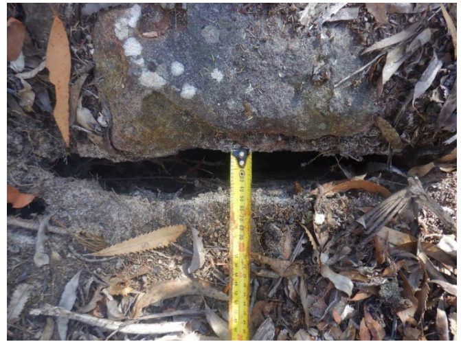
Photo 65: DA3C_LW21_011, maximum width of the fracture. Taken on 19/06/2023.
