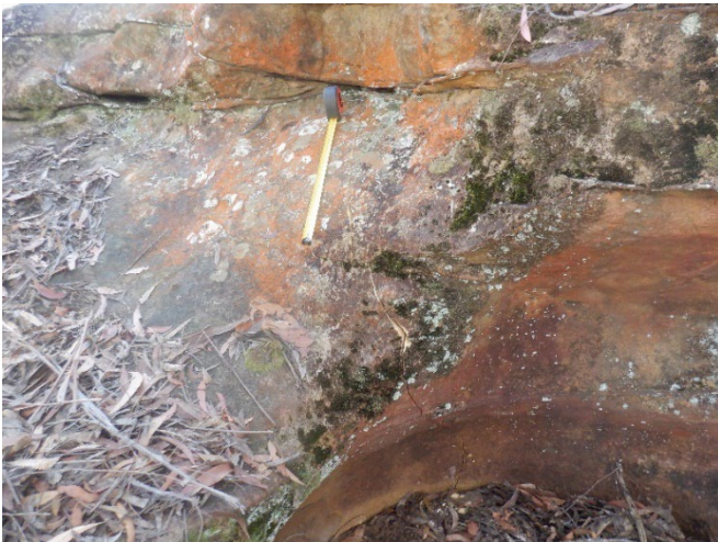
Photo 80: DA3C_LW21_018, overview of rock fracturing. Taken on 26/07/2023.
