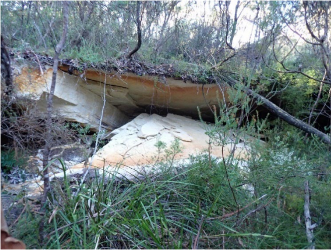
Photo 76: DA3C_LW21_016 , looking at the rockfall. Taken on 26/07/2023.
