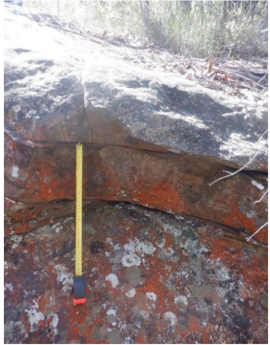
Photo 79: DA3C_LW21_018, section of rock fracturing. 26/07/2023.
