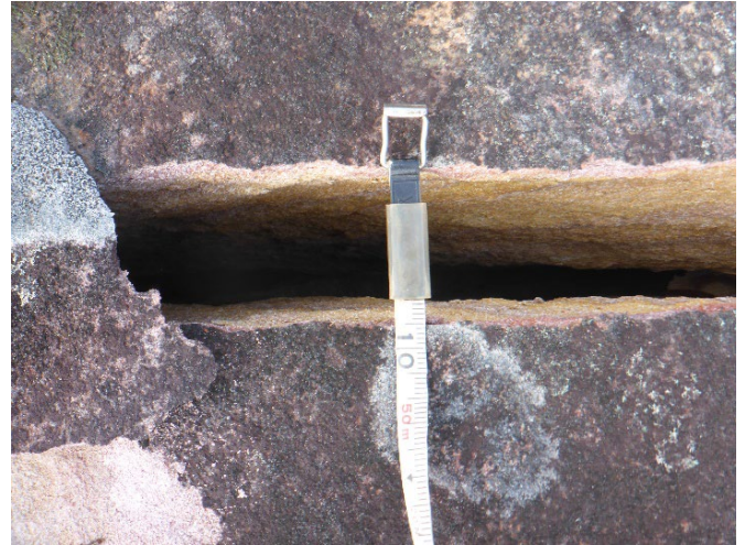
Photo 47: DA3C_LW21_004, rock fracture width. Taken on 06/06/2023.
