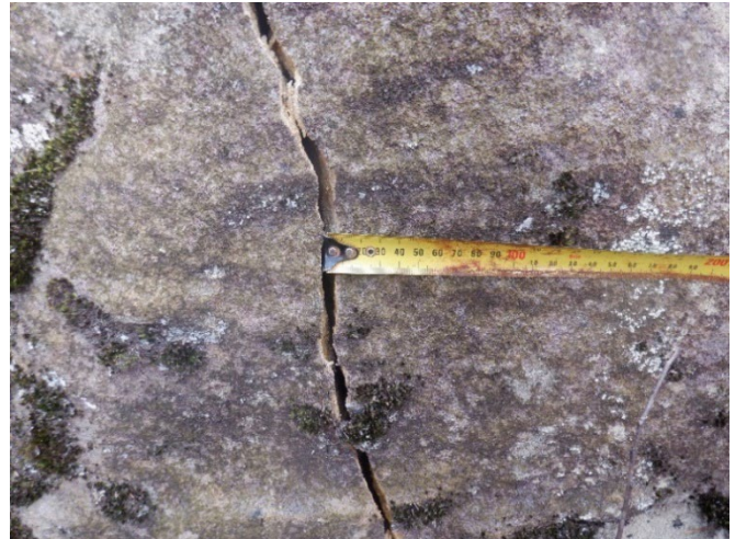
Photo 69: DA3C_LW21_012, maximum width of the rock fracture. Taken on 27/06/2023.
