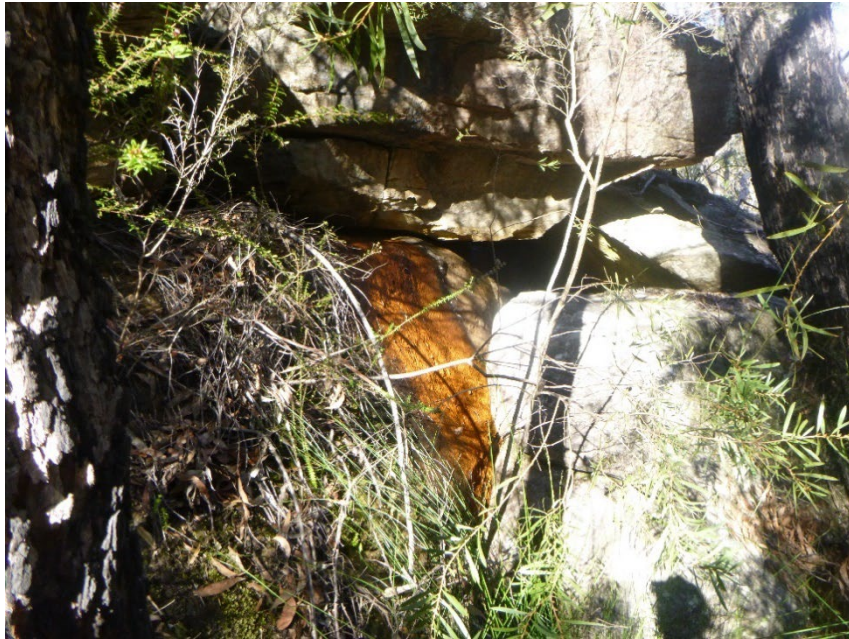
Photo 31: DA3C_LW21_021 , overview of the iron staining. Taken on 1/08/2023.
