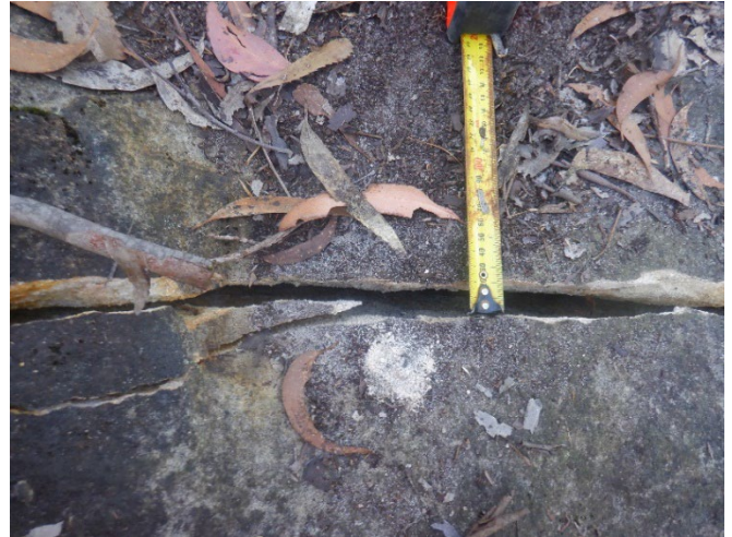
Photo 56: DA3C_LW21_008, maximum width of the rock fracture. Taken on 19/06/2023.
