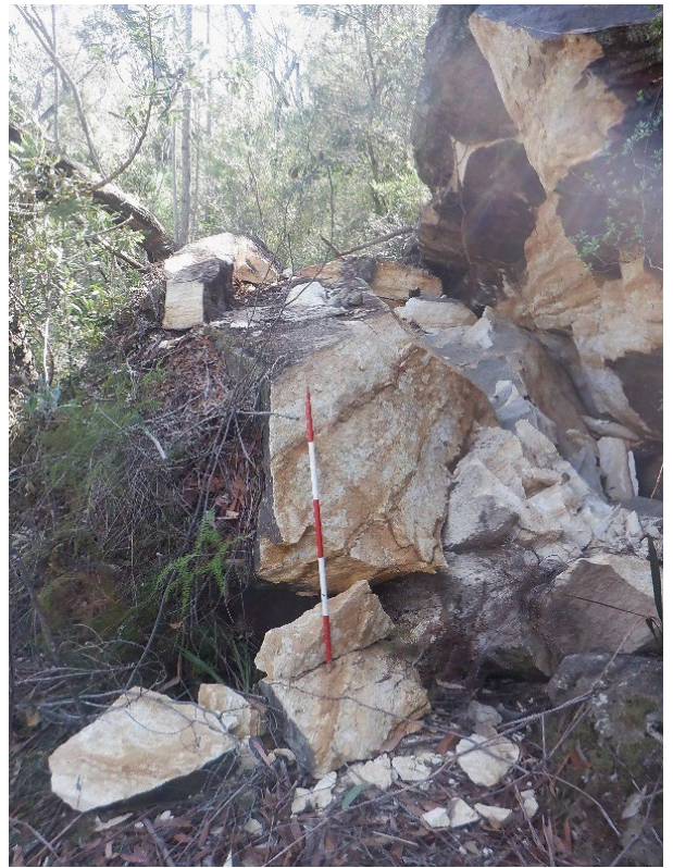
Photo 100: DA3C_LW21_027, overview of rockfall. Taken 06/09/2023.
