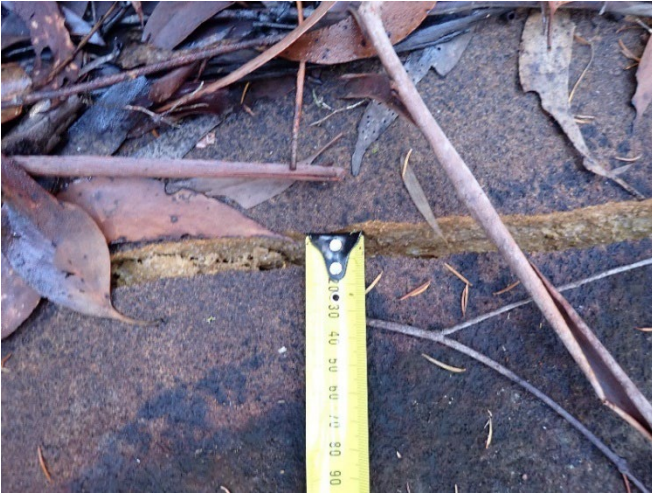
Photo 27: DA3C_LW21_017, width of the rock fracture. Taken on 26/07/2023.
