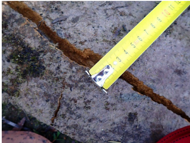
Photo 26: DA3C_LW21_015 , width of rock fracture. Taken on 11/07/2023.
