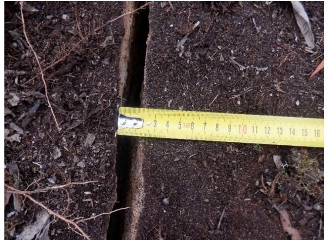
Photo 72: DA3C_LW21_013, maximum width of the rock fracture. Taken on 03/07/2023.
