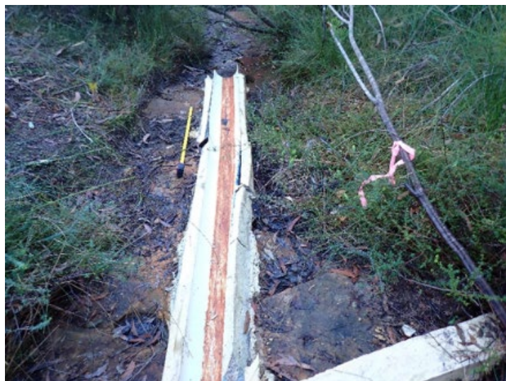
Photo 23: DA3C_LW21_014 , damage to concrete footing of flow monitoring site WC20S2 . Taken on 11/07/2023.
