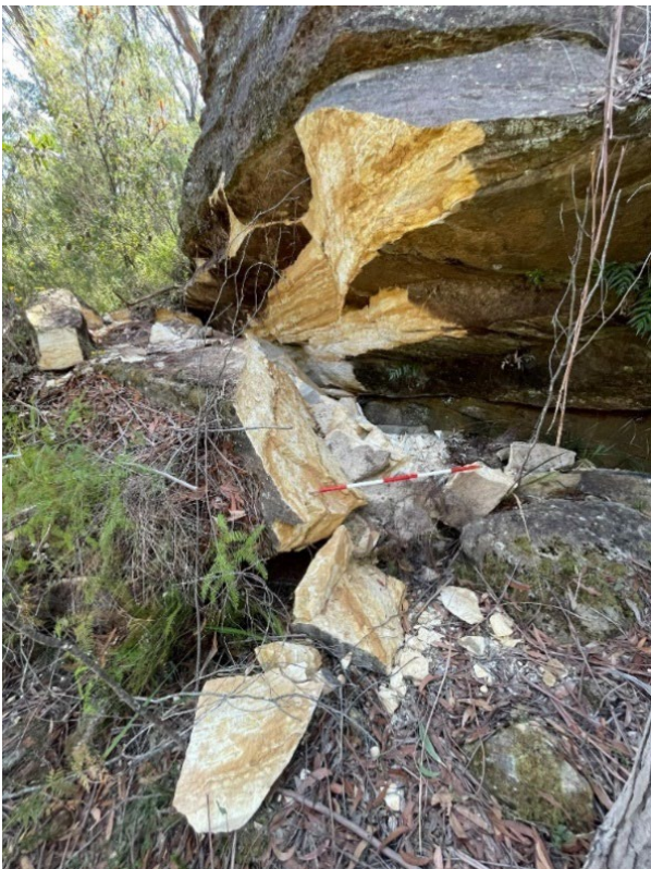
Photo 99: DA3C_LW21_027, overview of rockfall. Taken 06/09/2023.
