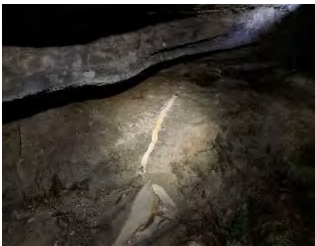
Plate 17: WC15 bedrock cracking
