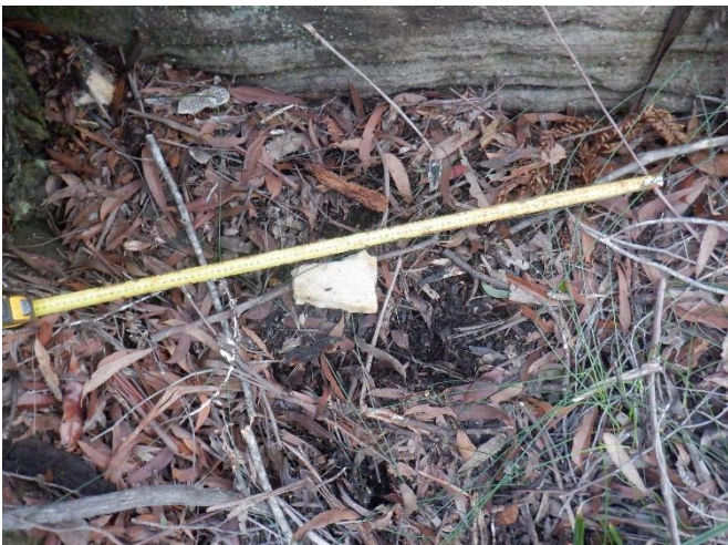
Photo 155: DA3A_LW19_055, showing area of rockfall. Taken on 4/5/2023.
