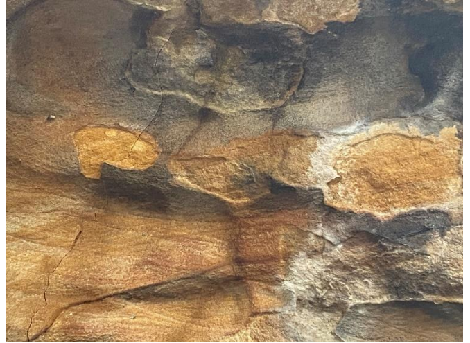
Photo 125: DA3A_LW19_038, rock fracturing extending to the upper part of overhang. Taken on 28/03/2023.
