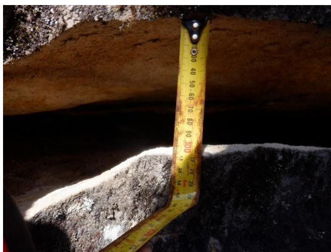
Photo 39: DA3A_LW19_002 , showing width of rock fracturing. Taken 19/04/2023.
