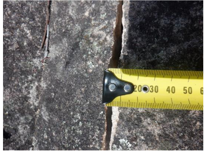
Photo 64: DA3A_LW19_012 , width of rock fracturing. Taken on 7/11/2022.
