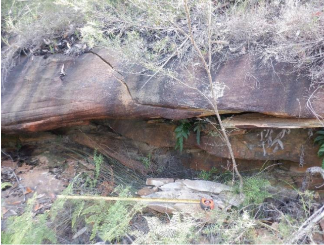
Photo 99: DA3A_LW19_027, section of rock fracturing and rockfall. Taken on 10/01/2023.
