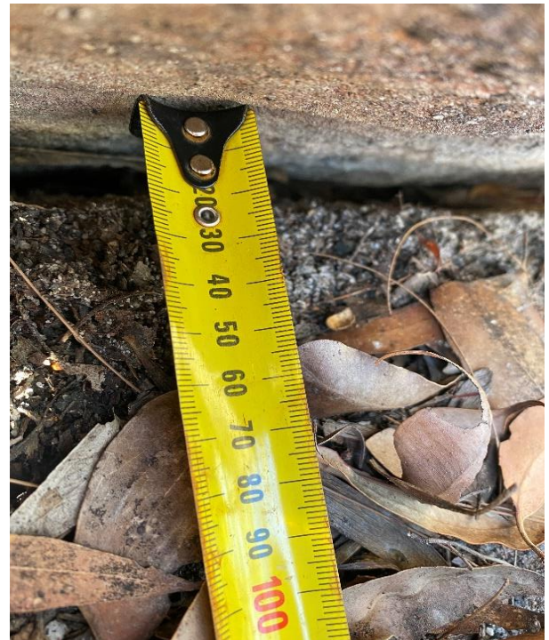
Photo 77: DA3A_LW19_018, width of rock displacement. Taken on 13/12/2022.
