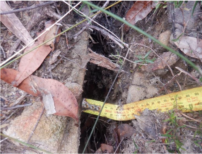
Photo 48: DA3A_LW19_007 , width of soil cracking. Taken on 18/10/2022.
