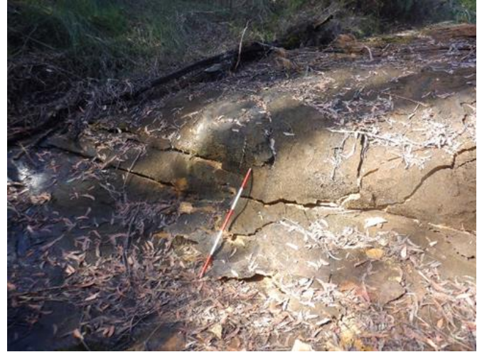
Photo 23: DA3A_LW19_043, looking upstream at rock fracturing on rockbar. Taken 17/04/2023.
