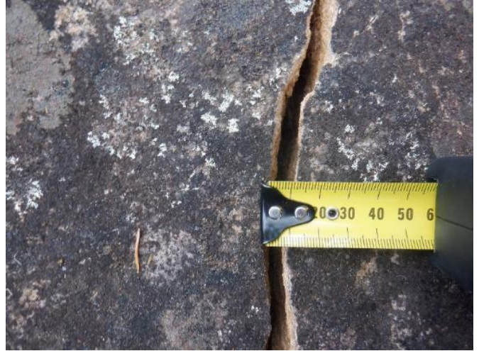
Photo 60: DA3A_LW19_010, width of rock fracturing. Taken on 7/11/2022.
