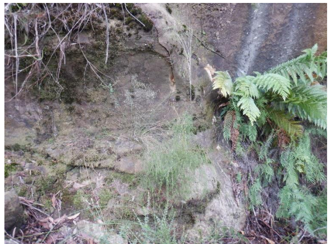
Photo 152: DA3A_LW19_053, showing rock fracturing. Taken on 4/5/2023
