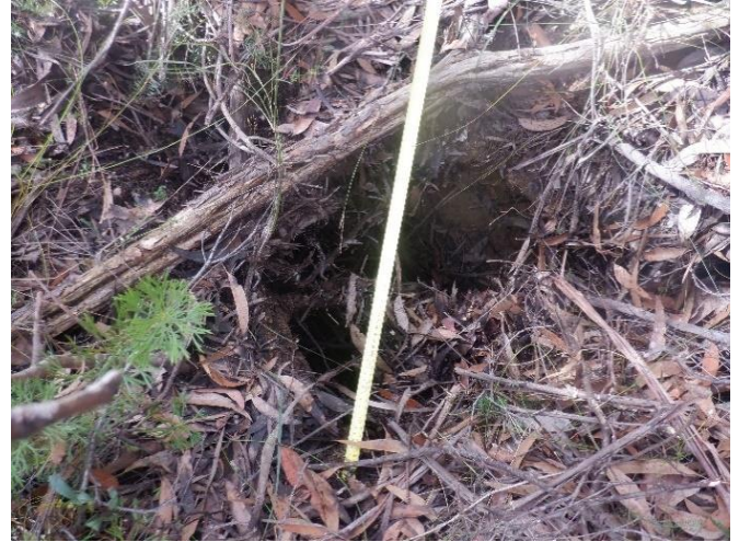
Photo 46: Width of surface erosion. Taken 31/08/2022.
