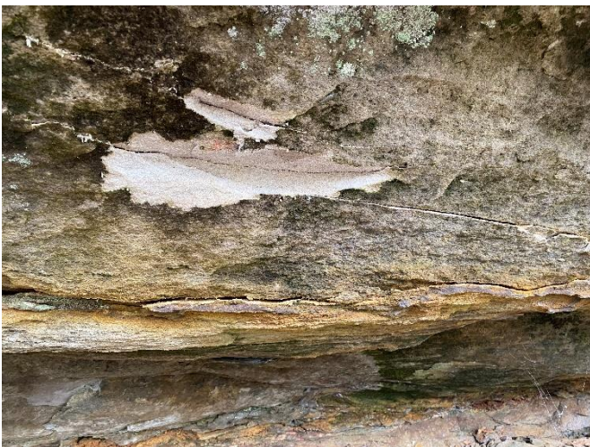
Photo 118: DA3A_LW19_037, rock fall. Taken on 28/03/2023.
