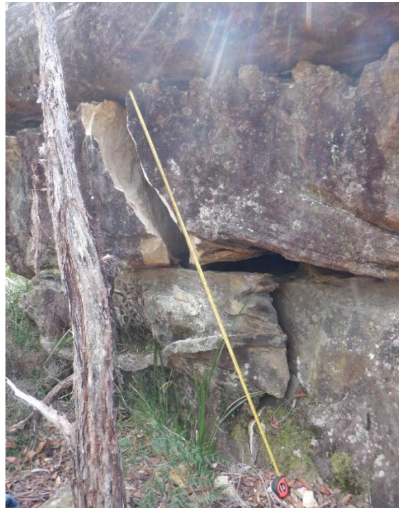
Photo 70: DA3A_LW19_015, section of rock fracturing. Measuring tape set at 2.3m. Taken on 19/04/2023.
