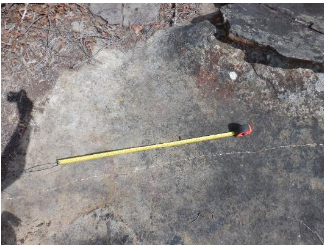
Photo 61: DA3A_LW19_011, section of rock fracturing. Taken on 7/11/2022.
