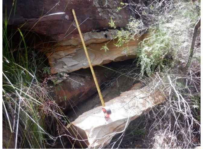
Photo 100: DA3A_LW19_027, section of rock fracturing and rockfall. Taken on 10/01/2023.
