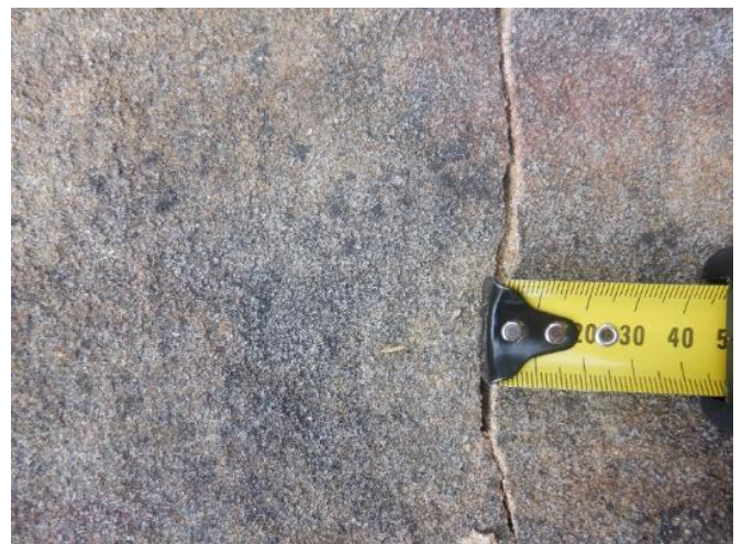
Photo 62: DA3A_LW19_011, width of rock fracturing. Taken on 7/11/2022.
