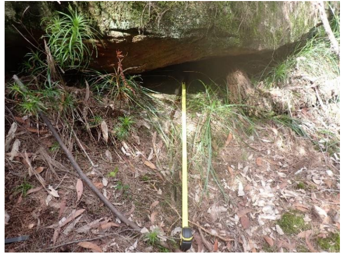
Photo 27: DA3A_LW8_003, looking at the extent of rock fracturing. Taken 12/04/2023.
