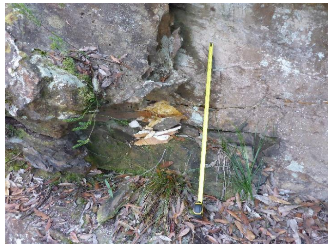
Photo 164: DA3A_LW19_059 , showing fallen debris. Taken on 5/05/2023.
