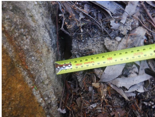
Photo 184: DA3A_LW19_048, showing rock movement. Taken on 27/04/2023.
