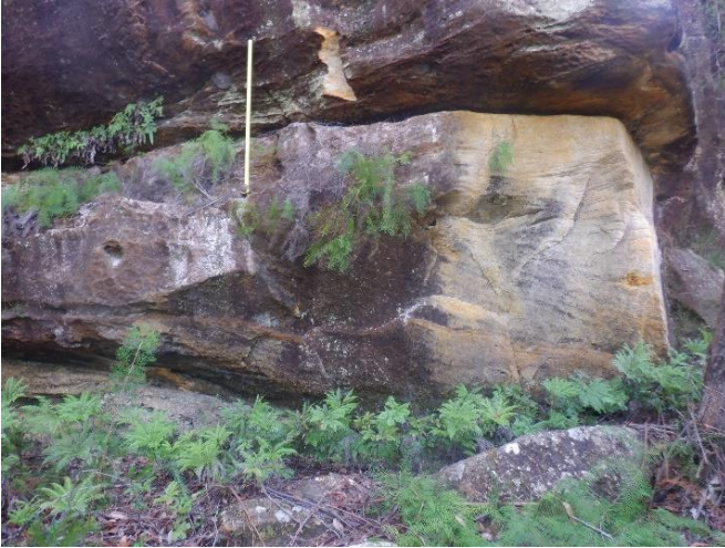
Photo 147: DA3A_LW19_047, showing steep slope/ step where rock has detached from rock face. Taken on 27/04/2023.
