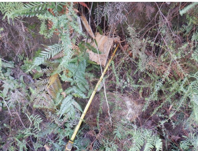
Photo 149: DA3A_LW19_052, showing area of rockfall. Taken on 4/5/2023.
