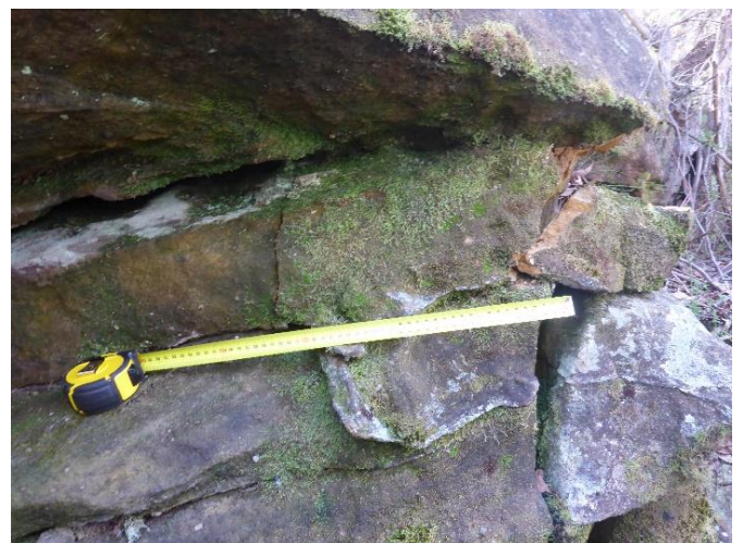
Photo 162: DA3A_LW19_058, showing step where rock has detached from rock face. Taken on 5/05/2023. Note: Tape measure is set to 0.5m in length.
