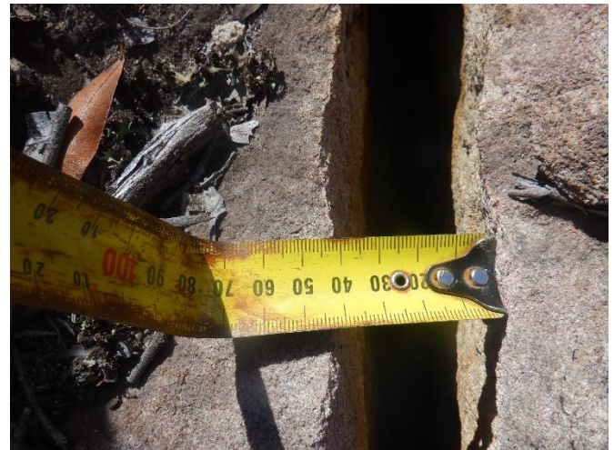
Photo 55: DA3A_LW19_008, width of rock fracturing taken on 09/05/2023.
