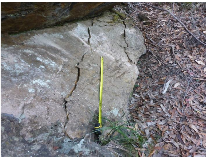
Photo 163: DA3A_LW19_059 , showing rock fracturing. Taken on 5/05/2023.
