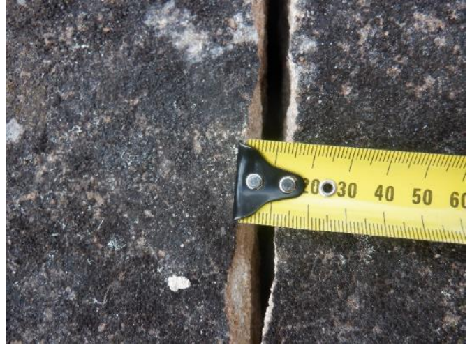
Photo 57: DA3A_LW19_009, width of rock fracturing. Taken on 7/11/2022.
