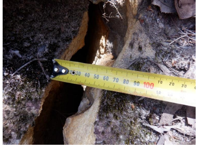
Photo 92: DA3A_LW19_023 , width of rock displacement. Taken on 13/12/2022.
