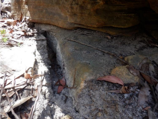
Photo 83: DA3A_LW19_021, section of soil cracking. Taken on 13/12/2022.
