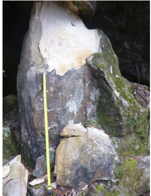
Photo 114: DA3A_LW19_033, rock fall from edge of steep slope. Taken on 15/2/2023.
