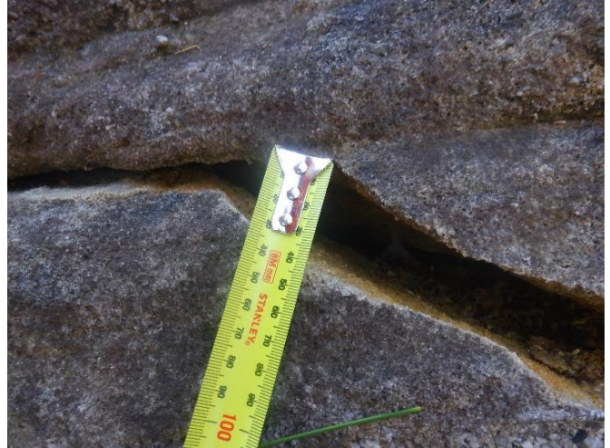
Photo 183: DA3A_LW19_048, showing width of rock fracture. Taken on 27/04/2023.
