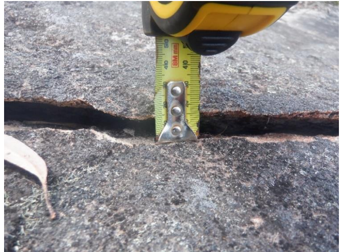
Photo 104: DA3A_LW19_028, width of rock fracturing. Taken on 6/02/2023.
