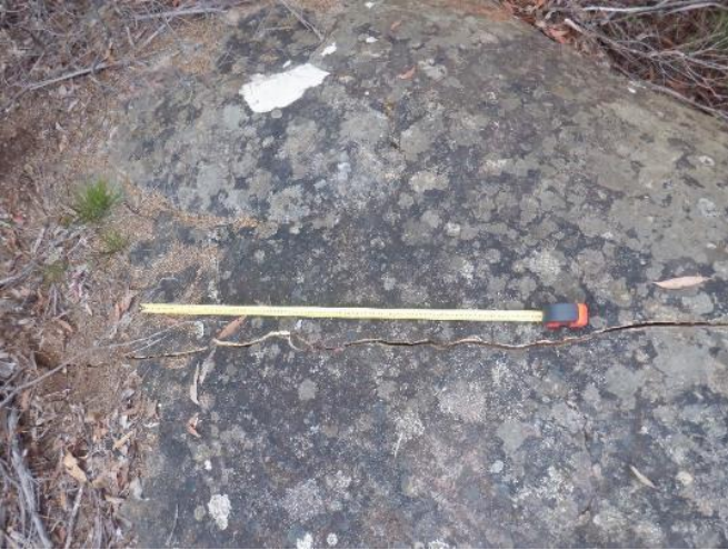
Photo 59: DA3A_LW19_010, section of rock fracturing. Taken on 7/11/2022.
