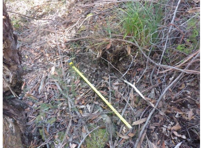
Photo 169: DA3A_LW19_061, showing extent of soil crack. Taken on 05/05/2023.
