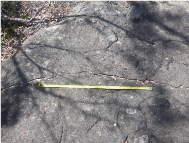
Photo 103: DA3A_LW19_028, section of rock fracturing. Taken on 6/02/2023.
