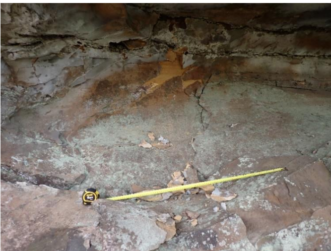
Photo 140: DA3A_LW19_042 looking at rockfall and associated fragments. Taken 12/04/2023.
