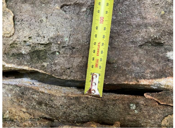
Photo 117: DA3A_LW19_037, rock fracturing. Taken on 28/03/2023.
