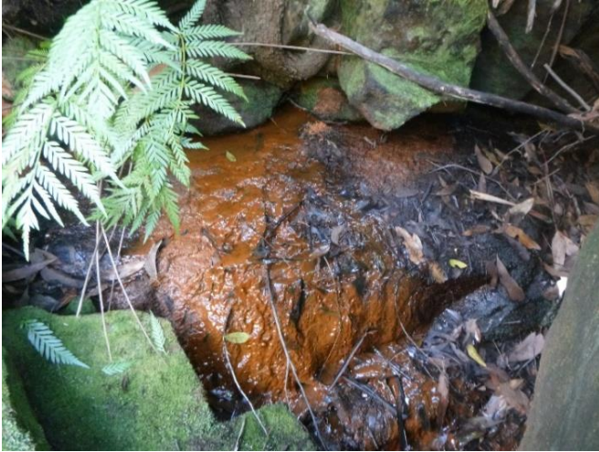
Photo 32: DA3A_LW19_045, showing iron staining appearing at base of a step. Taken on 26/04/2023.
