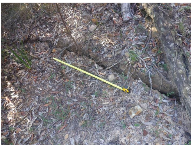
Photo 187: DA3A_LW19_050, showing extent of soil crack. Taken on 27/04/2023.
