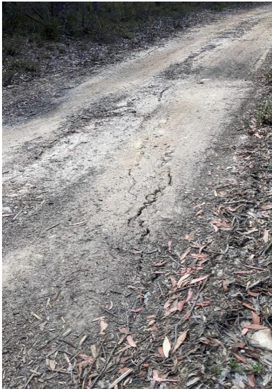
Photo 174: DA3A_LW19_026, section of soil cracking. Taken on 21/12/2022.
