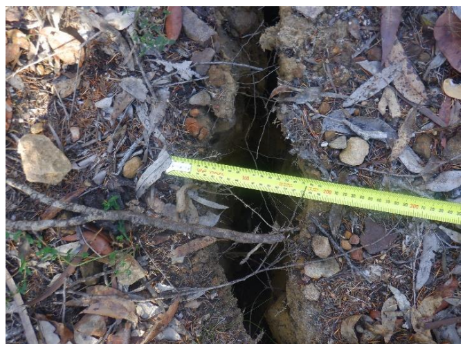
Photo 188: DA3A_LW19_050, showing width of soil crack. Taken on 27/04/2023.
