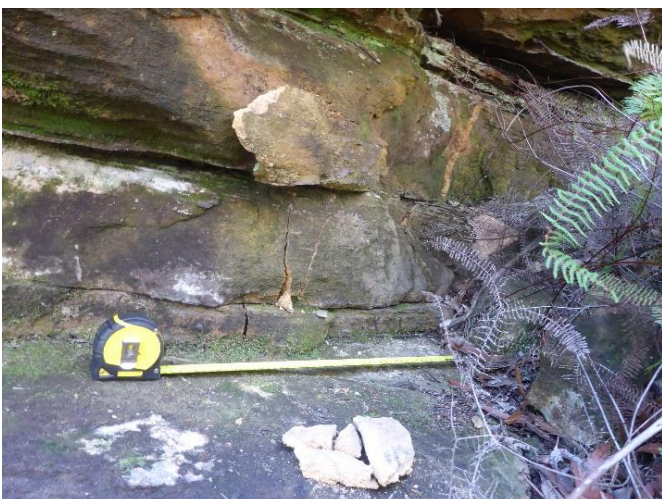
Photo 161: DA3A_LW19_058, showing step where rock has detached from rock face. Taken on 5/05/2023. Note: Tape measure is set to 0.5m in length.
