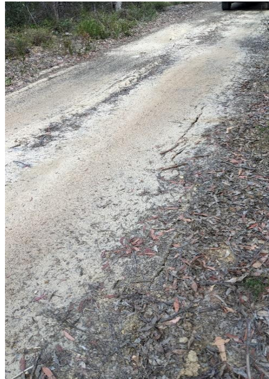
Photo 175: DA3A_LW19_026, section of soil cracking. Taken on 21/12/2022.
