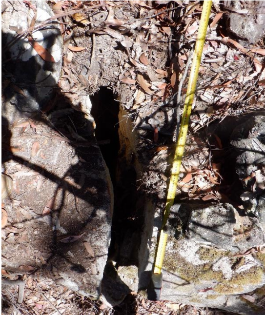
Photo 87: DA3A_LW19_022 , section of rock fracturing. Taken on 13/12/2022.
