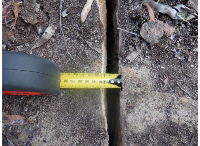
Photo 53: DA3A_LW19_008, width of rock fracturing. Taken on 7/11/2022.
