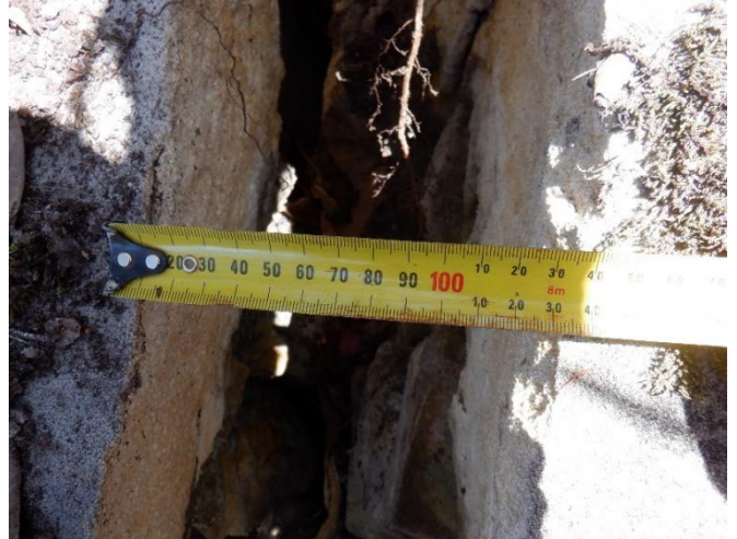
Photo 88: DA3A_LW19_022 , width of rock fracturing. Taken on 13/12/2022.
