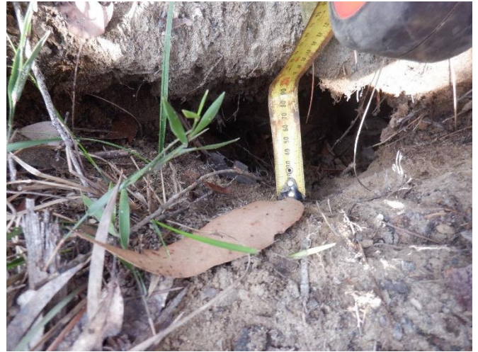
Photo 49: DA3A_LW19_007 , width of soil cracking. Taken on 19/04/2023.
