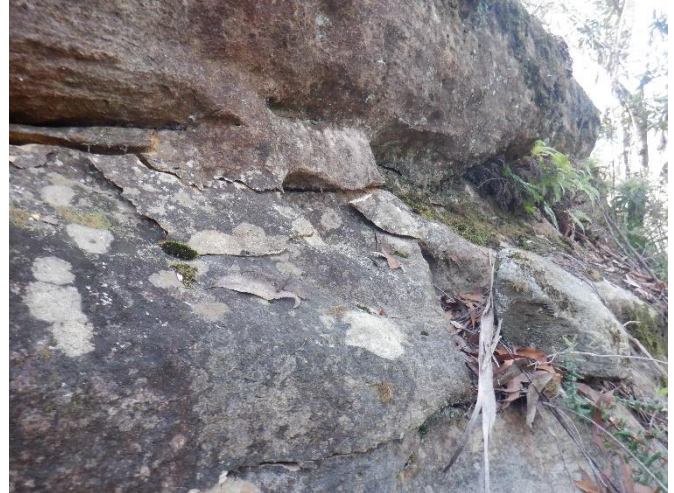
Photo 154: DA3A_LW19_054, showing rock fracturing and fragmentation. Taken on 4/5/2023.
