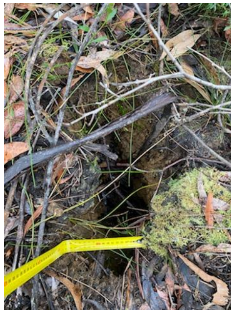
Photo 47: Width of soil crack. Taken 1/09/2022.
