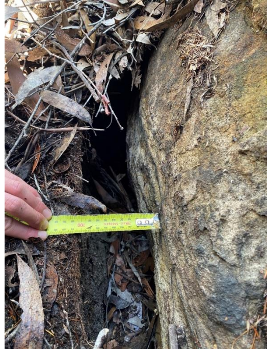
Photo 177: DA3A_LW19_035, width of the soil cracking/rock displacement. Taken on 16/03/2023.
