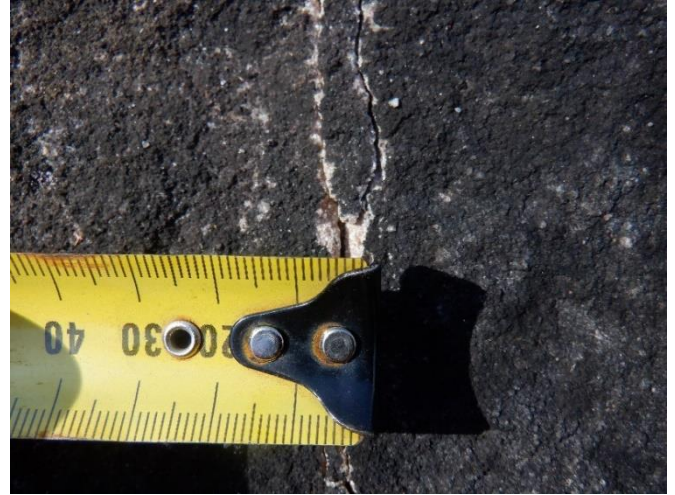
Photo 75: DA3A_LW19_017, width of rock fracturing. Taken on 13/12/2022.
