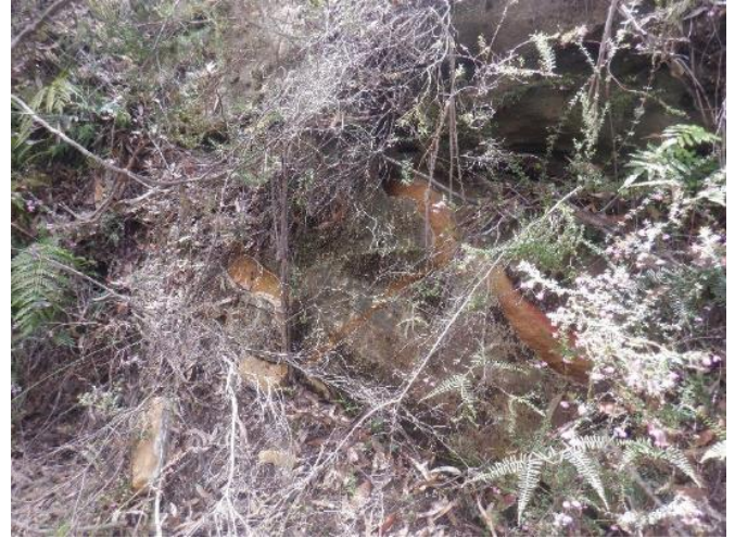
Photo 72: DA3A_LW19_016, section of rock fracturing. Taken on 7/11/2022.
