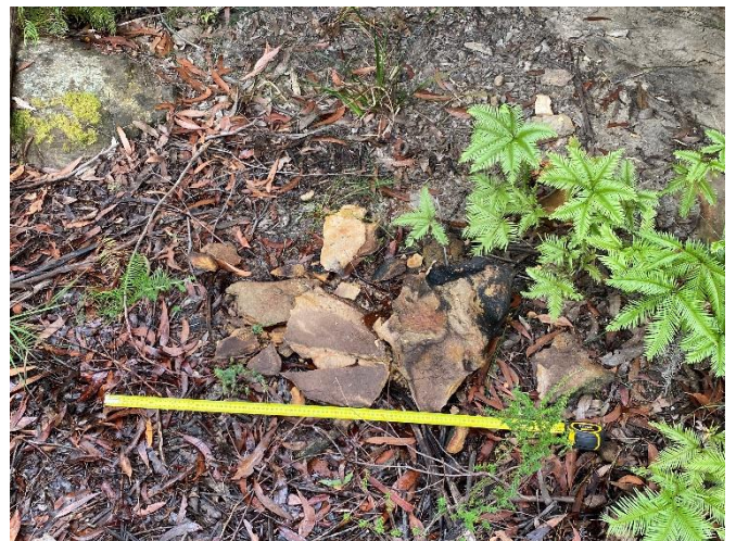
Photo 127: DA3A_LW19_038, rock fall on ground. Taken on 28/03/2023.
