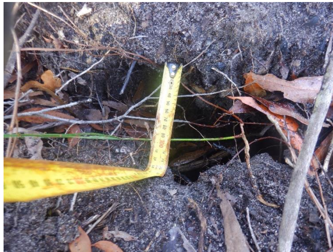
Photo 82: DA3A_LW19_020, showing erosion of soil crack. Taken on 09/05/2023.
