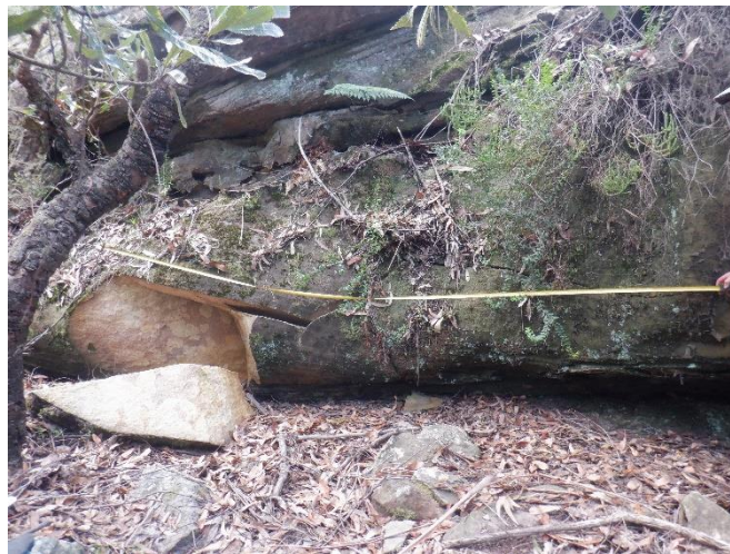
Photo 73: DA3A_LW19_016, showing extent of rock fracturing. Taken on 19/04/2023.
