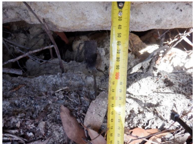
Photo 86: DA3A_LW19_021, width of soil cracking. Taken on 13/12/2022.
