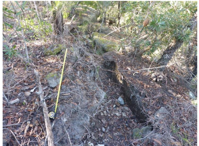
Photo 158: DA3A_LW19_056, showing top view of block that have moved away from the adjacent ground. Taken on 5/05/2023.
