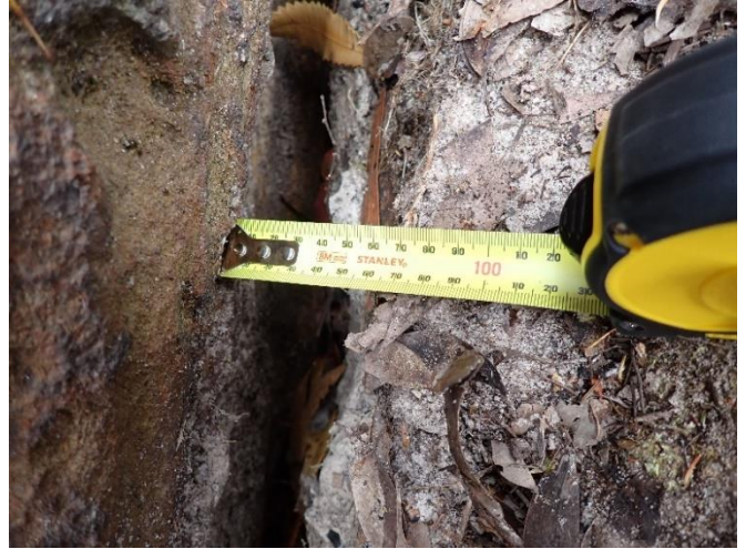
Photo 98: DA3A_LW19_025, width of rock displacement. Taken on 20/12/2022.
