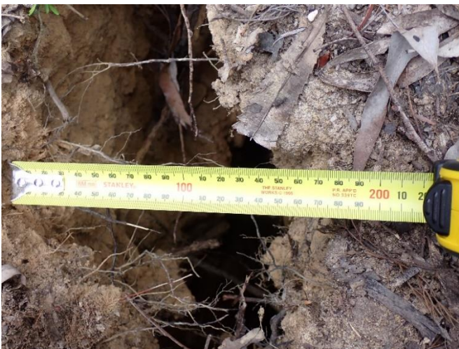
Photo 95: DA3A_LW19_024, width of soil cracking. Taken on 20/12/2022.
