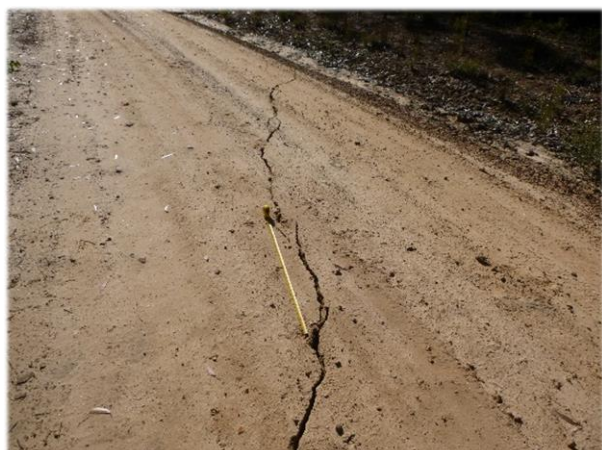
Photo 67: DA3B_LW13_003, showing the longest continuous section of cracking on FR6A, taken 26/06/2017.
