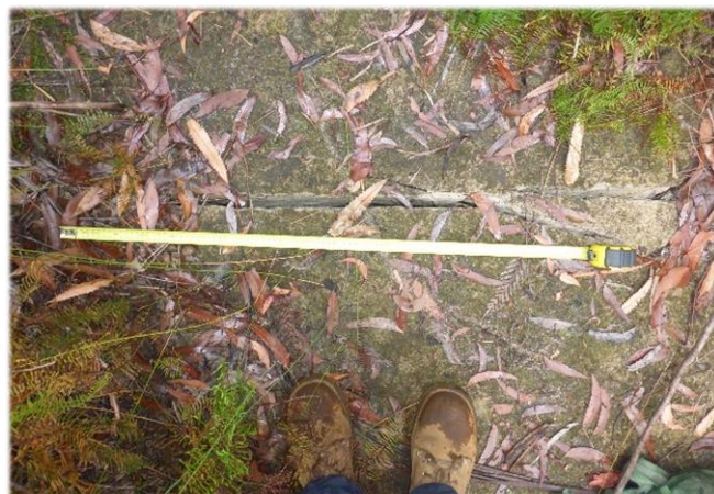
Photo 57: Impact DA3B_LW13_017, overall extent. Taken on 8/01/2018.
