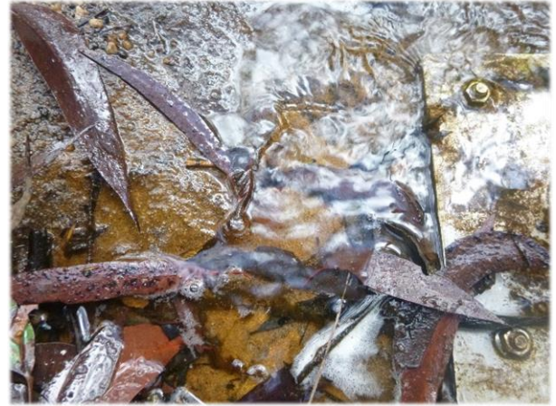
Photo 8: Flow diversion through fracturing in base of pool. Taken on 3/05/2017.
