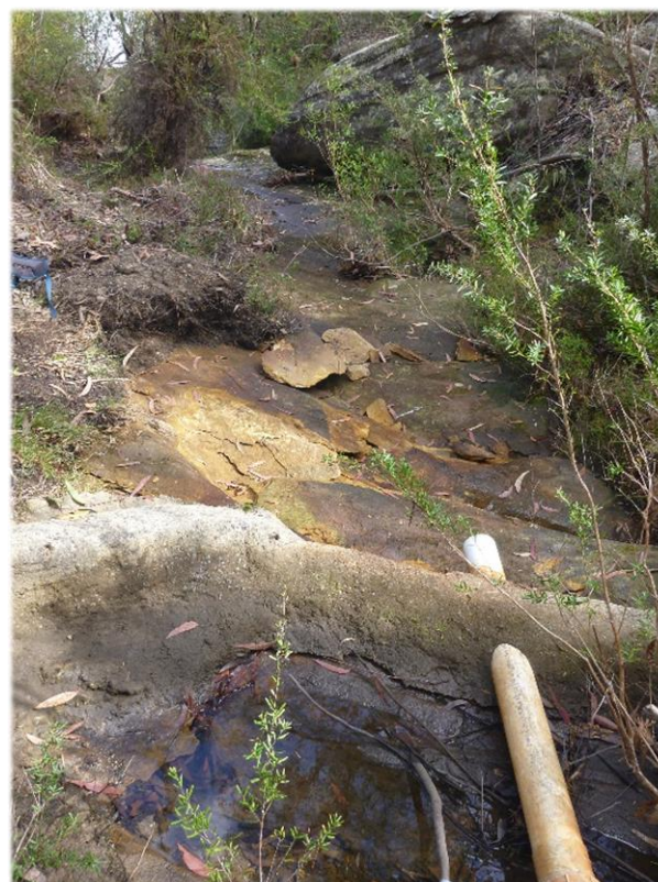
Photo 6: Fracturing downstream from concrete weir, looking downstream. Taken on 19/04/2017.
