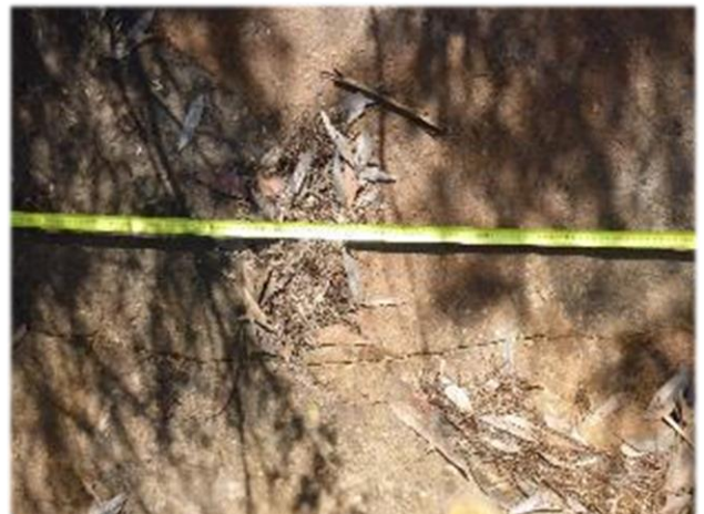
Photo 14: DA3B_LW13_021, looking at the narrowest section of fracturing. Taken 29 th March 2018.
