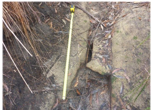
Photo 45: Impact DA3B_LW13_009 , looking upstream, taken on 23/10/2017.
