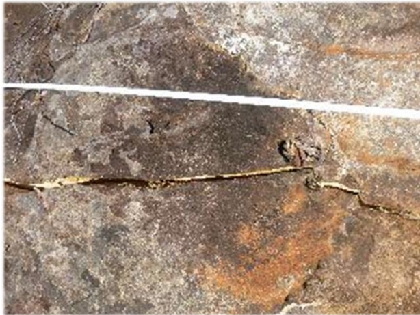
Photo 19: DA3B_LW13_023, widest section of fracturing. Taken 29 th March 2018.
