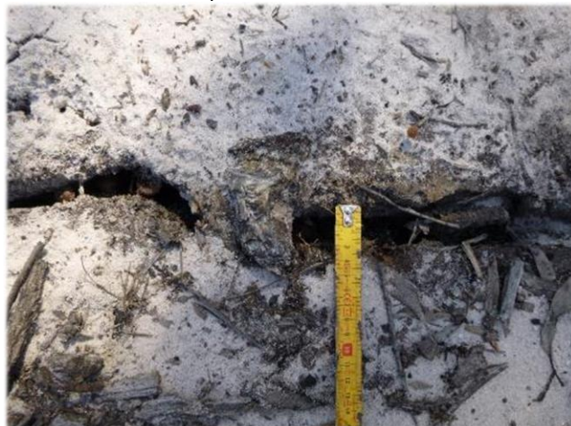
Photo 65: DA3B_LW13_034, close up of the widest section of the soil cracking impact. Taken 9 th April 2018.
