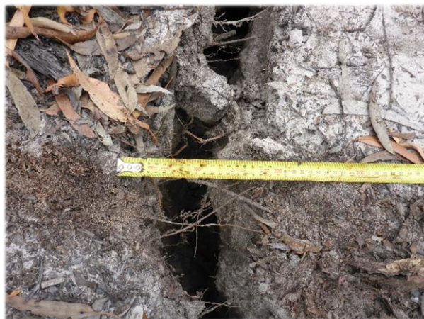
Photo 70: DA3B_LW13_019, looking inside soil crack. Taken on 2/03/2018
