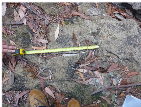
Photo 59: DA3B_LW13_018, looking top-down at the largest fracture. Taken on 12/02/2018.
