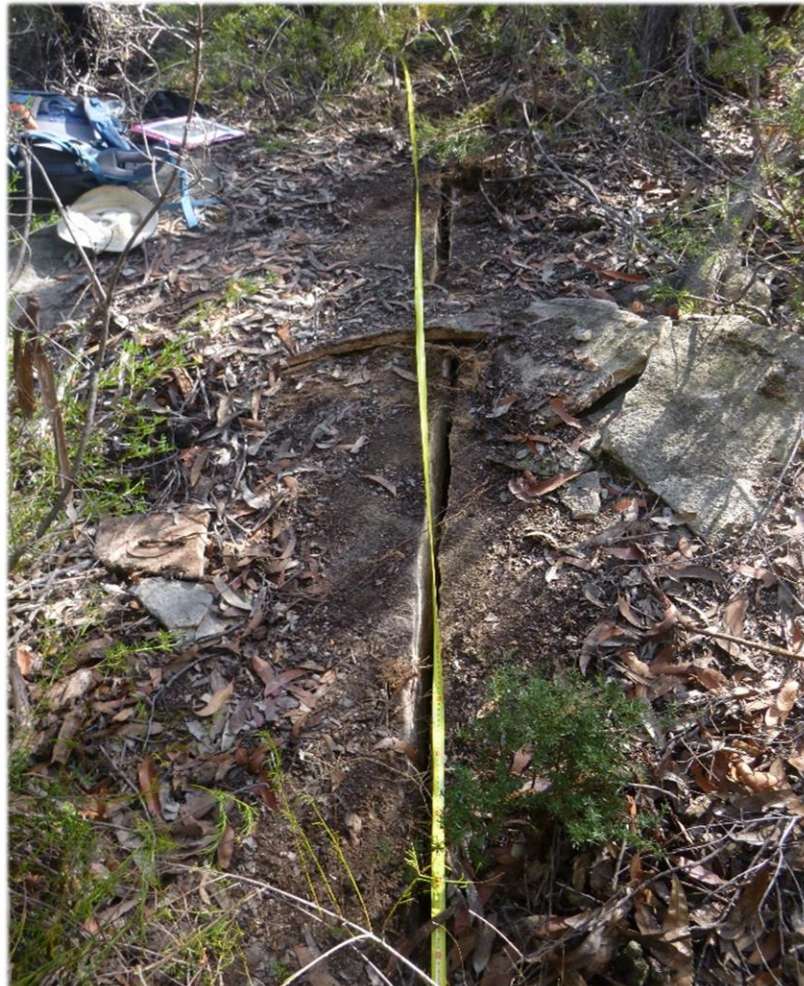
Photo 62: Photo DA3B_LW13_036, looking at the extent of the fracture. Taken 23 rd April 2018
