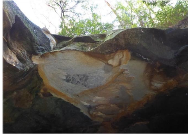
Photo 32: DA3B_LW13_041, looking at the extent of the rockfall. Taken 7 th May 2018
