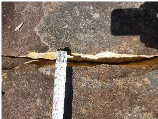
Photo 21: DA3B_LW13_023, closeup of the widest section of fracturing. Taken 29 th March 2018.
