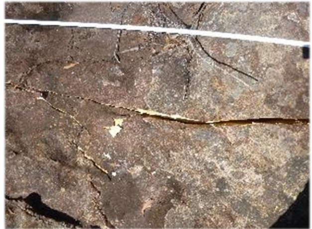
Photo 20: DA3B_LW13_023, widest section of fracturing. Taken 29 th March 2018.
