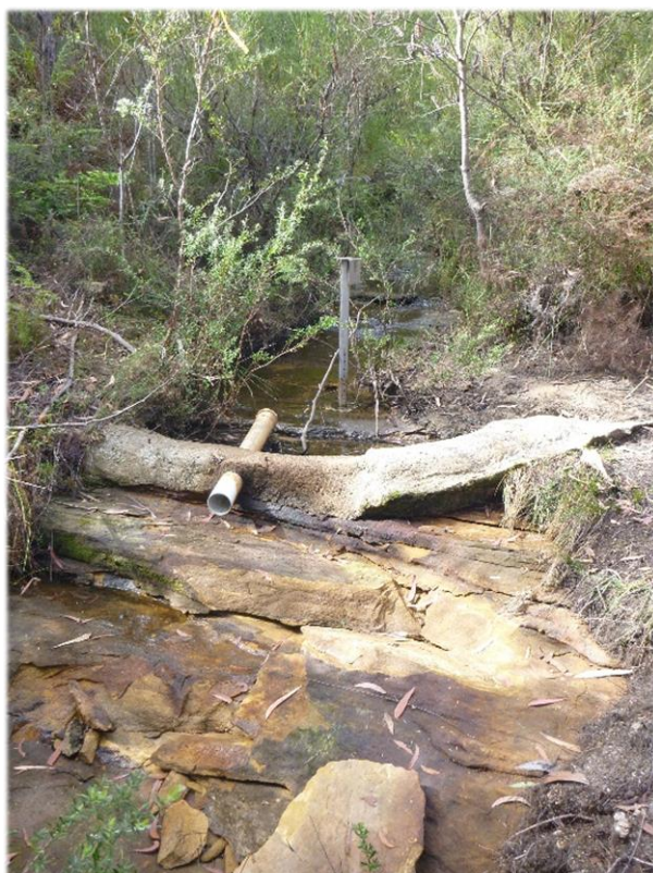
Photo 5: Fracturing downstream from concrete weir, looking upstream. Taken on 19/04/2017.
