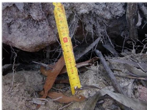
Photo 68: DA3B_LW13_029, close up of the widest section of cracking. Taken 9 th April 2018.
