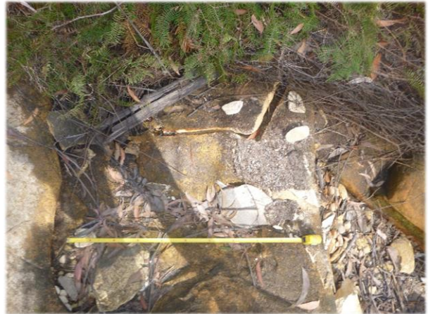
Photo 41: Impact DA3B_LW13_006 , looking across pool at fracturing. Taken on 3/10/2017.
