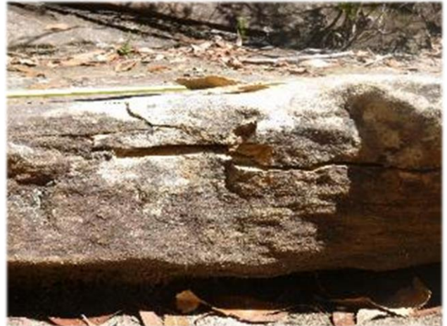
Photo 24: DA3B_LW13_028, looking upstream at largest section of fracturing. Taken 5 th April 2018.
