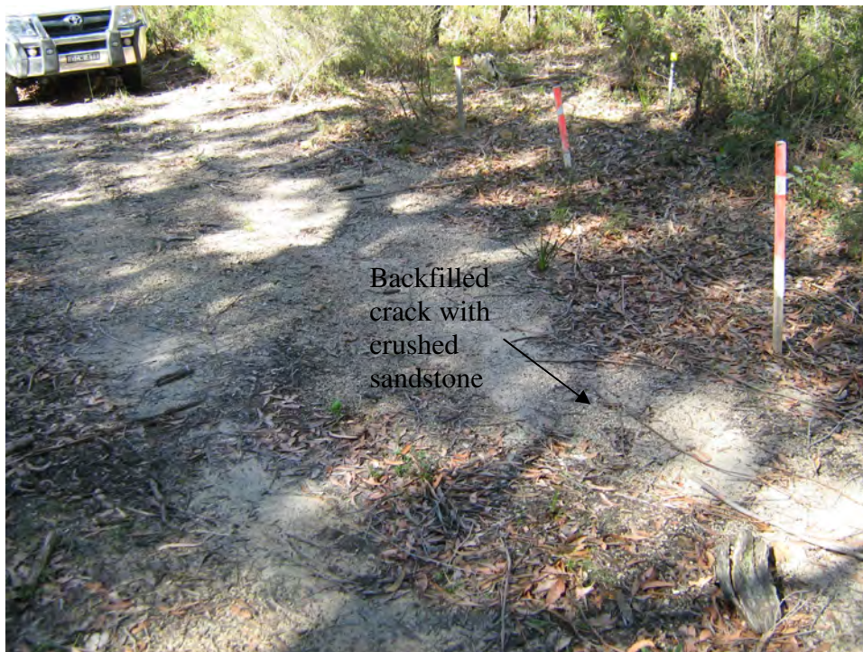
Photo 2 - Remediation Works of 300 mm wide Fire Trail Cracks in Area 1 (2-3 years old)
