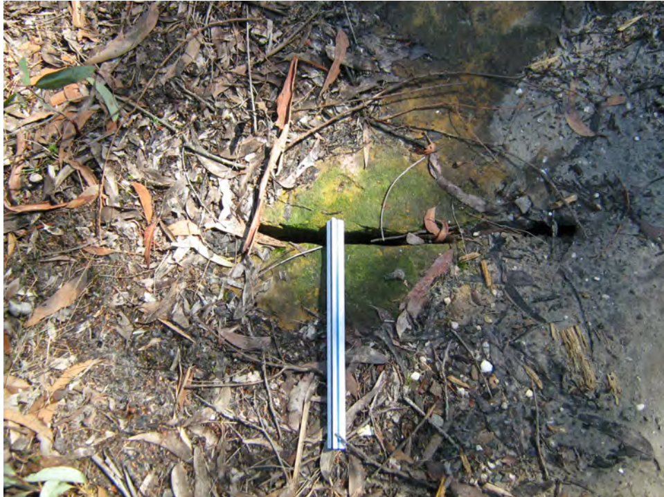
Photo 1 - Remnant Fire Trail Cracks in Area 1 (2 years since mining of LWs 1 and 2)
