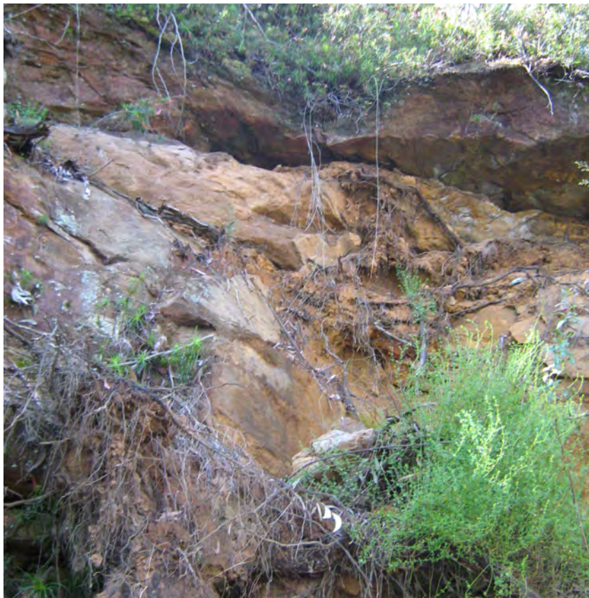
Photo 4 - Area 1 Rock fall Site G (exposed cliff face)
