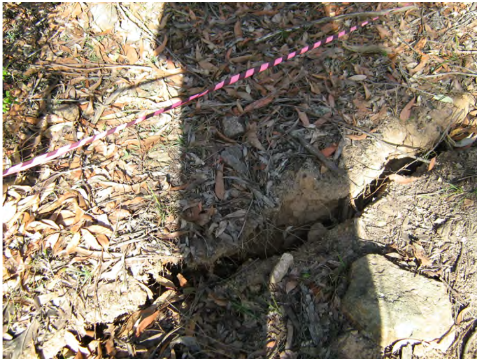
Photo 8 - Area 2 Fire Trail Cracking ( 1 year since mining)
