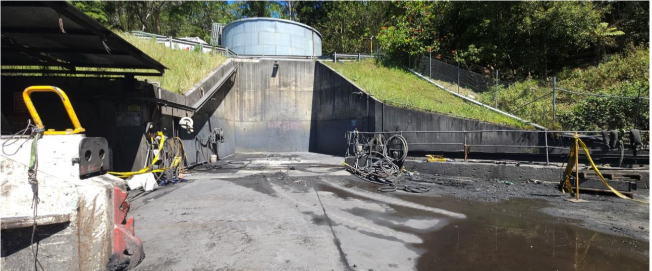
Dendrobium Pit Top – Upper Portal Road, dust suppression spray system in use
