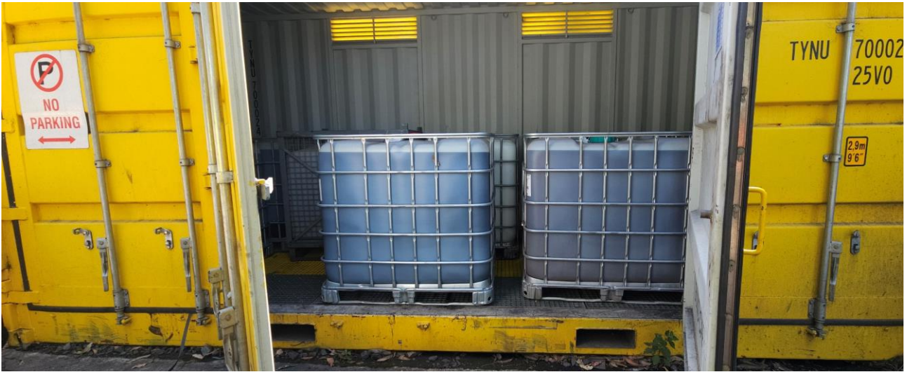
Dendrobium Pit Top – Liquids bunding and spill response station
