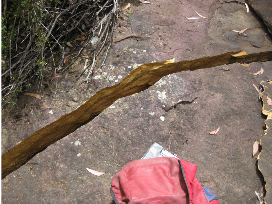
Photo 7 - Tensile (left) and shear cracking (SE) in Area 3A Along WC17
