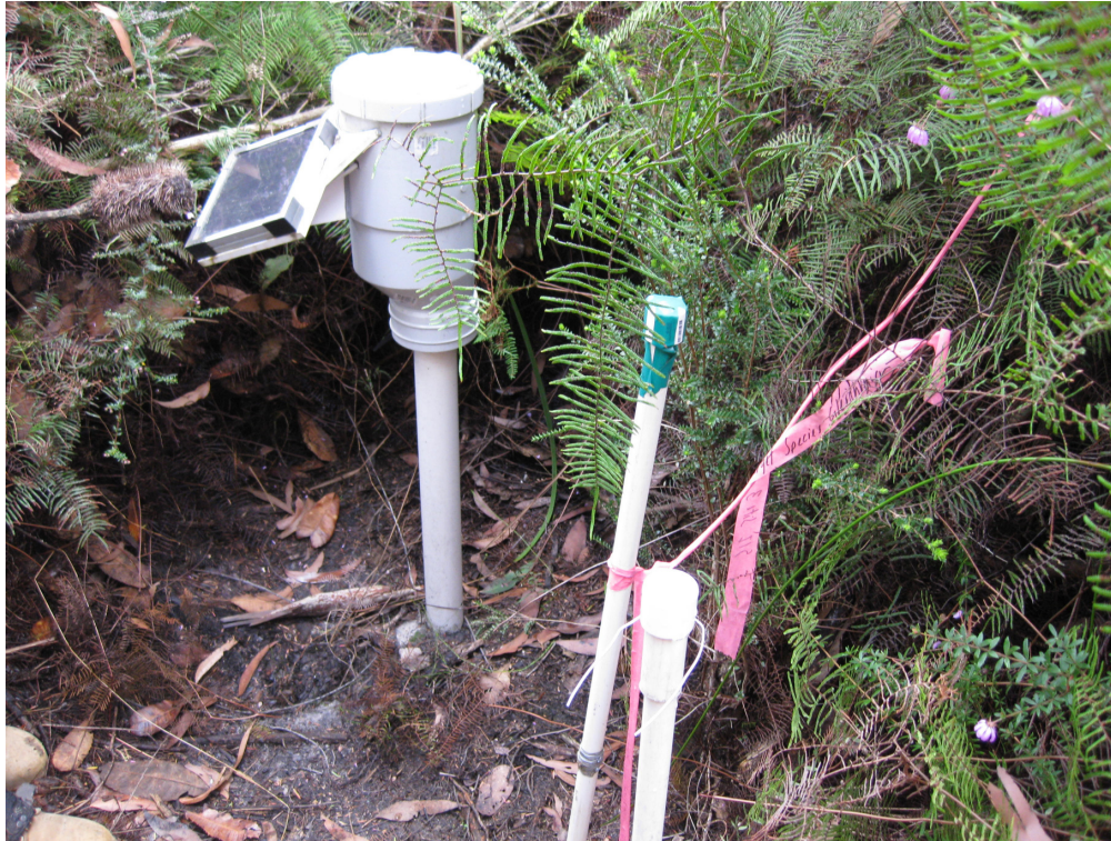
Photo 5 - Swamp 12 Environment Monitoring Cluster of Boreholes in Area 3A
