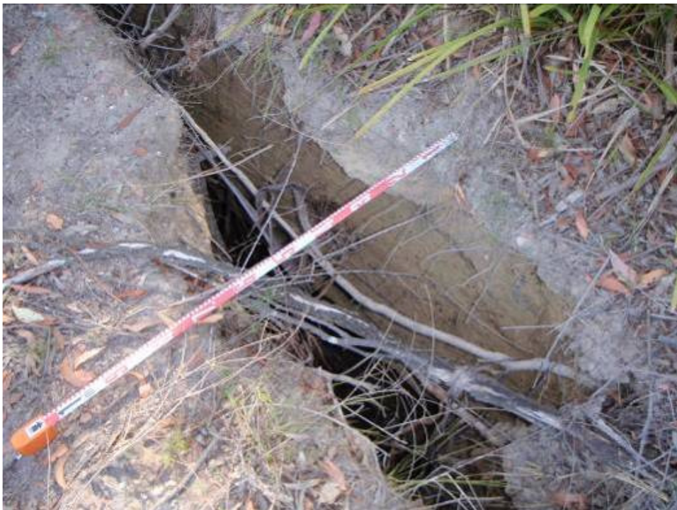
Photo 2 - 500 mm Wide Tension crack on steep slope above Watercourse LW 5 (Photo courtesy of IC Environmental Team dated Dec, 2009)
