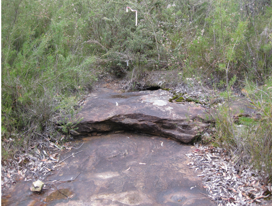
Photo 1 - Down stream Rock Bar (minor cracking) at Swamp 1 in Area 2 (>2 years since mining of LWs 4 and 5)
