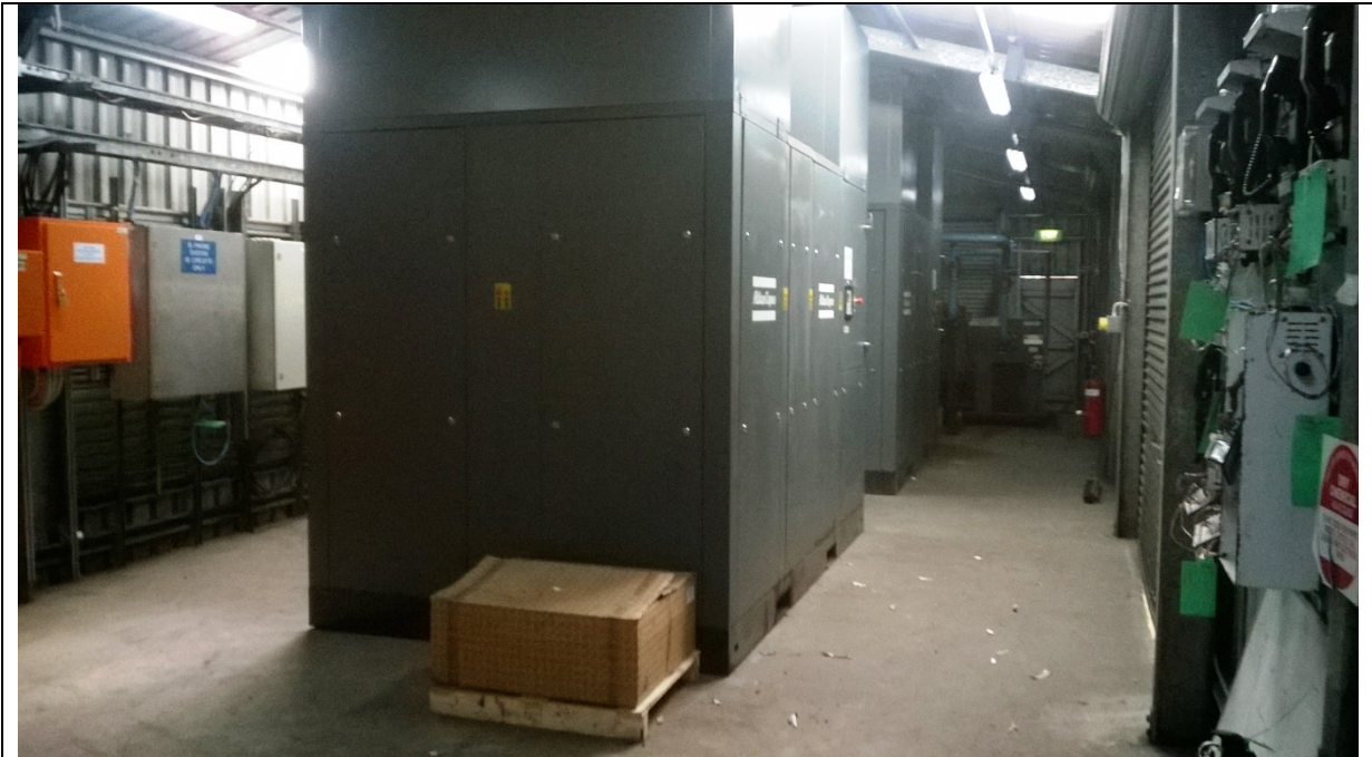
Picture E3: Acoustically treated compressor enclosures (Dendrobium Colliery Surface)
