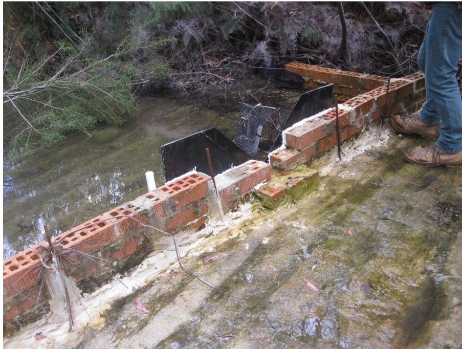
Photo 11 - V-Notch Weir Constructed by OEH Contractors to Independently Measure Surface Water Discharge Variation over a Rock Bar Down Stream of Swamp No. 1b above LW9
