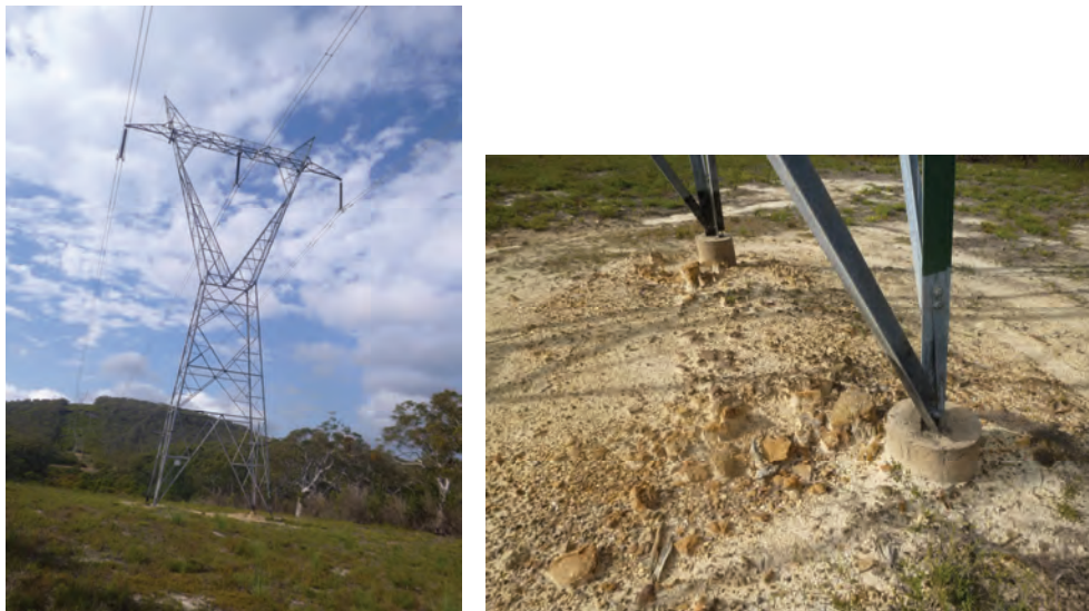
Fig. 6.3 330 kV transmission tower
