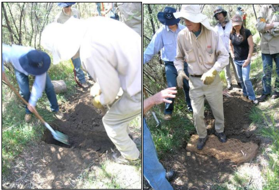
Figure 6-4 Trenching & positioning of the first layer of coir logs and construction of a small dam in an eroding swamp channel
