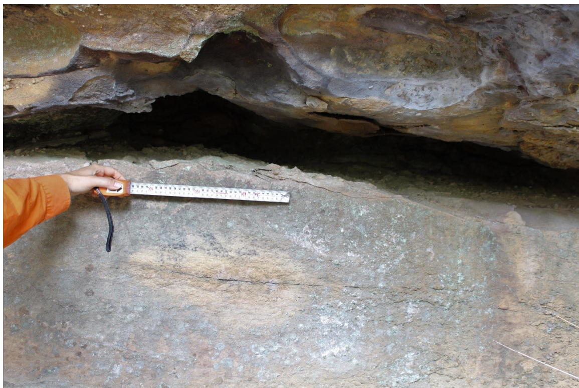
Figure 24: Photograph of cracking above Art Panel 3 motif 1 at Dendrobium 7 (AHIMS ID#52-2-2248).
