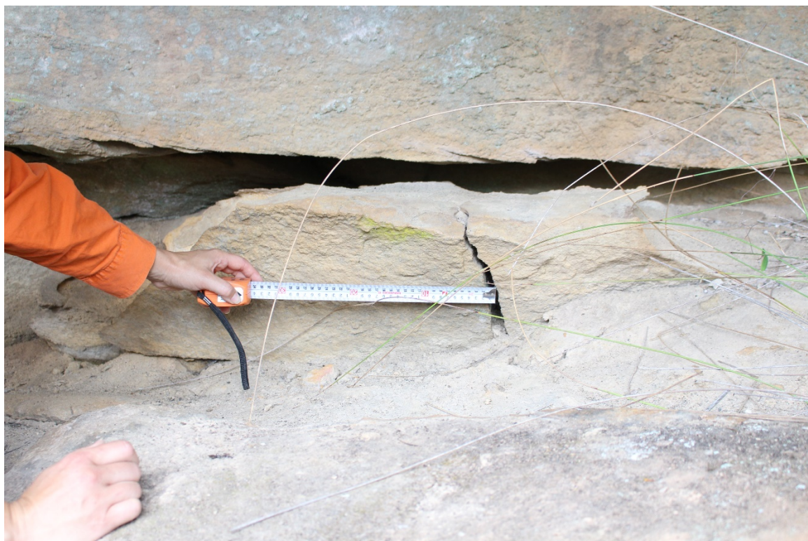
Figure 23: Photograph of vertical cracking at the western end of Dendrobium 7 (AHIMS ID#52-2-2248).
