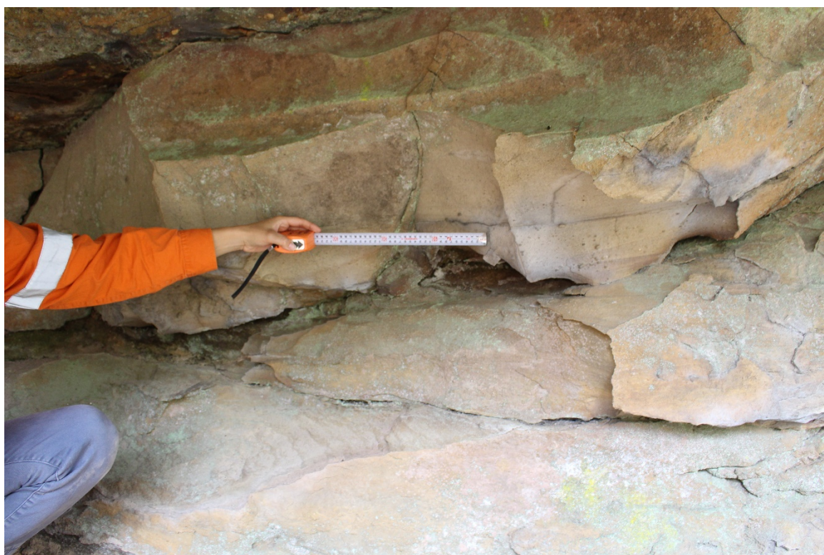
Figure 22: Photograph of cracking and bedding planes at eastern end of the shelter at Dendrobium 7 (AHIMS ID#52-2-2248).
