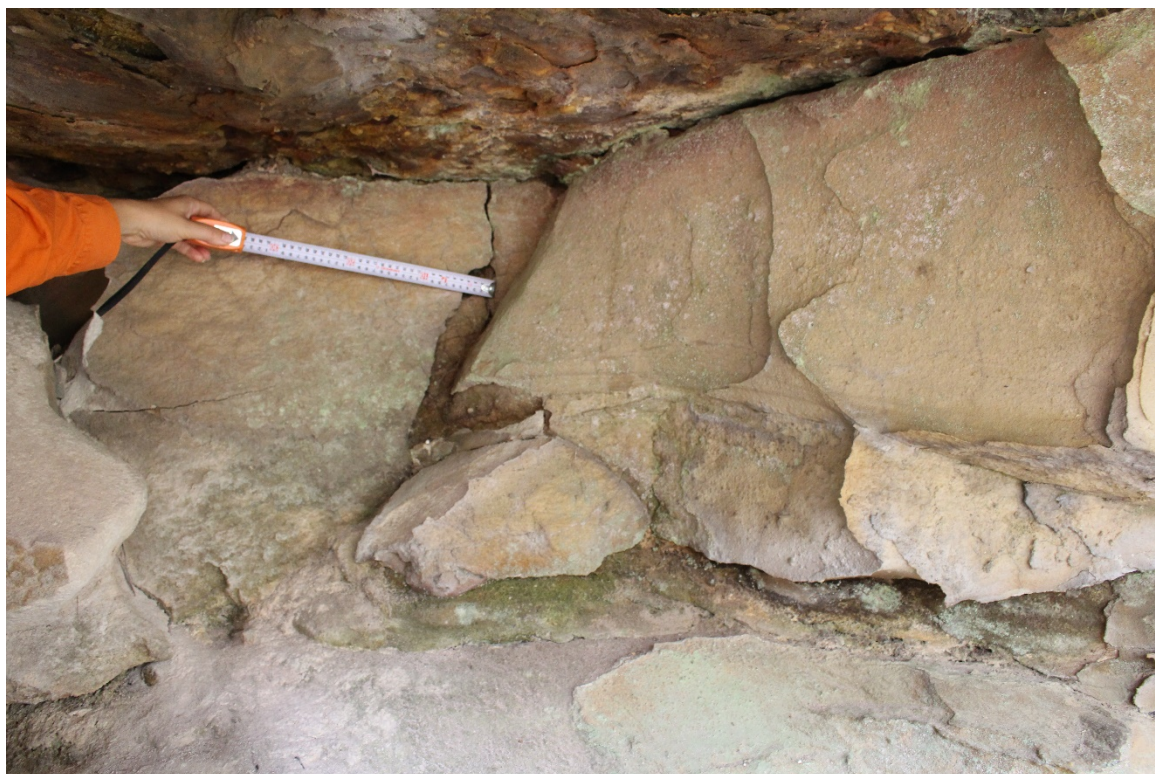
Figure 21: Photograph of natural cracking at western end of the shelter at Dendrobium 7 (AHIMS ID#52-2-2248).
