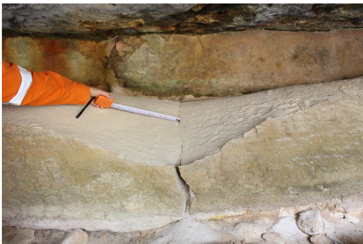
Figure 20: Photograph of crack at the eastern end of the shelter at Dendrobium 7 (AHIMS ID#52-2-2248).
