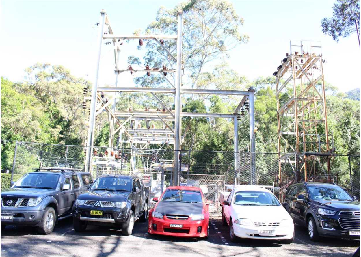
003 View of the 33kV Substation facing west
