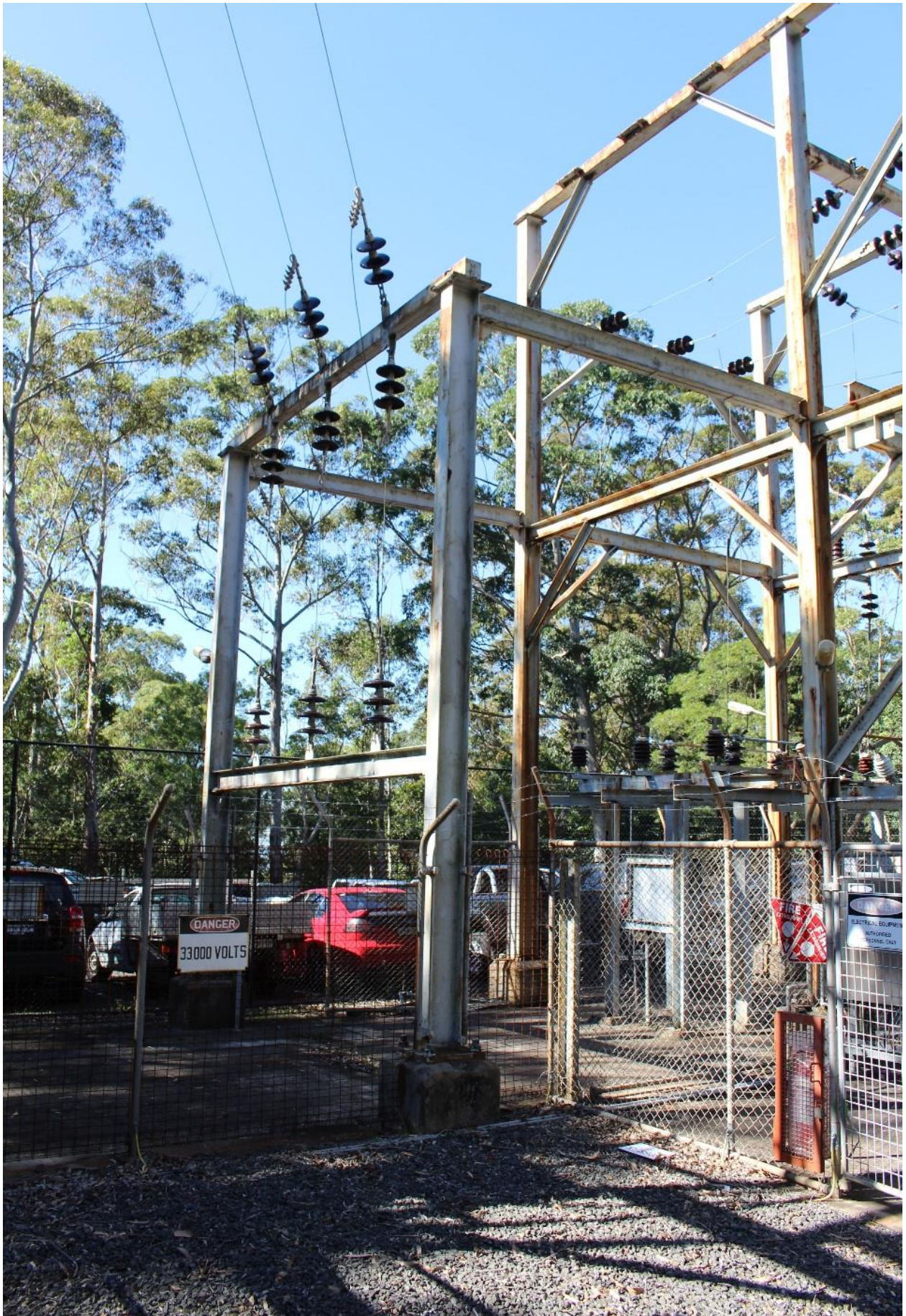
012 View of the eastern side of 33kV Substation looking south east
