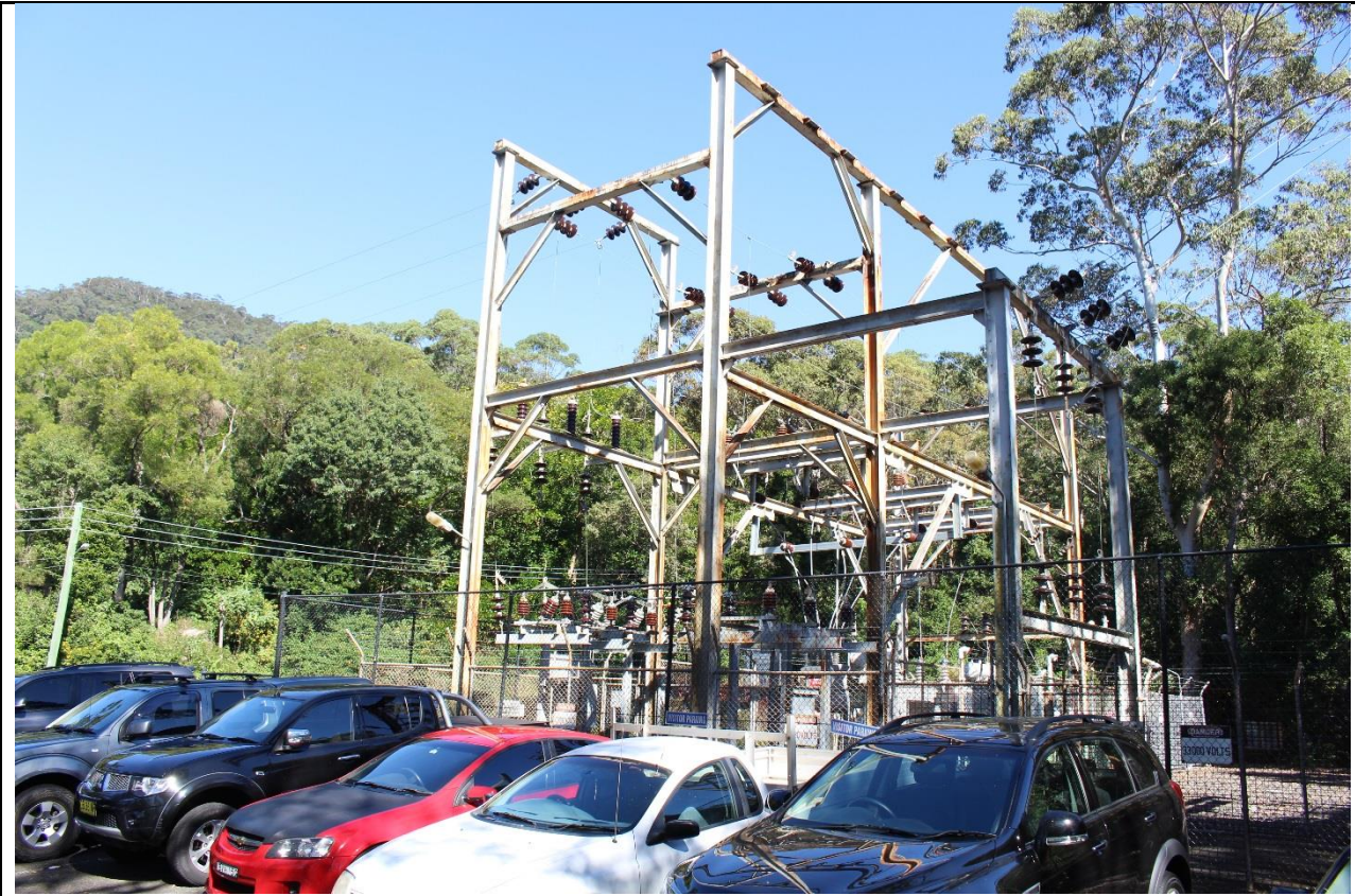
005 View of the 33kV Substation facing north west
