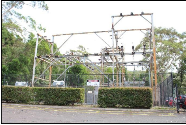
Plate 7: 4 m by 15 m steel tower to the south of the compound, south aspect. (Source: Niche 2018).
