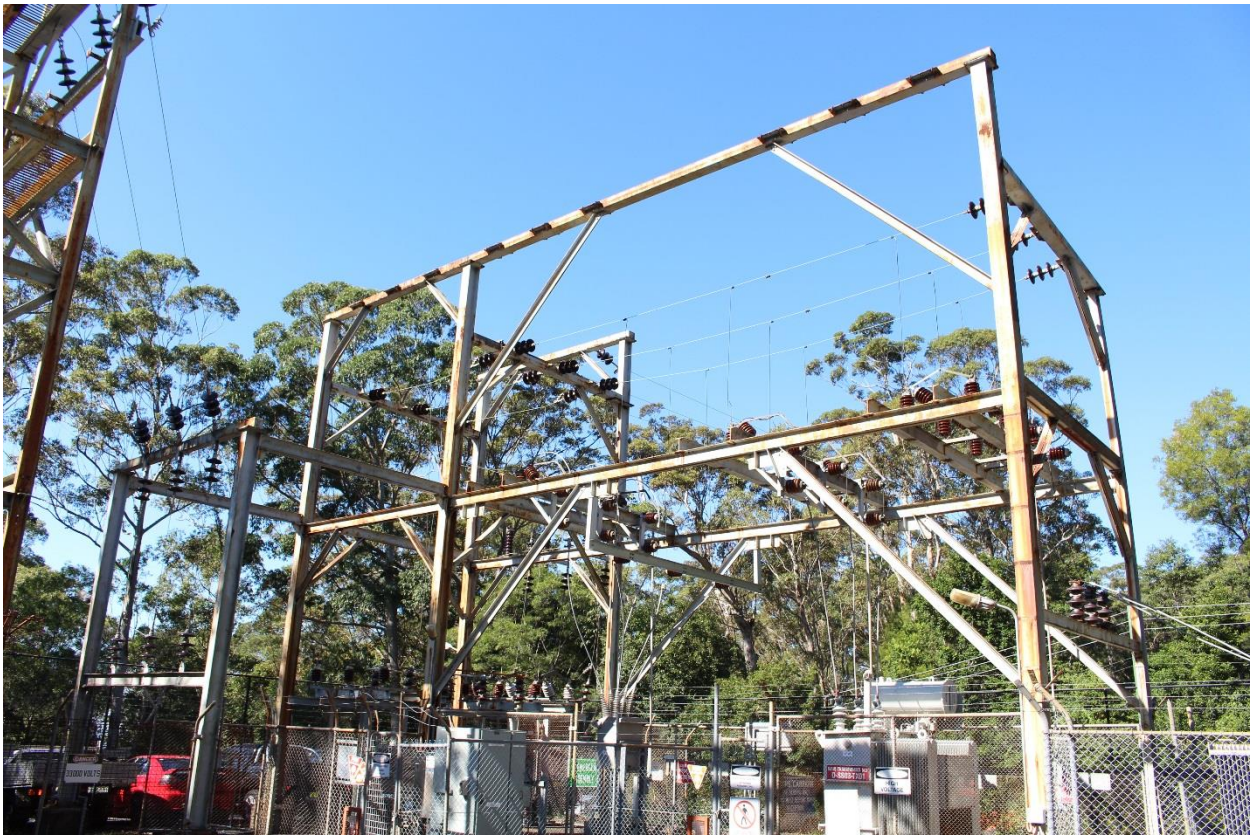
009 View of the 33kV Substation looking south east
