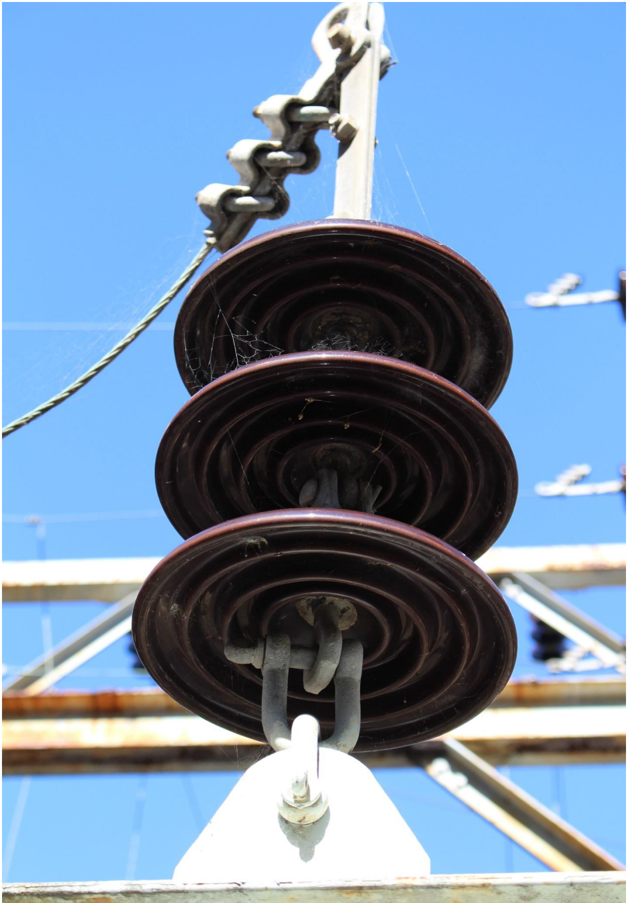
036 View of historical insulators looking south looking south
