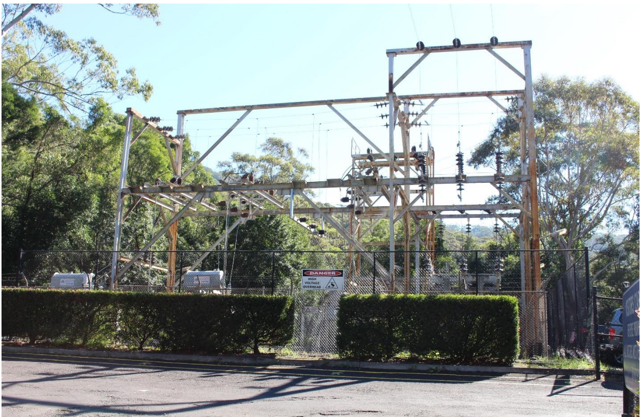
004 View of the 33kV Substation facing north
