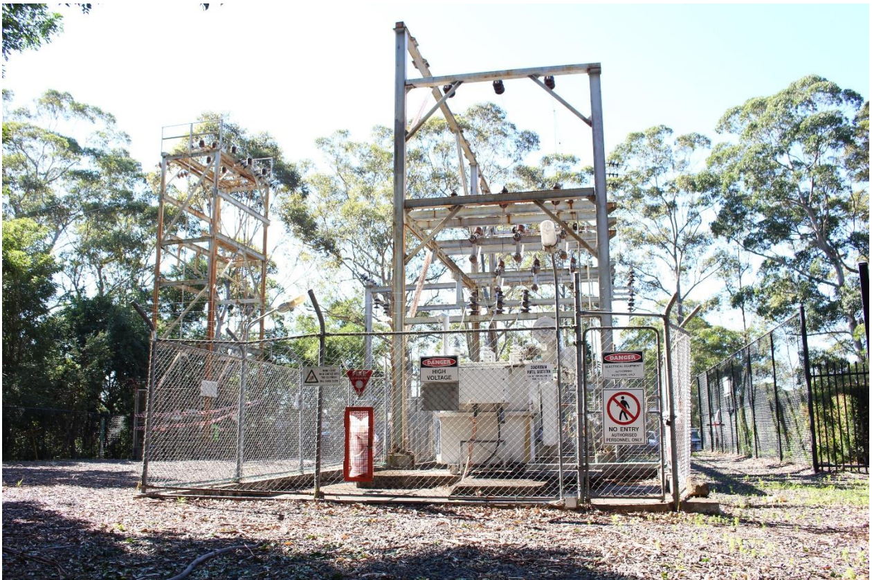
002 View of the 33kV Substation facing north
