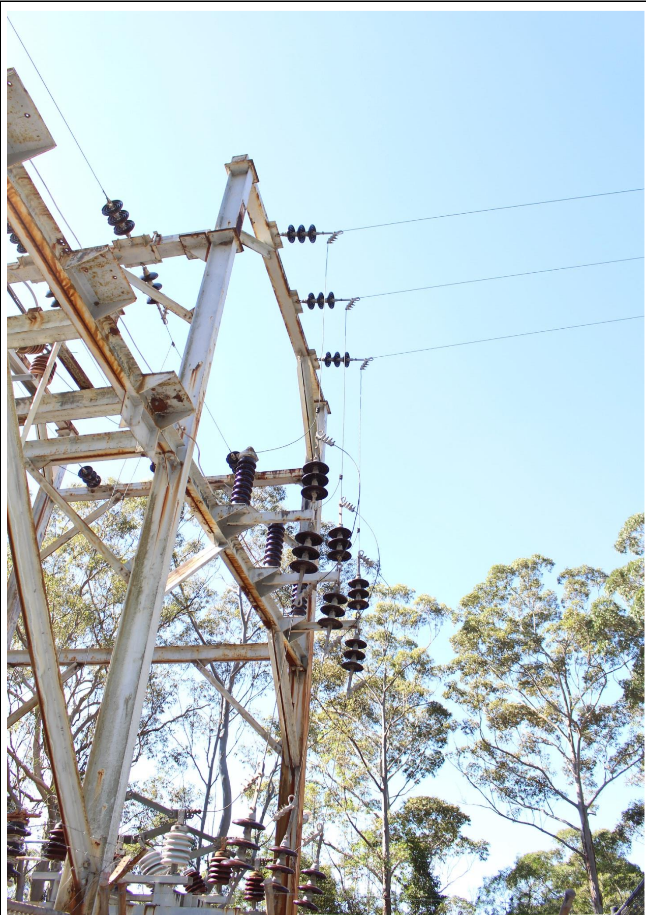
041 View of historical insulators on eastern section 33kV Substation looking north
