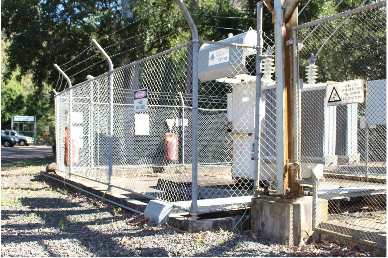
015 View of modern addition to 33kV Substation looking west
