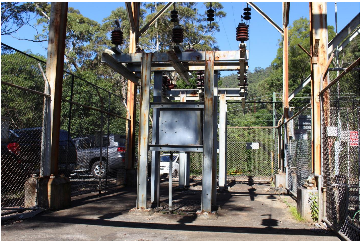
035 View of modern electrical distribution box looking south
