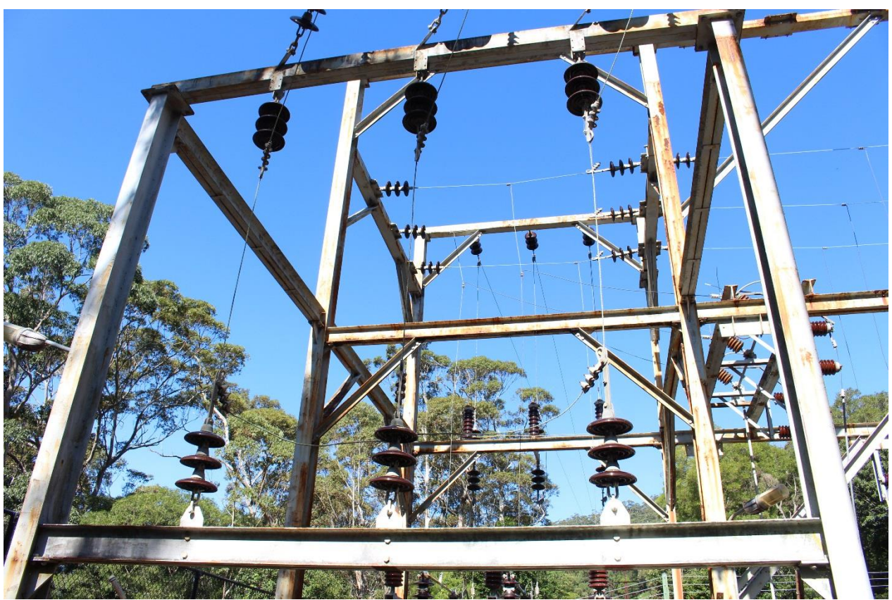
032 View of various historical insulators looking north
