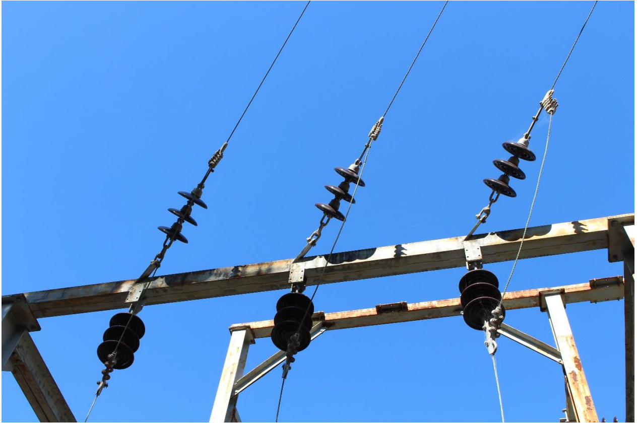
034 View of various historical insulators looking south
