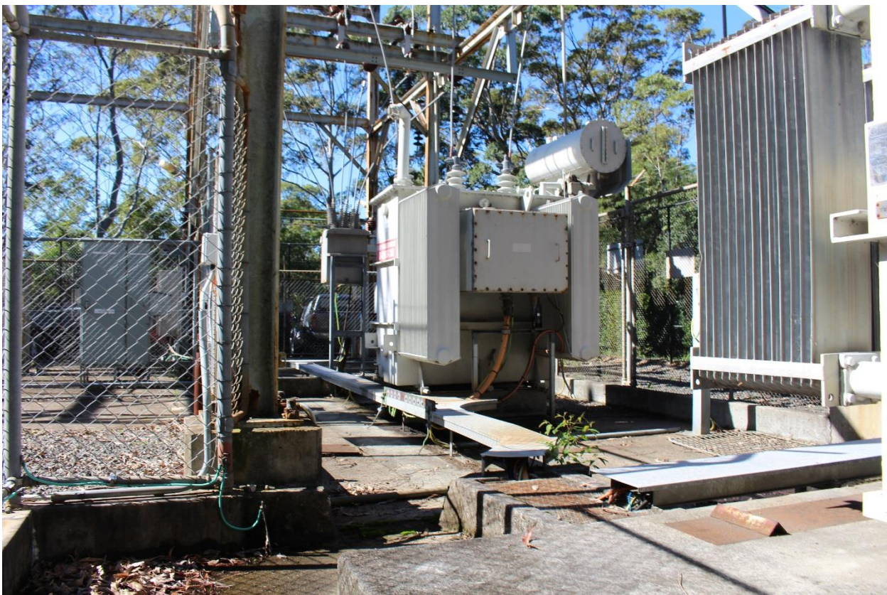
019 View of modern 33/6.6kV 1.5MVA power transformer (D-SS03-TX02) looking east south east
