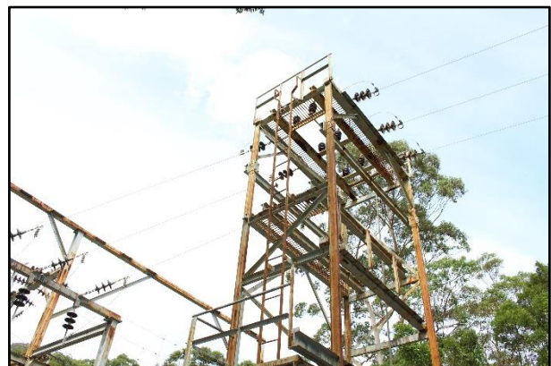
Plate 6: Overhead power cables and orange brown ceramic transmission insulators, south east aspect. (Source: Niche 2018).
