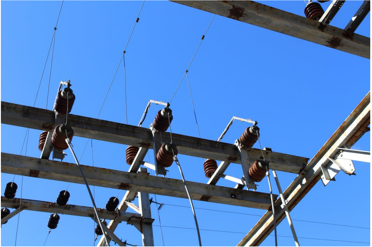
022 View of historic insulators connected to modern transformer looking south east
