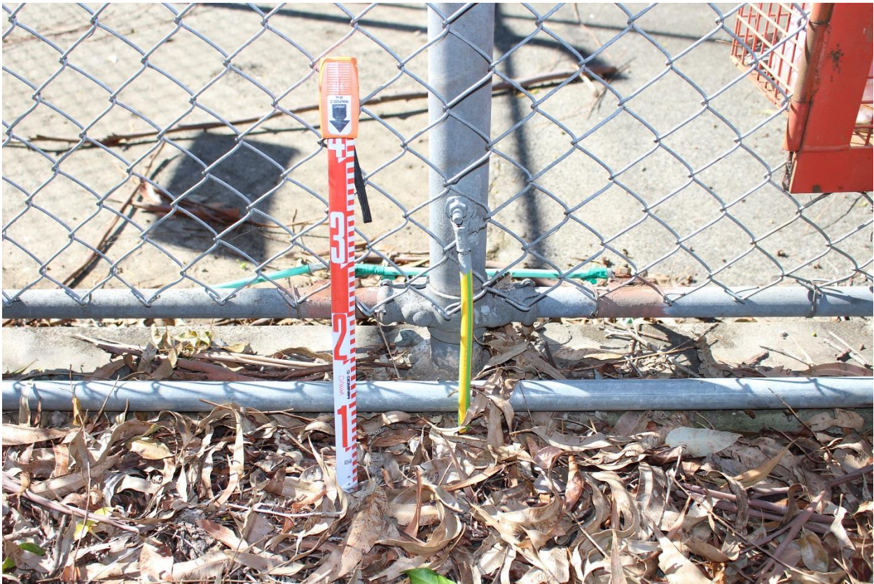
013 View of modern electrical addition to the substation looking south
