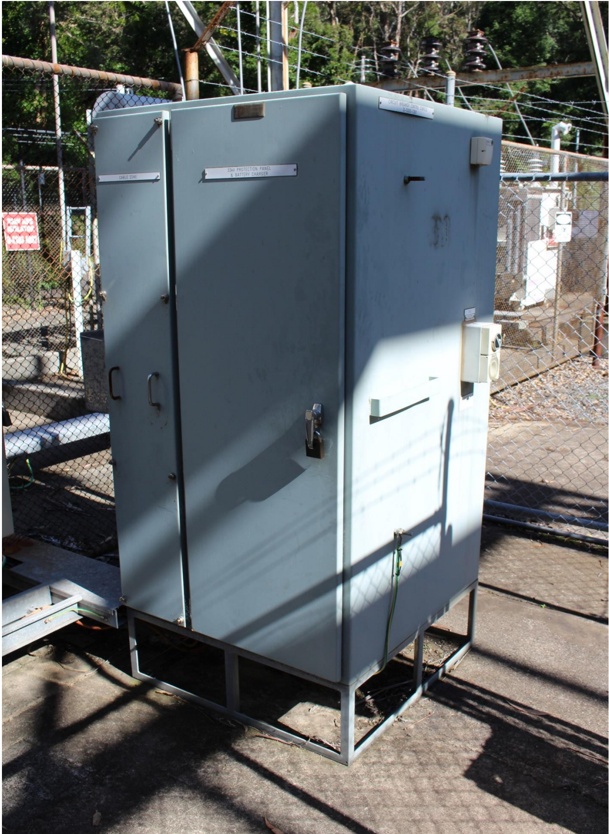
029 View of modern circuit breaker control cubicle (0-SS03-CB01) looking north east
