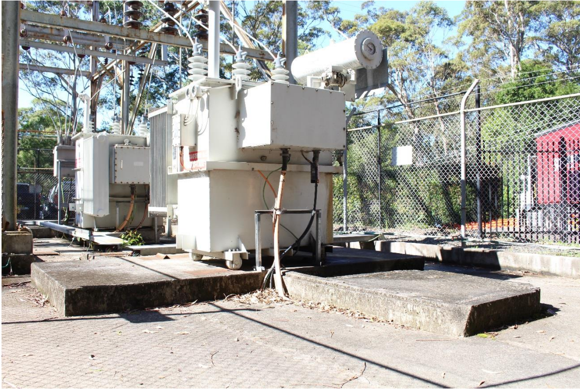
018 View of modern 33/6.6kV 1.5MVA power transformer (D-SS03-TX01) looking east south east
