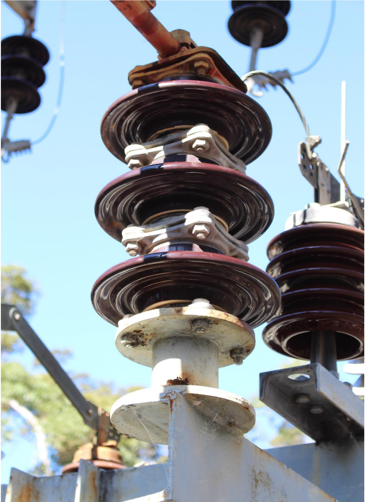
039 View of historical insulators looking south east
