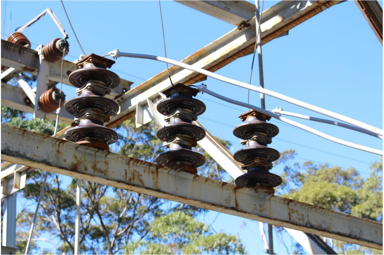
020 View of historic insulators connected to modern transformer looking east
