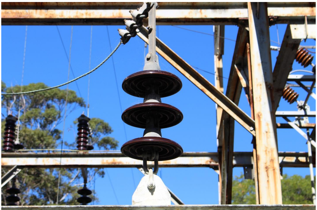
033 View of historical insulator looking north
