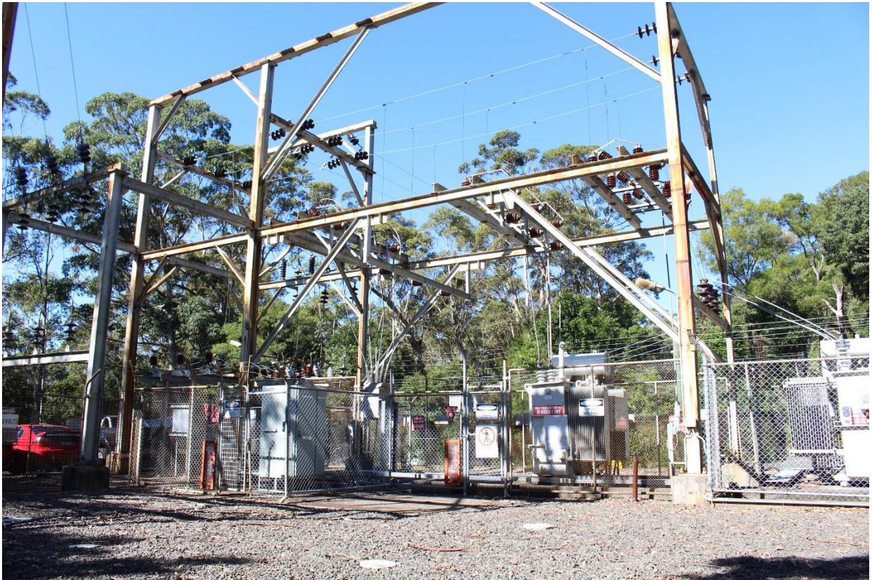
011 View of the 33kV Substation looking south east
