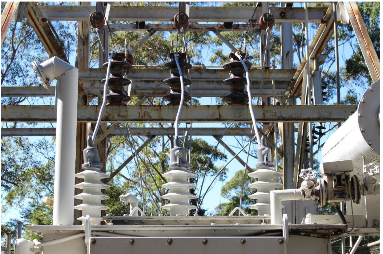
021 View of historic insulators connected to modern insulators looking east
