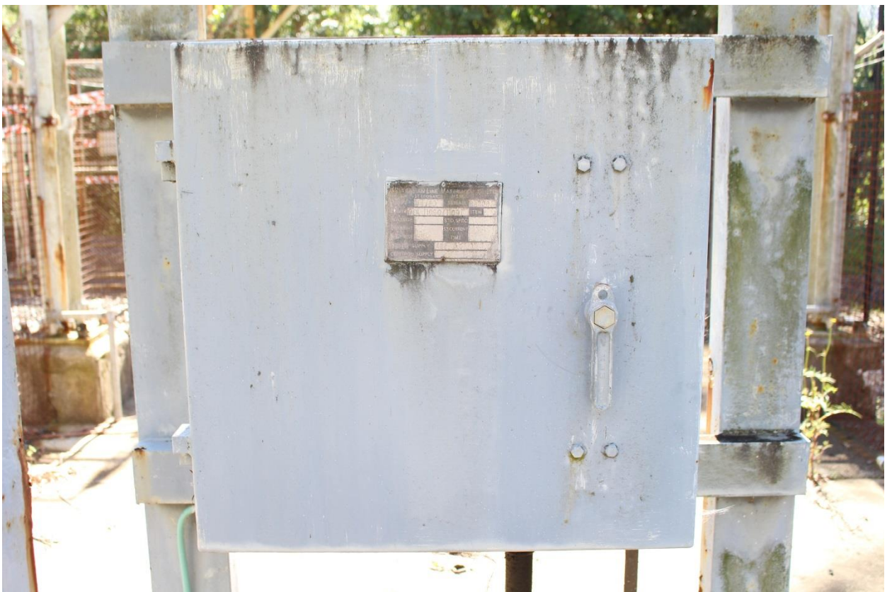
031 View of electrical box looking south
