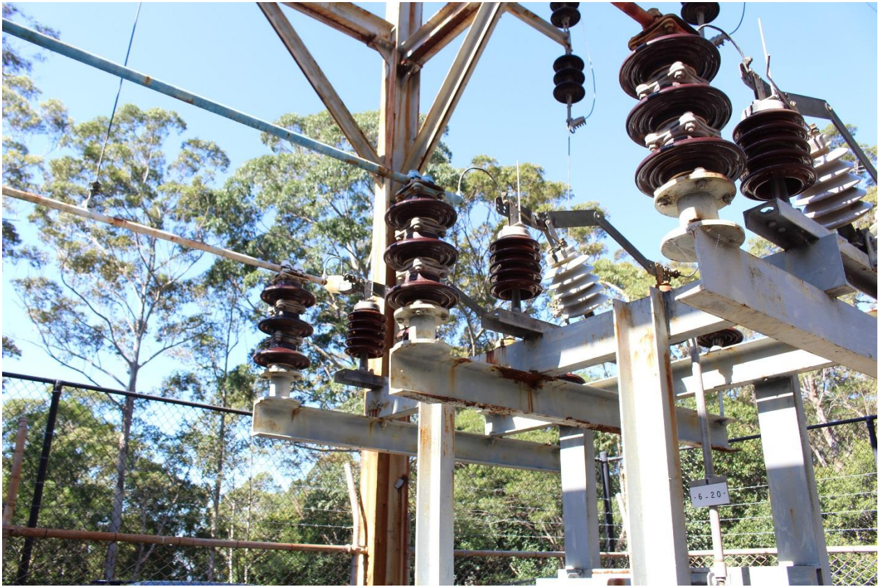
038 View of various historical insulators looking south east
