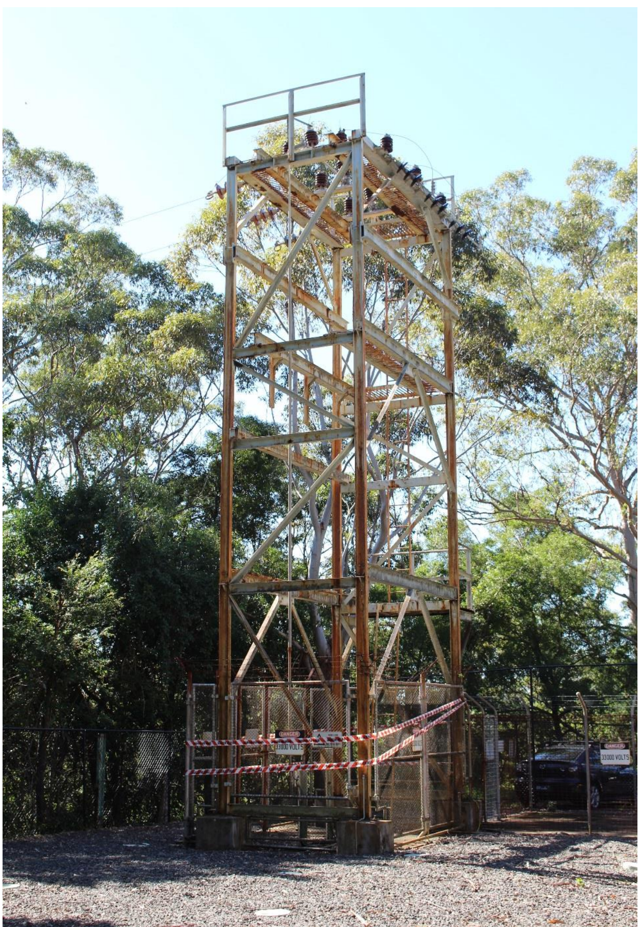
017 View of northern tower of 33kV Substation looking north east
