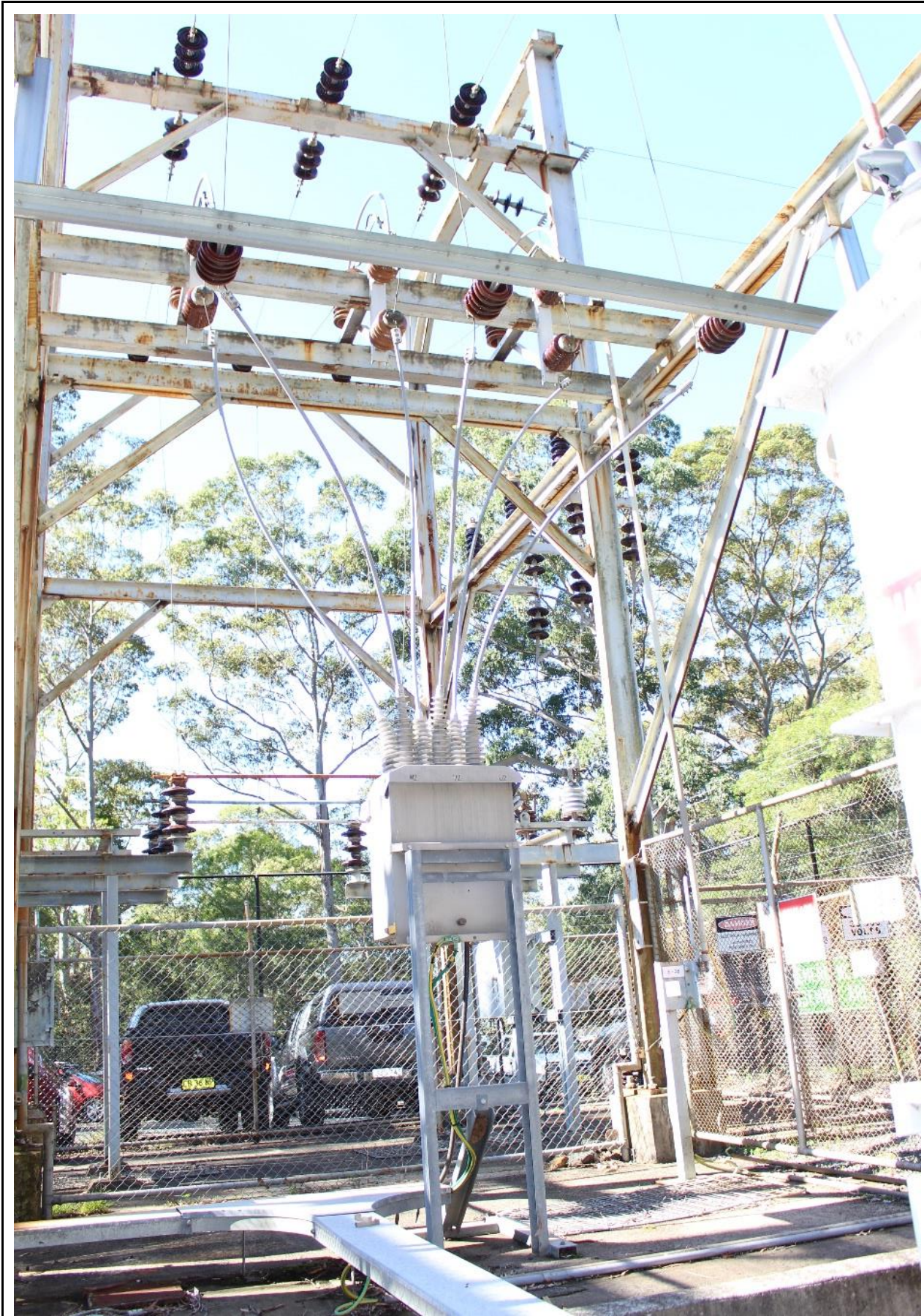
023 View of modern addition to 33kV Substation looking east
