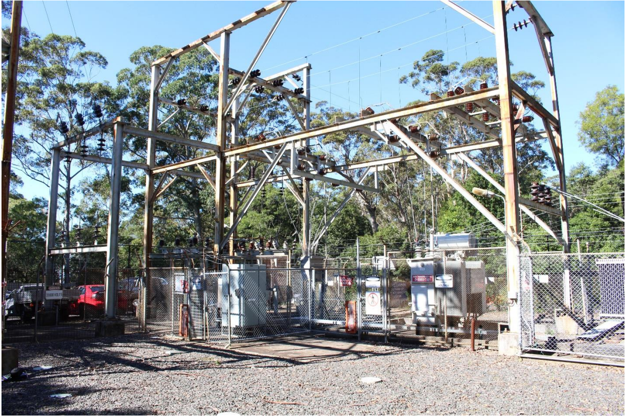
008 View of the 33kV Substation looking south east
