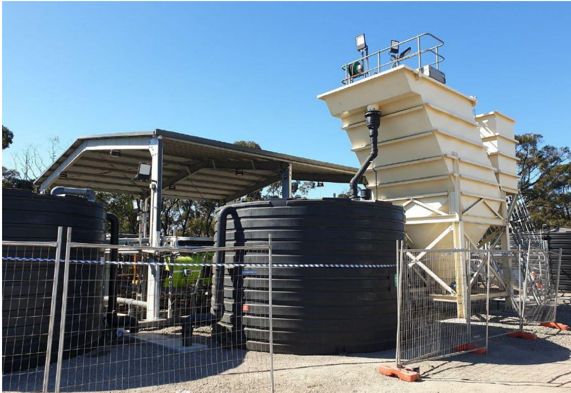
Plate 6: Appin North Temporary WTP
