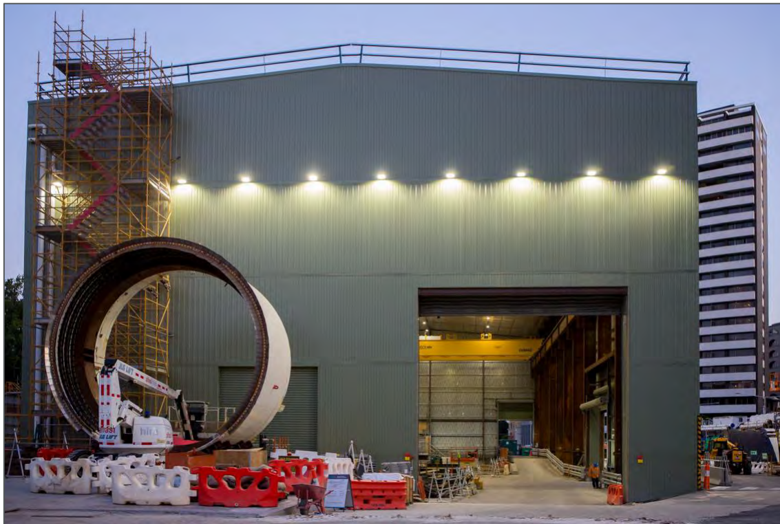
Figure 3-13 Acoustic shed example (external view)
