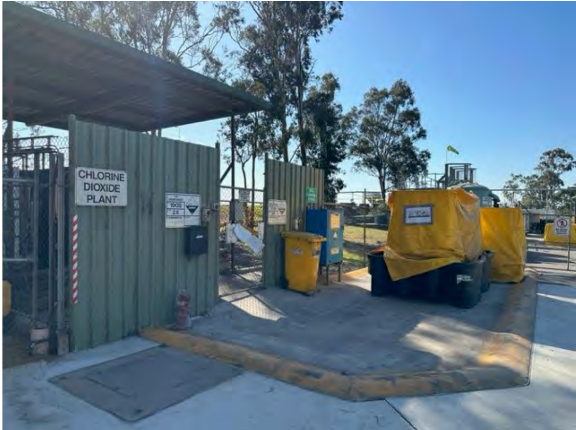
Plate 4: AW WTP Chlorine dioxide refilling bund
