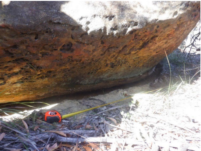
Photo 17: DA3C_LW21_010, Overview of the rock movement/displacement. Taken on 19/06/2023.
