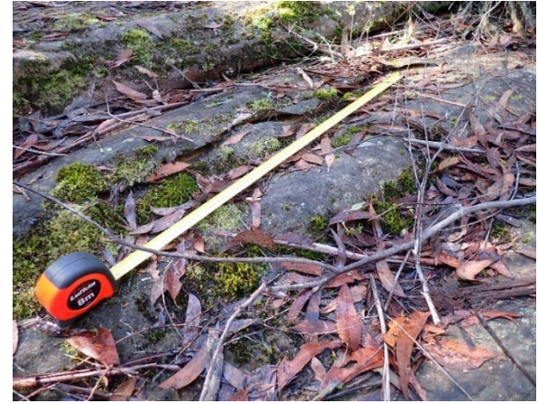
Photo 5: DA3C_LW21_017 , section of rock fracturing. Taken on 26/07/2023.
