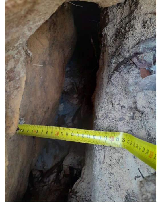
Photo 37: DA3C_LW21_034 , width of soil crack. Taken 12/09/2023.
