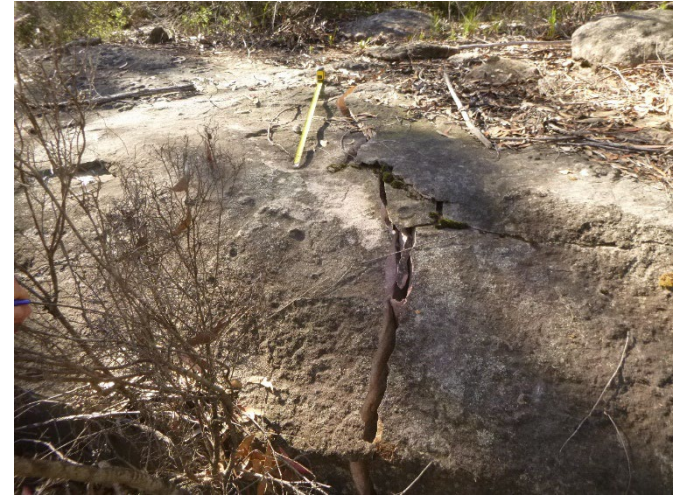
Photo 13: DA3C_LW21_006 , fracturing to rock outcrop. Taken on 15/06/2023.
