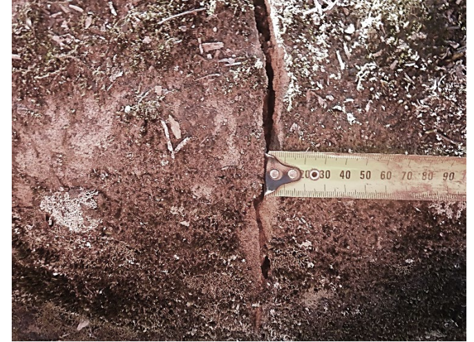
Photo 16: DA3C_LW21_009, maximum width of the rock fracture. Taken on 19/06/2023.
