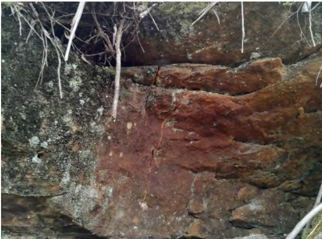
Photo 5: DA3C_LW21_032, overview of fracturing to rock step/overhang. Taken 12/09/2023.
