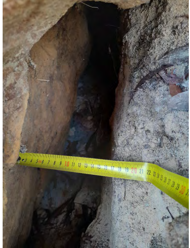
Photo 10: DA3C_LW21_034 width of soil crack. Taken 12/09/2023.
