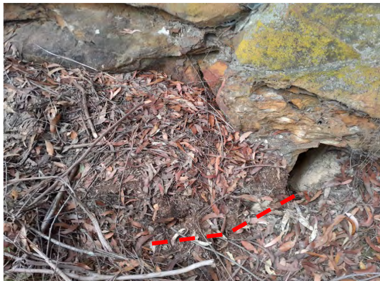
Photo 11: DA3C_LW21_034. Dashed line shows approximate section of unstable soil/leaf litter extending from rock movement. Taken 12/09/2023
