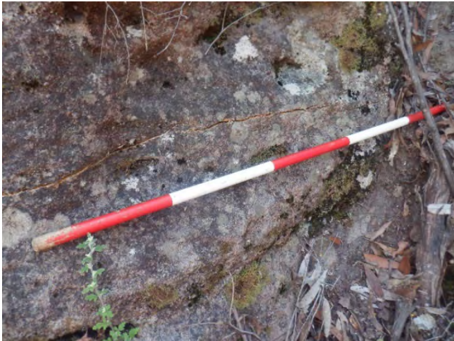
Photo 10: DA3C_LW21_028, rock fracture. Taken 06/09/2023
