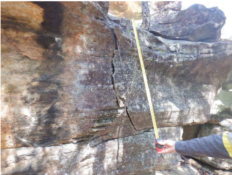
Photo 1: DA3C_LW21_019, looking at the rock fracture. Taken on 1/08/2023.
