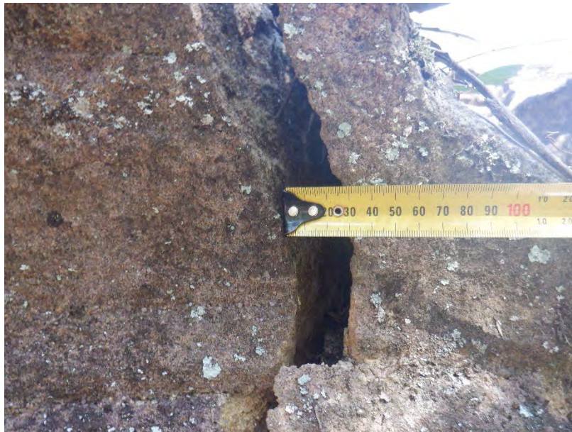
Photo 3: DA3C_LW21_019 , looking at the width of the rock fracture. Taken on 1/08/2023.
