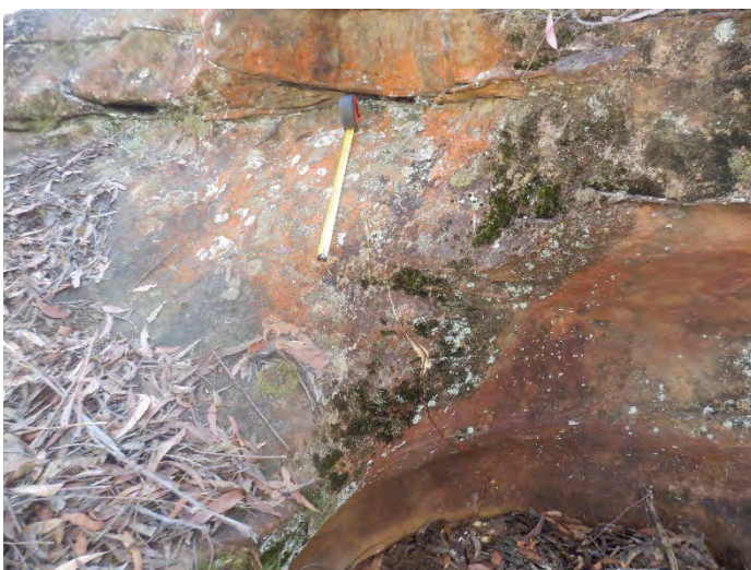
Photo 8: DA3C_LW21_018, section of rock fracturing. Taken on 26/07/2023.
