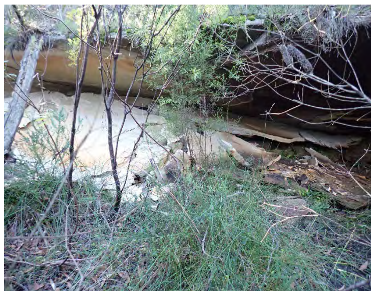
Photo 2: DA3C_LW21_016 , looking at the rockfall. Taken on 26/07/2023.
