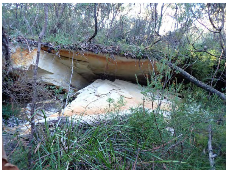
Photo 1: DA3C_LW21_016 , looking at the rockfall. Taken on 26/07/2023.
