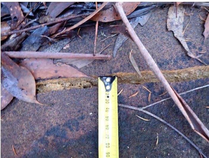
Photo 5: DA3C_LW21_017 , width of the rock fracture. Taken on 26/07/2023.
