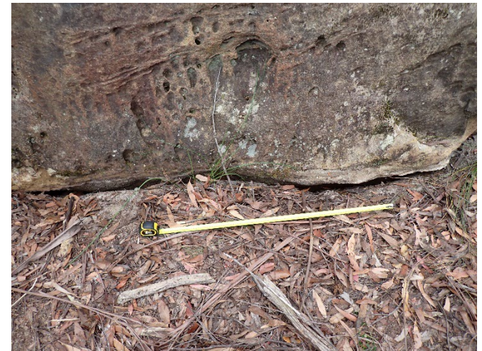
Photo 30: DA3A_LW19_025, showing rock fracturing. Taken on 20/12/2022.
