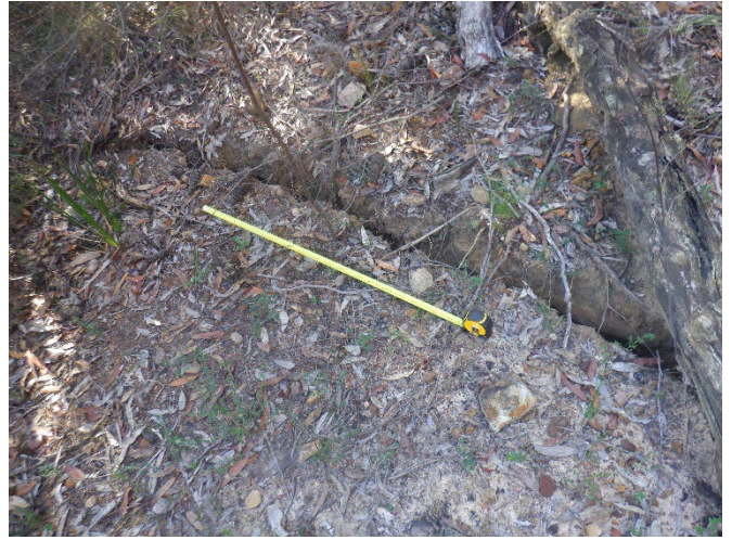
Photo 67: DA3A_LW19_050, showing soil cracking on a closed vehicle access track. Taken on 27/04/2023.
