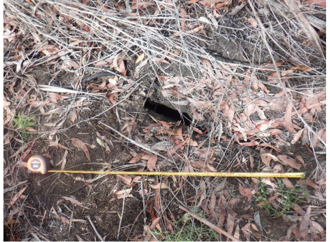
Photo 63: DA3A_LW19_036, showing soil cracking on a closed vehicle access track. Taken on 21/03/2023.
