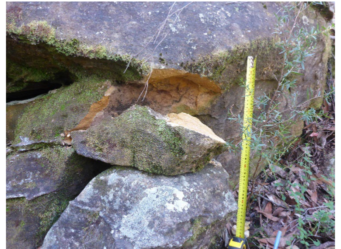
Photo 51: DA3A_LW19_058, showing rockfall. Tape measure set at 0.5m. Taken on 05/05/2023.
