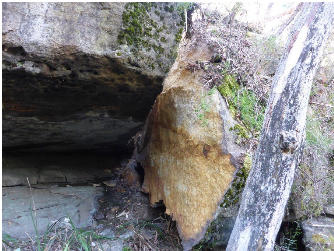
Photo 49: DA3A_LW19_056, showing rockfall. Taken on 05/05/2023.
