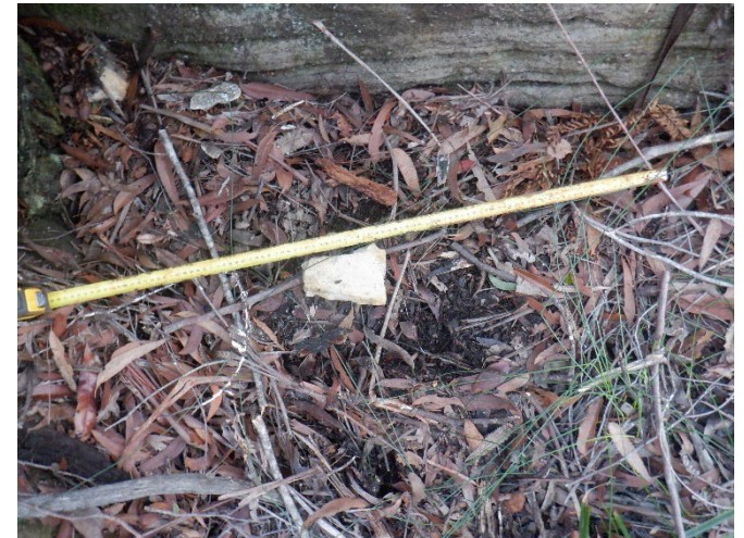
Photo 48: DA3A_LW19_055, showing area of rockfall. Taken on 04/05/2023.
