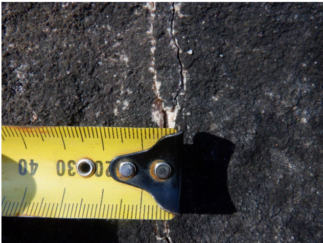
Photo 22: DA3A_LW19_017, showing rock fracturing. Taken on 13/12/2022.
