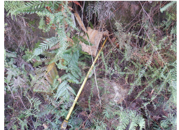
Photo 45: DA3A_LW19_052, showing rock fracturing and rockfall. Taken on 04/05/2023.
