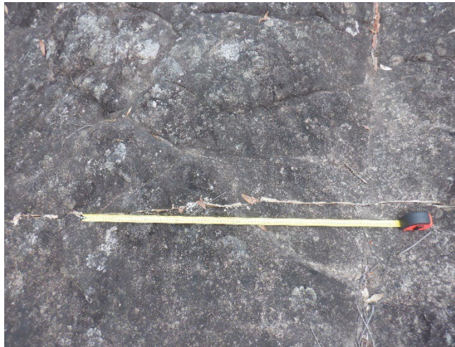
Photo 17: DA3A_LW19_012, showing rock fracturing. Taken on 7/11/2022.
