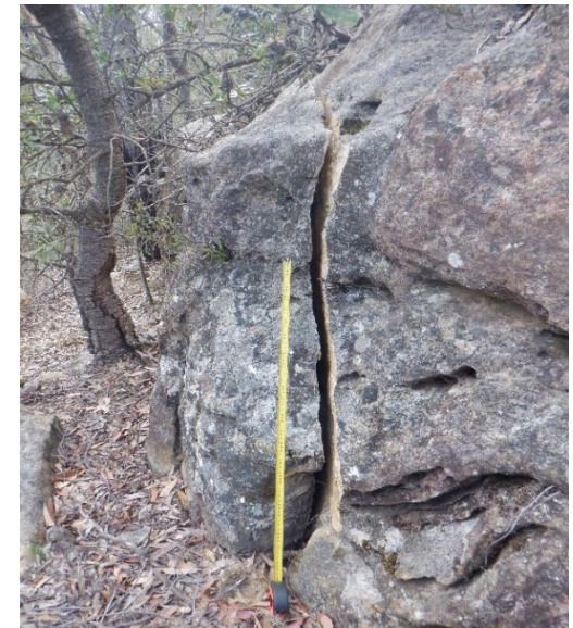
Photo 18: DA3A_LW19_013, showing rock fracturing. Taken on 7/11/2022.
