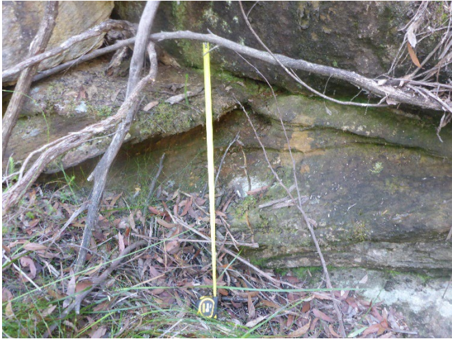
Photo 55: DA3A_LW19_062, showing rock fracturing. Taken on 05/05/2023.
