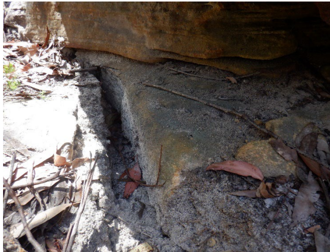
Photo 26: DA3A_LW19_021, showing soil cracking and displacement. Taken on 13/12/2022.
