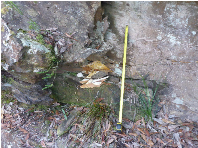
Photo 52: DA3A_LW19_059, showing rock fracturing and rockfall. Taken on 05/05/2023.
