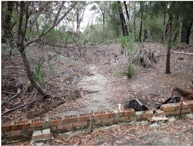
Photo 59: Erosion upstream of weir on DC13. Taken on 28/02/2023.
