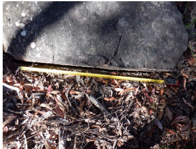
Photo 23: DA3A_LW19_018, showing rock displacement. Taken on 13/12/2022.
