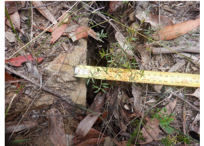
Photo 12: DA3A_LW19_007, showing soil cracking. Taken on 19/04/2023.
