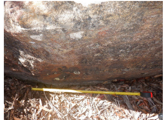
Photo 24: DA3A_LW19_019, showing rock displacement. Taken on 13/12/2022.
