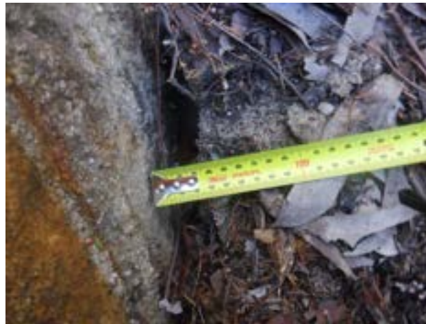
Photo 10: DA3A_LW19_048, showing rock movement. Taken on 27/04/2023.
