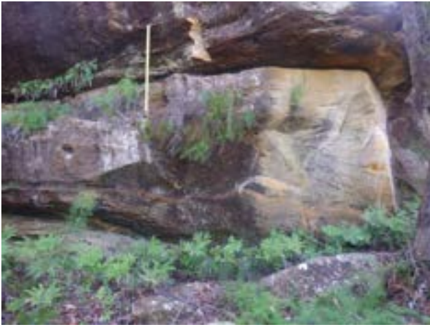
Photo 6: DA3A_LW19_047, showing steep slope/step where rock has detached from rock face. Taken on 27/04/2023
