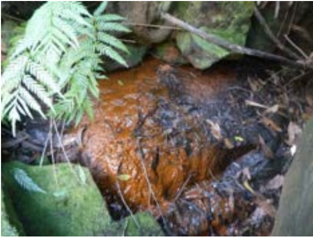
Photo 1: DA3A_LW19_045, showing iron staining appearing at base of a step. Taken on 26/04/2023.
