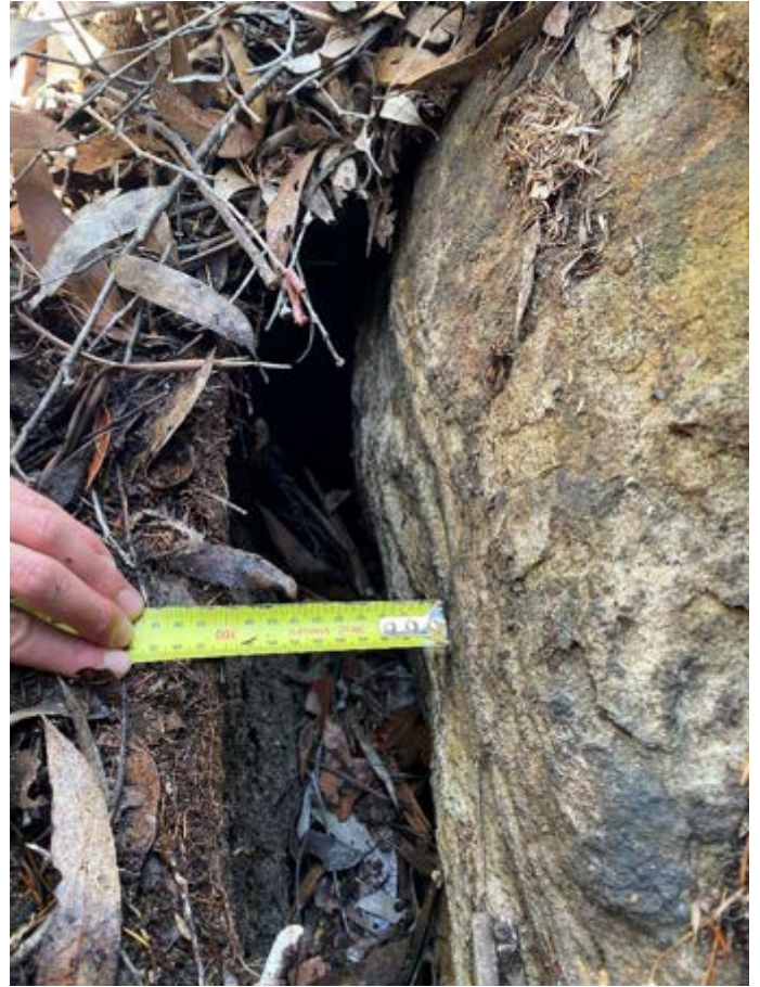
Photo 2: DA3A_LW19_035, width of the soil cracking/rock displacement. Taken on 16/03/2023.
