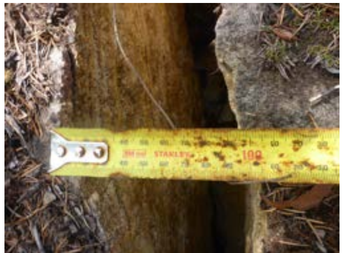
Photo 7: DA3A_LW19_025, width of rock fracturing. Taken on 17/01/2023.
