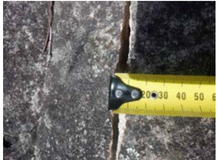
Photo 10: DA3A_LW19_012, width of rock fracturing. Taken on 7/11/2022.
