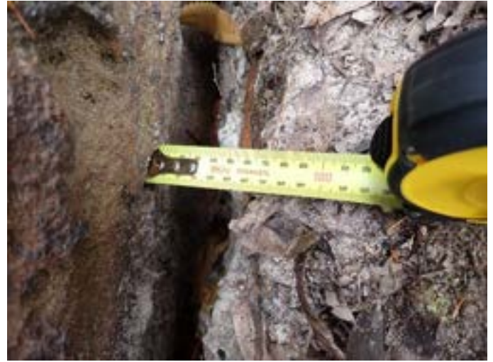
Photo 6: DA3A_LW19_025 , width of rock displacement. Taken on 20/12/2022.
