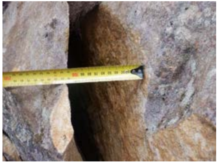
Photo 12: DA3A_LW19_013 , width of rock fracturing. Taken on 7/11/2022.
