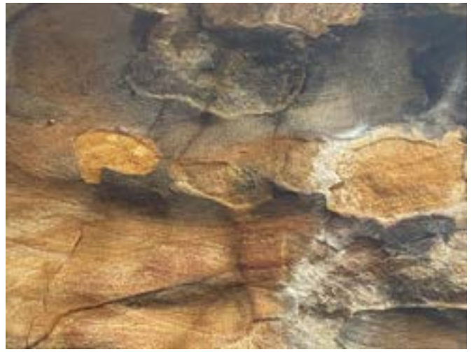
Photo 10: DA3A_LW19_038, rock fracturing extending to the upper part of overhang. Taken on 28/03/2023.
