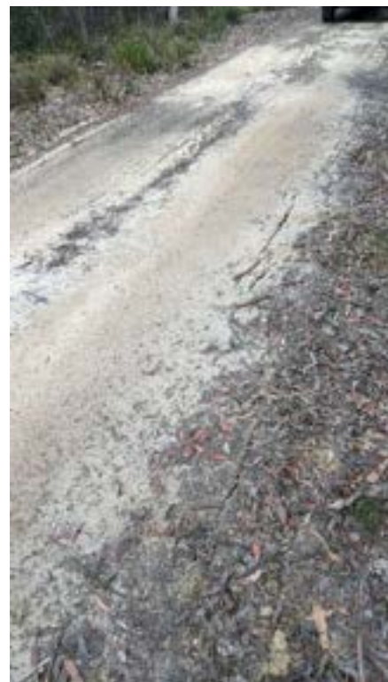
Photo 8: DA3A_LW19_026 , section of soil cracking. Taken on 21/12/2022.
