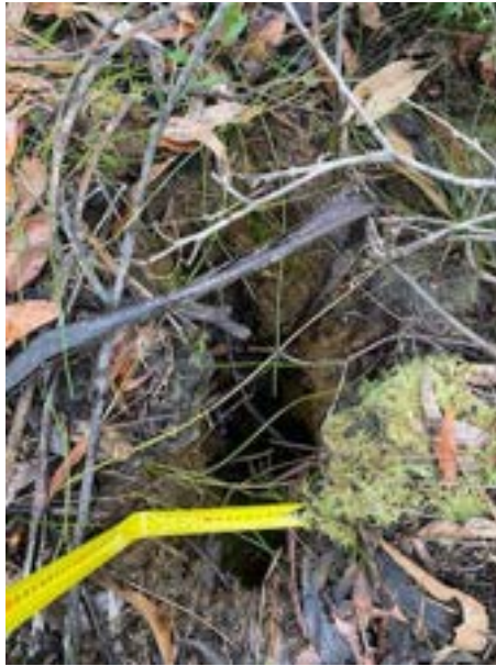
Photo 3: Width of soil crack. Taken 1/09/2022.
