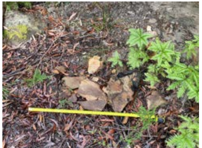
Photo 12: DA3A_LW19_038, rock fall on ground. Taken on 28/03/2023.
