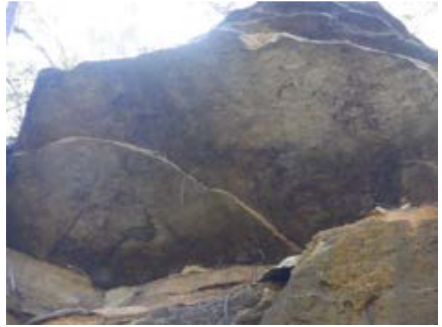
Photo 4: DA3A_LW19_046, showing steep slope/step face where rocks detached. Taken on 27/04/2023.
