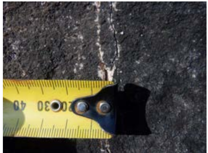
Photo 2: DA3A_LW19_017, width of rock fracturing. Taken on 13/12/2022.
