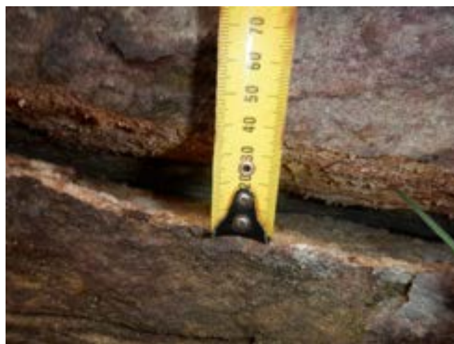
Photo 4: DA3A_LW19_005, looking at width of rock fracture. Taken on 19/08/2022.
