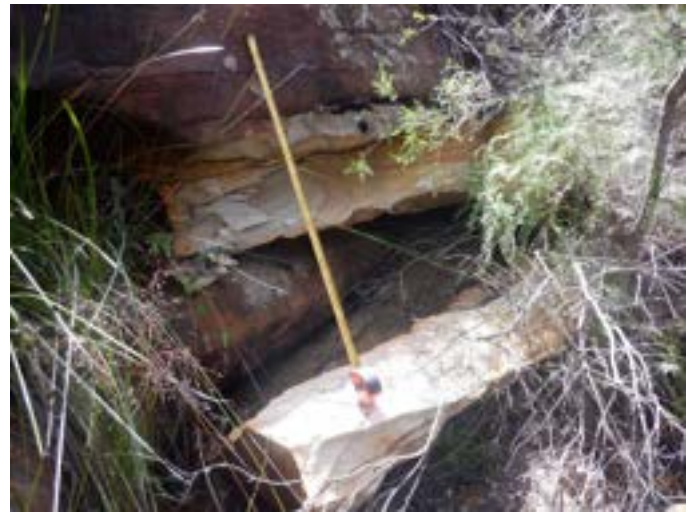
Photo 2: DA3A_LW19_027, section of rock fracturing and rockfall. Taken on 10/01/2023.
