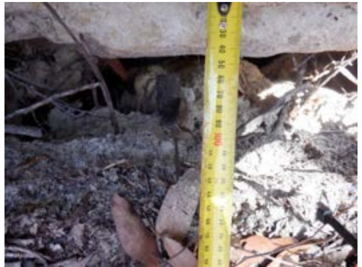
Photo 12: DA3A_LW19_021, width of soil cracking. Taken on 13/12/2022.
