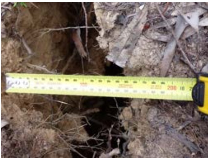
Photo 3: DA3A_LW19_024, width of soil cracking. Taken on 20/12/2022.
