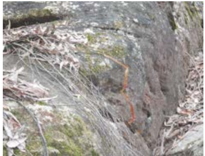
Photo 3: DA3A_LW19_005, looking at section of rock fracturing. Taken on 19/08/2022.
