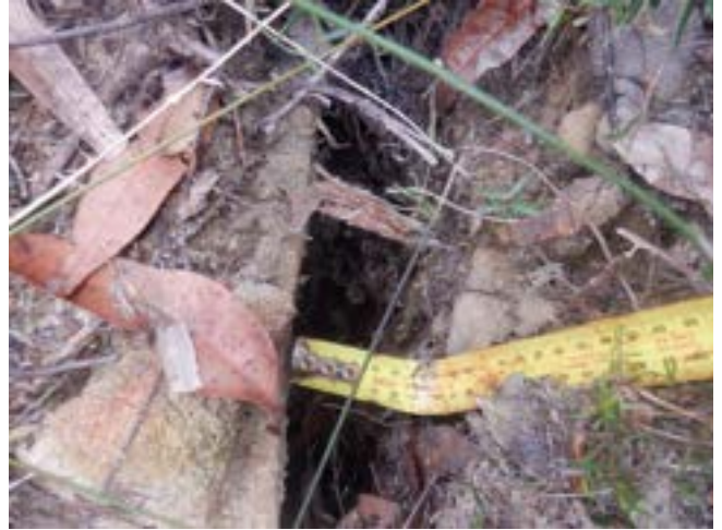
Photo 2: DA3A_LW19_007, width of soil cracking. Taken on 18/10/2022.
