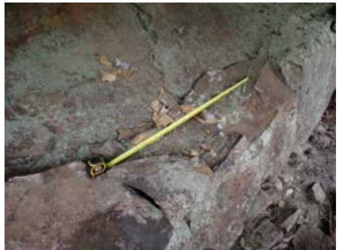
Photo 16: DA3A_LW19_042 looking at rockfall and associated fragments. Taken 12/04/2023.
