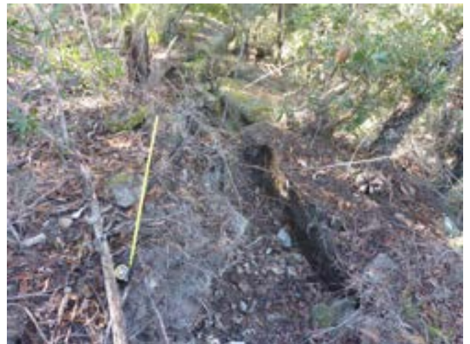
Photo 12: DA3A_LW19_056, showing top view of block that have moved away from the adjacent ground. Taken on 5/05/2023.
