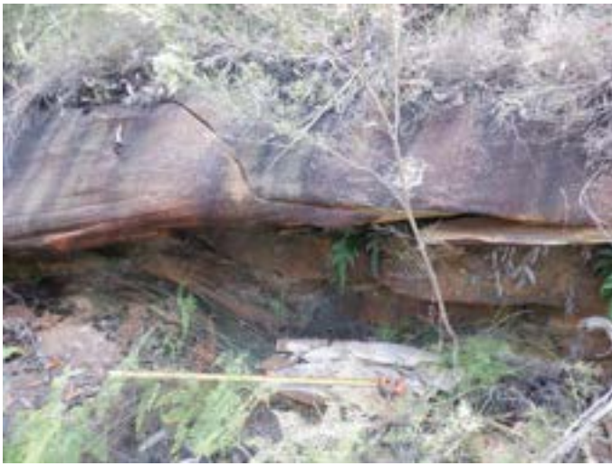
Photo 1: DA3A_LW19_027, section of rock fracturing and rockfall. Taken on 10/01/2023.
