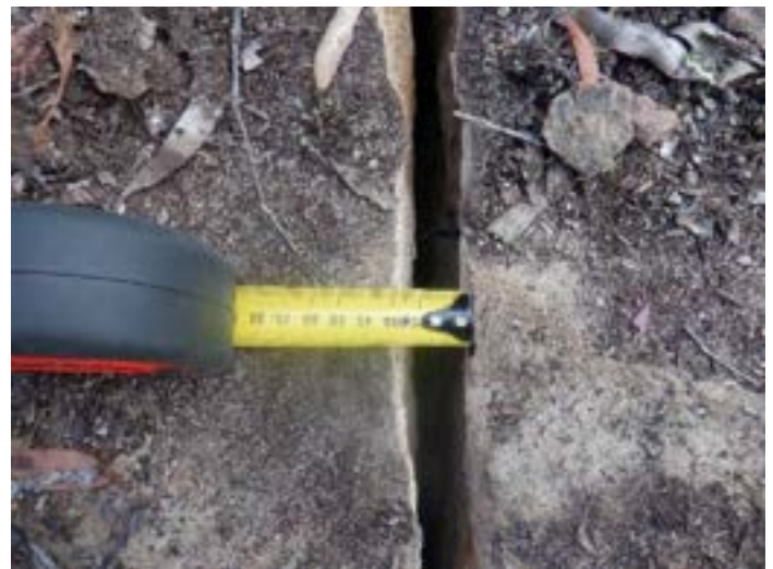
Photo 2: DA3A_LW19_008, width of rock fracturing. Taken on 7/11/2022.
