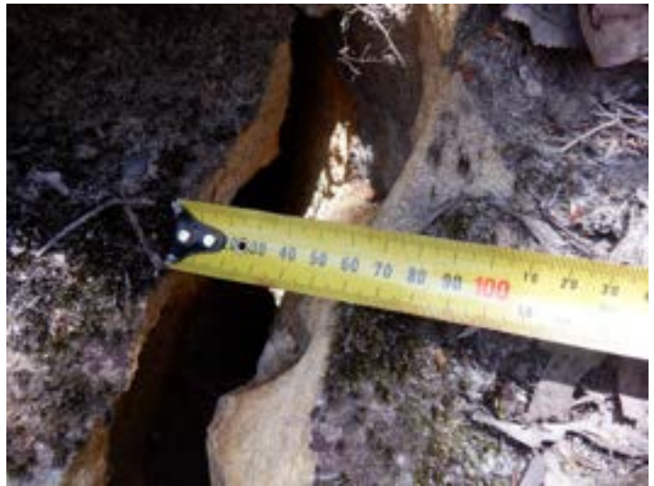
Photo 18: DA3A_LW19_023 , width of rock displacement. Taken on 13/12/2022.
