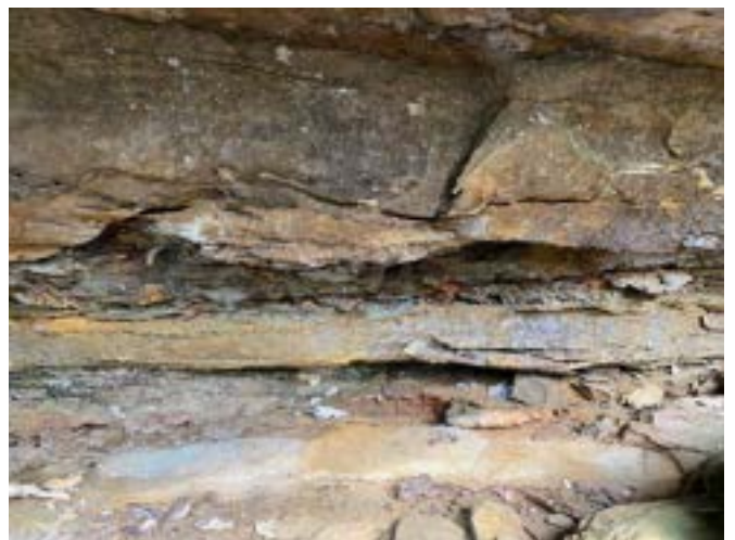
Photo 6: DA3A_LW19_037, rock fracturing through overhang at Sandy Creek 21. Taken on 28/03/2023.
