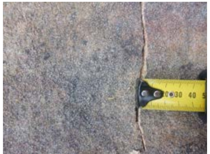
Photo 8: DA3A_LW19_011 , width of rock fracturing. Taken on 7/11/2022.
