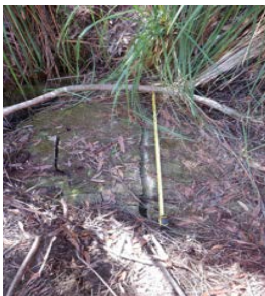
Photo 1: DA3A_LW19_051 , showing rock fracturing to an outcrop on WC14 . Taken on 4/5/2023.
