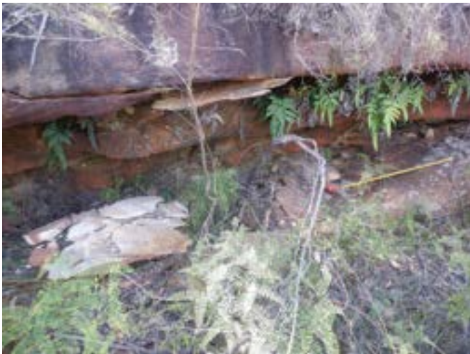
Photo 3: DA3A_LW19_027, section of rock fracturing and rockfall. Taken on 10/01/2023.
