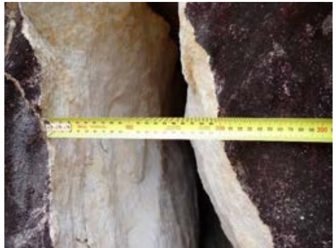
Photo 10: DA3A_LW19_015, width of rock fracturing. Taken on 20/12/2022.
