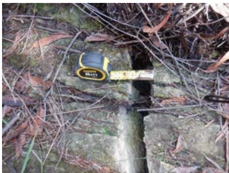
Photo 2: DA3A_LW19_051 , showing width of rock fracture. Taken on 4/5/2023.
