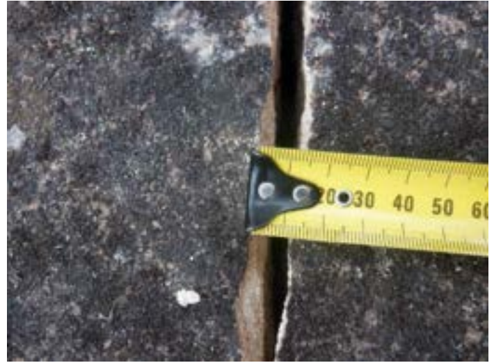
Photo 4: DA3A_LW19_009 , width of rock fracturing. Taken on 7/11/2022.
