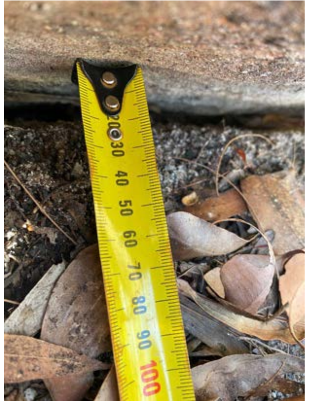
Photo 4: DA3A_LW19_018 , width of rock displacement. Taken on 13/12/2022.
