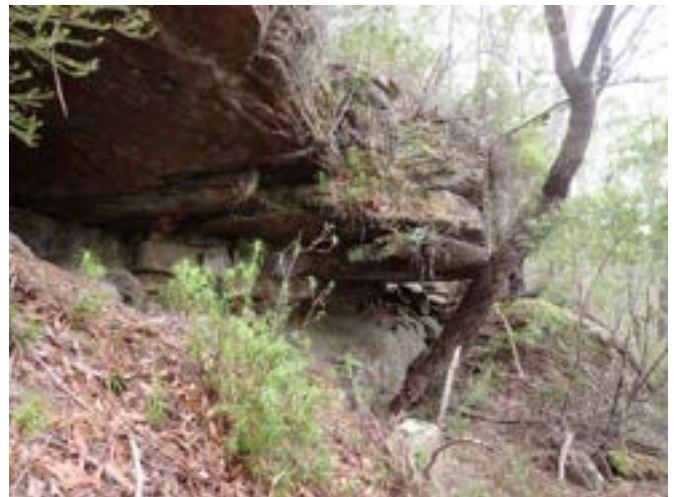
Photo 14: LW19_SS4 during its most recent inspection. Taken 12/04/2023.
