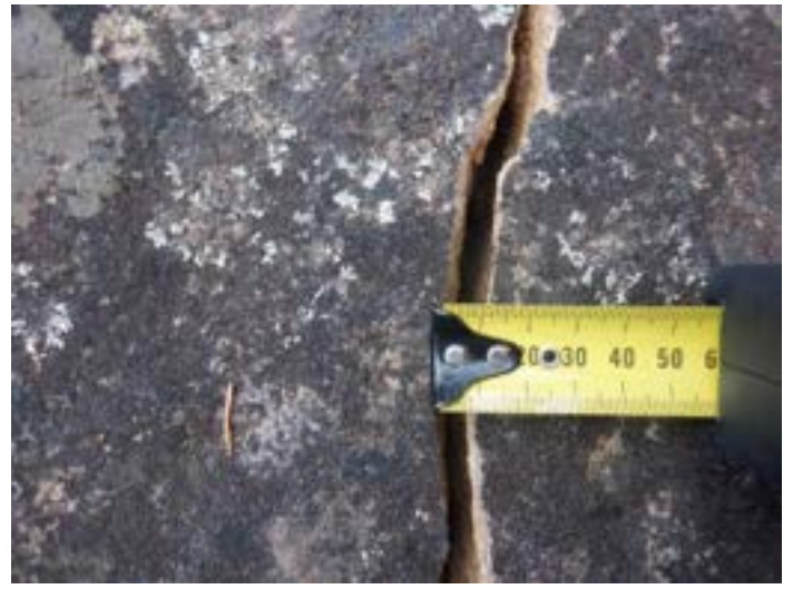
Photo 6: DA3A_LW19_010 , width of rock fracturing. Taken on 7/11/2022.
