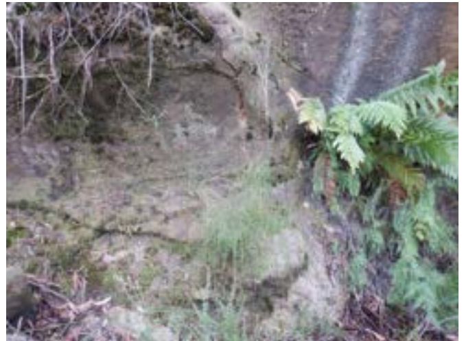
Photo 6: DA3A_LW19_053 , showing rock fracturing. Taken on 4/5/2023
