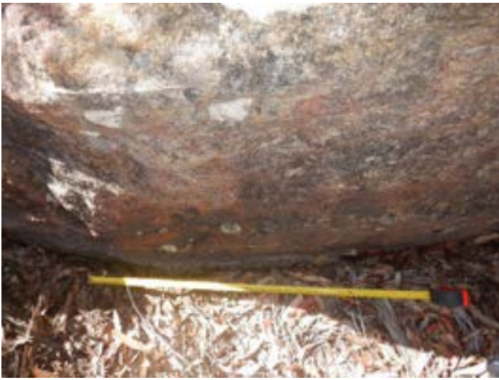
Photo 5: DA3A_LW19_019, section of rock displacement. Taken on 13/12/2022.
