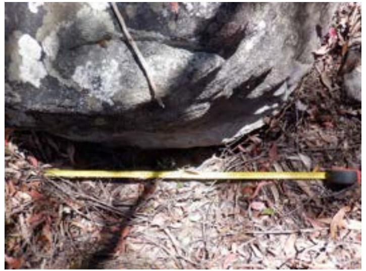
Photo 10: DA3A_LW19_021, section of rock displacement. Taken on 13/12/2022.
