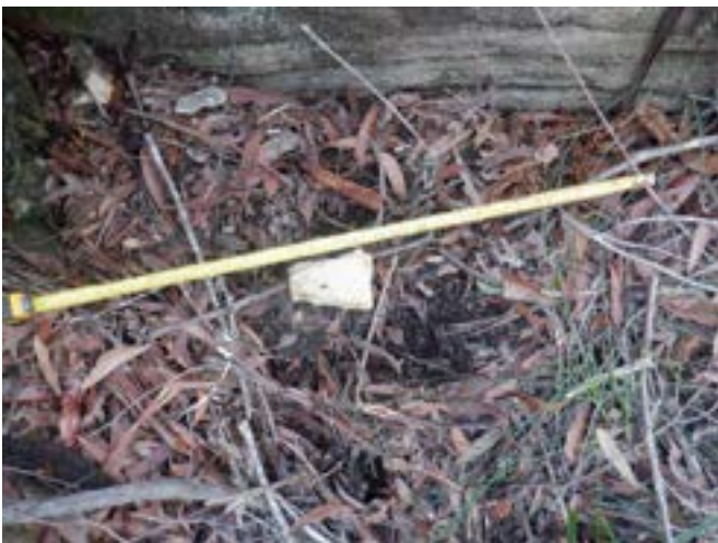
Photo 9: DA3A_LW19_055 , showing area of rockfall. Taken on 4/5/2023.
