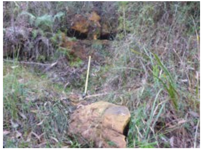
Photo 14: DA3A_LW19_057 , showing step where rocks detached and debris area. Taken on 5/05/2023.
