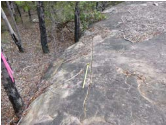
Photo 1: DA3A_LW19_030, rock fracturing to an outcrop. Taken on 15/2/2023.
