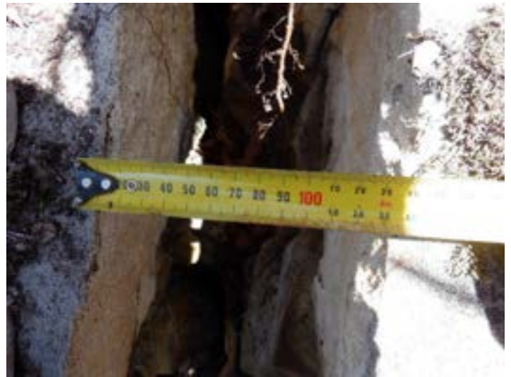
Photo 14: DA3A_LW19_022, width of rock fracturing. Taken on 13/12/2022.
