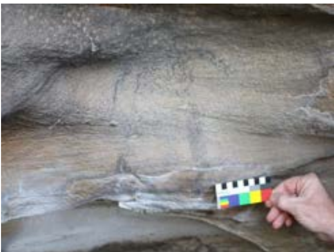
Photo 13: Art at DM15- baseline image displaying horizontal rock fracture identified prior to mining. Taken circa October 2020.
