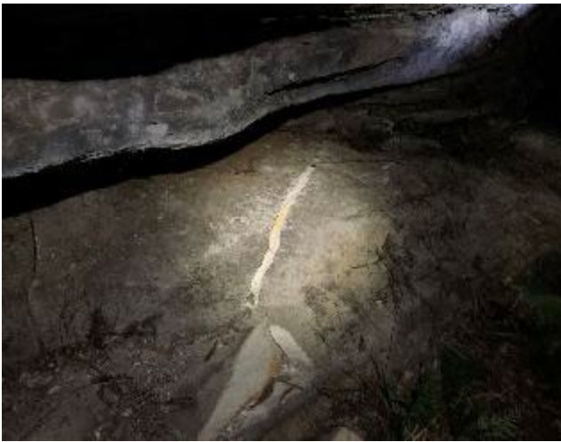
Plate 18: WC15 bedrock cracking
