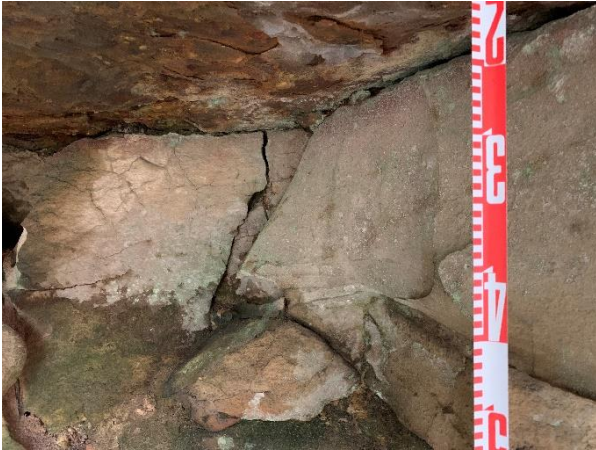
Plate 13: Close up of vertical crack #1, location at 11.5m. Taken on 24 June 2022.
