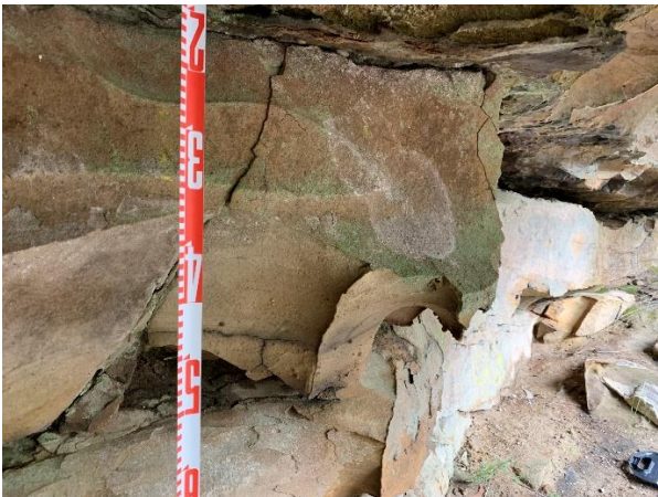
Plate 15: Close up of vertical crack #2, location at 12.13m (General view displayed in Plate 11 and Plate 16 as comparison photos). Taken on 24 June 2022.
