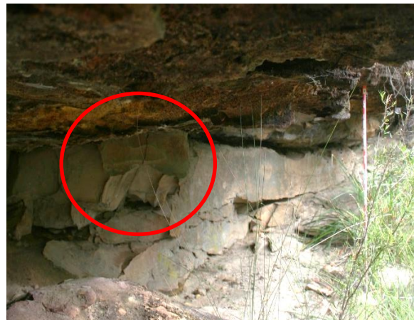
Plate 16: Cropped comparison photo of Plate 12 taken by Biosis during baseline monitoring (2103). Red circle highlights evidence of cracking (crack#2) prior to Longwall 18 extraction.
