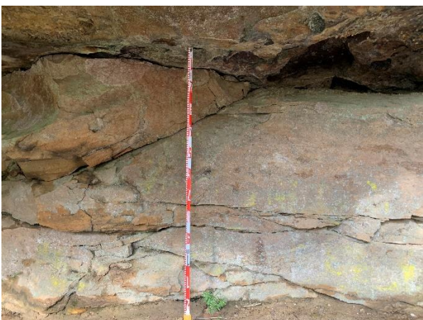
Plate 17: General view of vertical crack #3, location at 12.98m. Taken on 24 June 2022.
