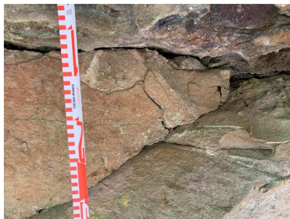
Plate 18: Close up of vertical crack #3. Taken on 24 June 2022.
