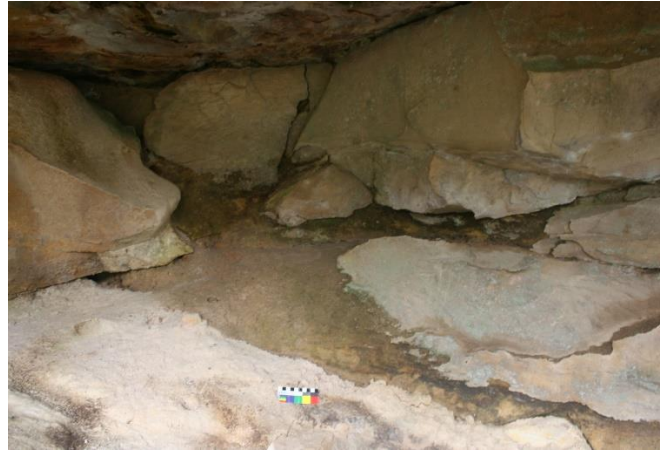
Plate 14: Comparison photo of vertical crack #1. Photo taken during baseline recording by Biosis and provided by IMC.
