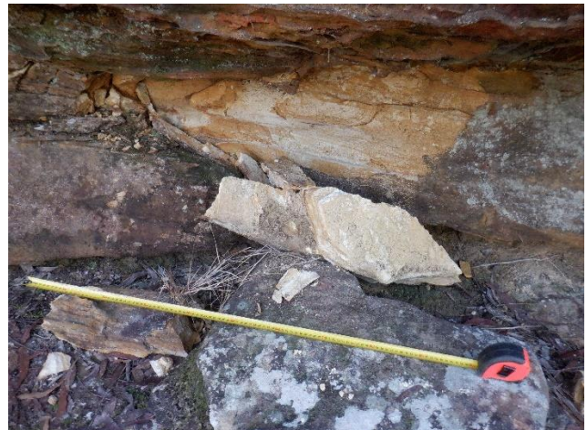
Photo 6: DA3B_LW18_014, showing rockfall debris. Taken 16/08/2022.
