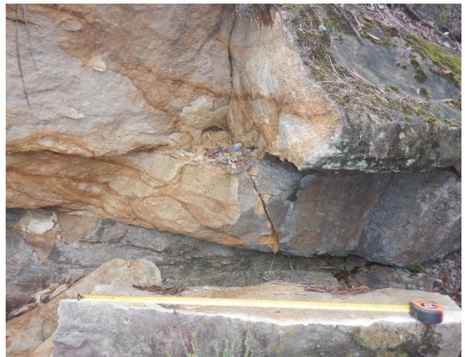
Photo 26: DA3B_LW18_022 , showing section of rockfall/debris. Taken 16/08/2022.
