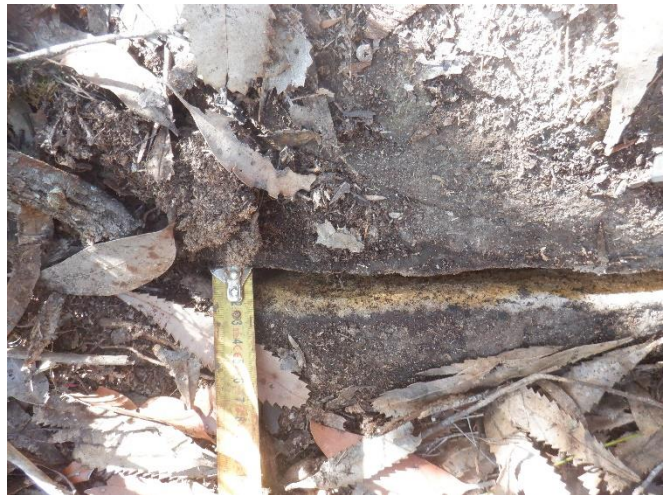
Photo 2: DA3B_LW18_002 , showing the width of the fracturing. Taken 31/01/2022.
