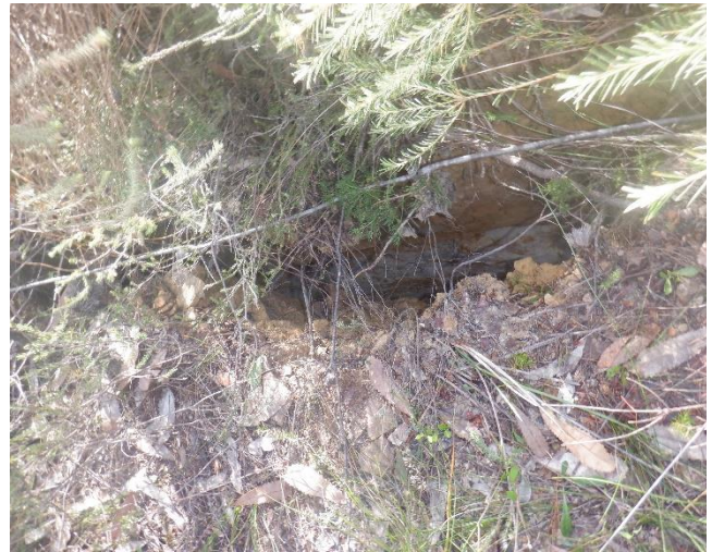
Photo 28: DA3B_LW18_023, showing maximum width of soil cracking. Taken 16/08/2022.
