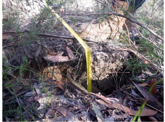
Photo 4: DA3B_LW18_008 , showing the depth of soil cracking. Taken 9/06/2022.
