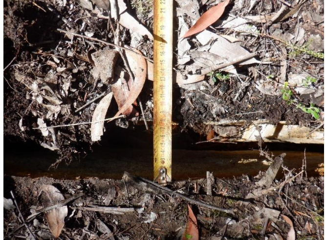
Photo 4: DA3B_LW18_003 , showing the width of the fracturing. Taken 31/01/2022.
