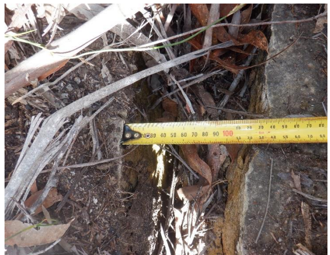
Photo 22: DA3B_LW18_021 , showing maximum width of rock fracturing. Taken 16/08/2022.
