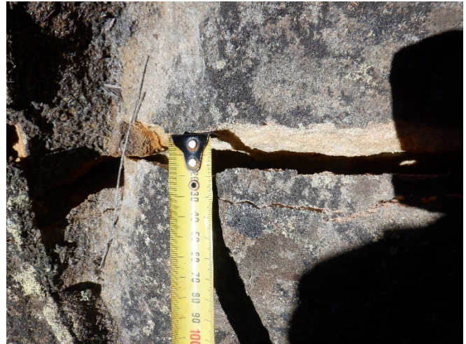
Photo 2: DA3B_LW18_004 , showing the width of the fracturing. Taken 9/02/2022.
