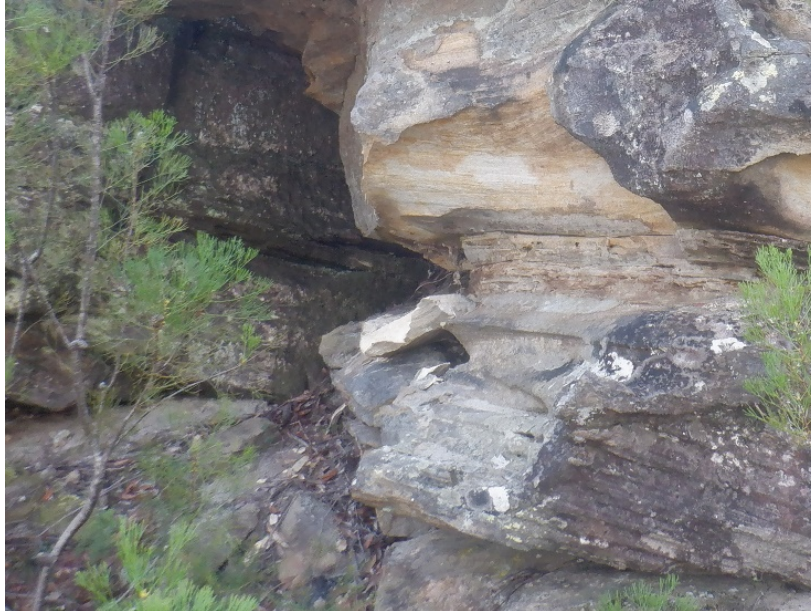
Photo 11: DA3B_LW18_011 , showing rockfall. Taken 10/06/2022.
