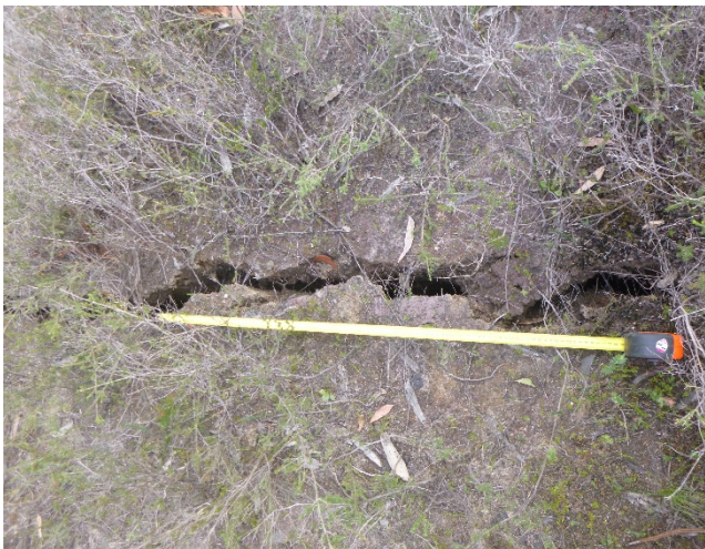
Photo 1: DA3B_LW18_005, showing a section of soil cracking. Taken 30/06/2022.
