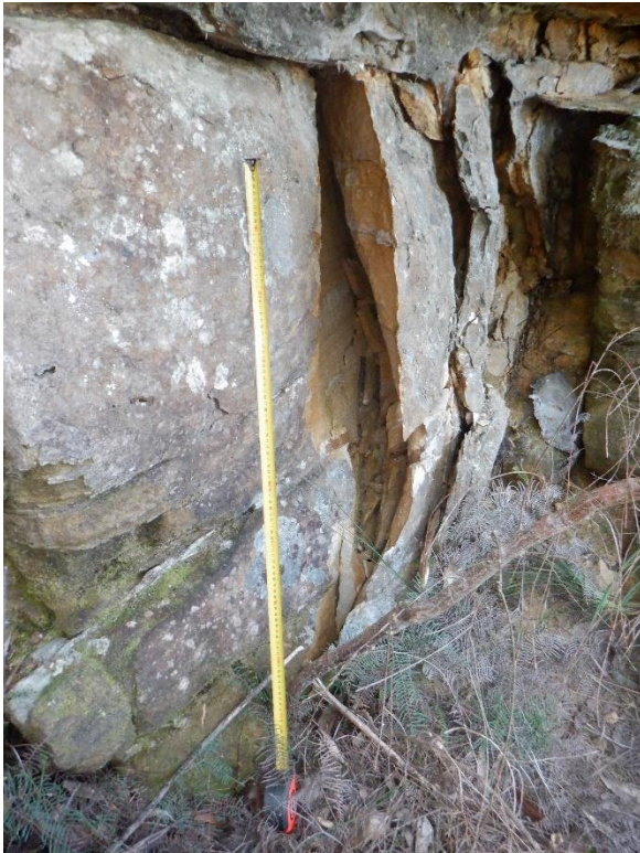
Photo 11: DA3B_LW18_017, showing rock displacement. Taken 16/08/2022.
