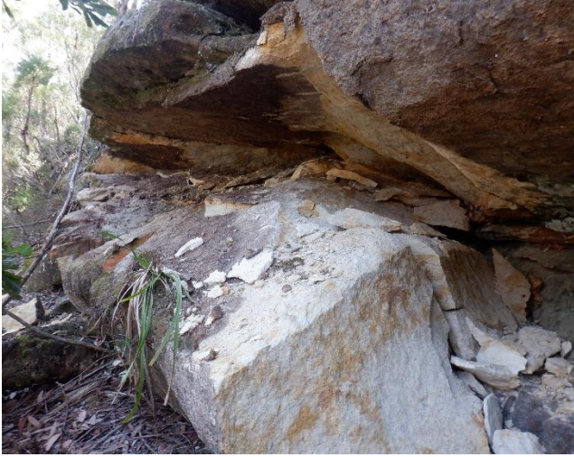
Photo 19: DA3B_LW18_020 , showing overview of impact. Taken 16/08/2022.
