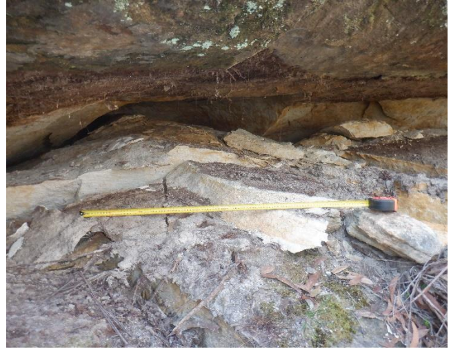
Photo 20: DA3B_LW18_020 , showing rockfall closer up. Taken 16/08/2022.
