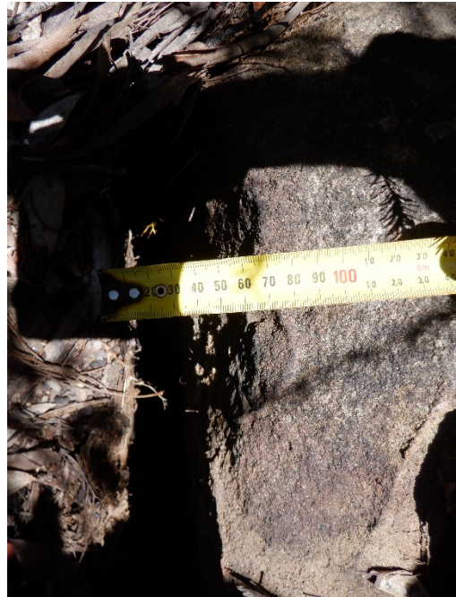
Photo 4: DA3B_LW18_005, showing the width of the displacement. Taken 9/02/2022.
