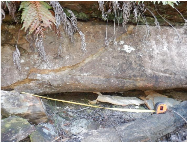
Photo 5: DA3B_LW18_014, showing section of rock fracturing. Taken 16/08/2022.
