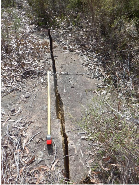
Photo 23: DA3B_LW18_021 , showing overview of largest fracture. Taken 16/08/2022.
