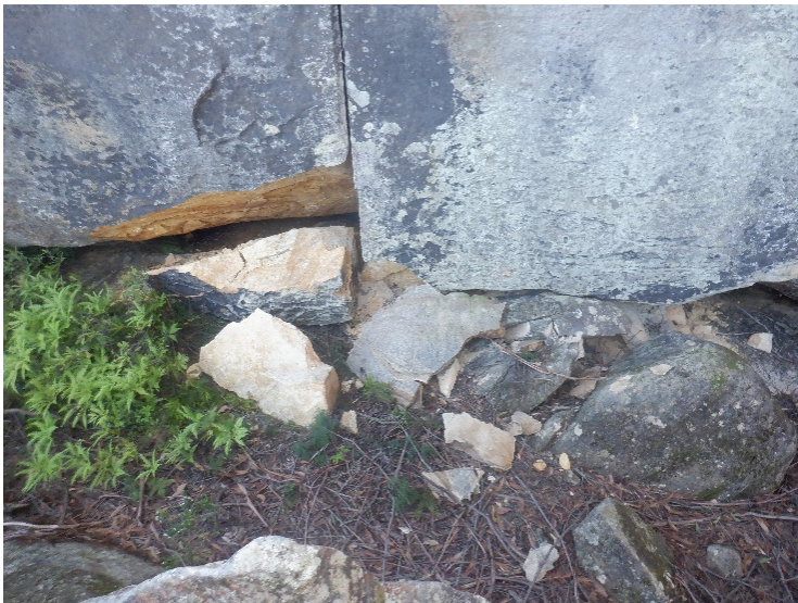
Photo 9: DA3B_LW18_010 , showing rock fall and fragmentation. Taken 10/06/2022.
