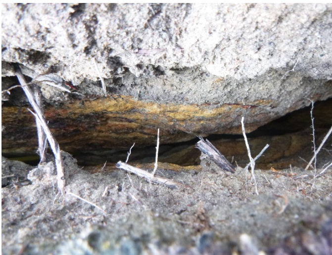
Photo 5: DA3B_LW18_012, showing exposed rock within the cracking. Taken 30/06/2022.
