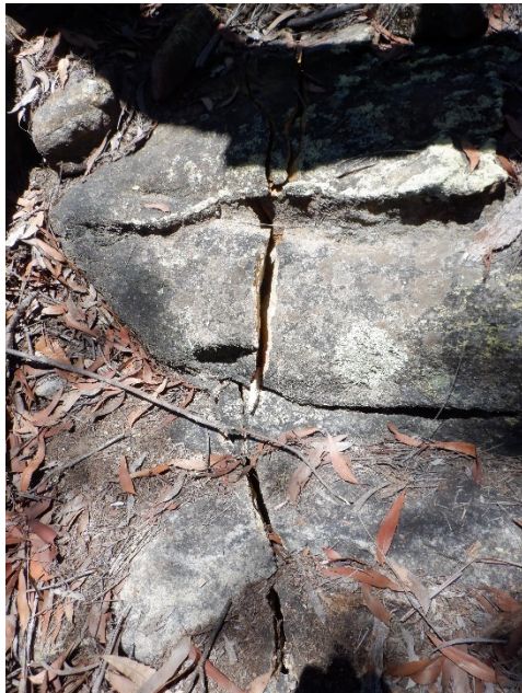
Photo 1: DA3B_LW18_004 , showing the length of rock fracturing. Taken 9/02/2022.
