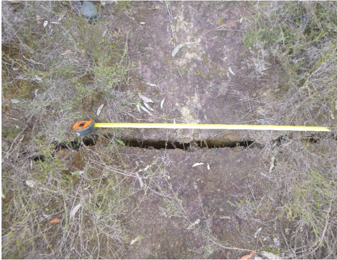
Photo 3: DA3B_LW18_012, showing a section of soil cracking. Taken 30/06/2022.
