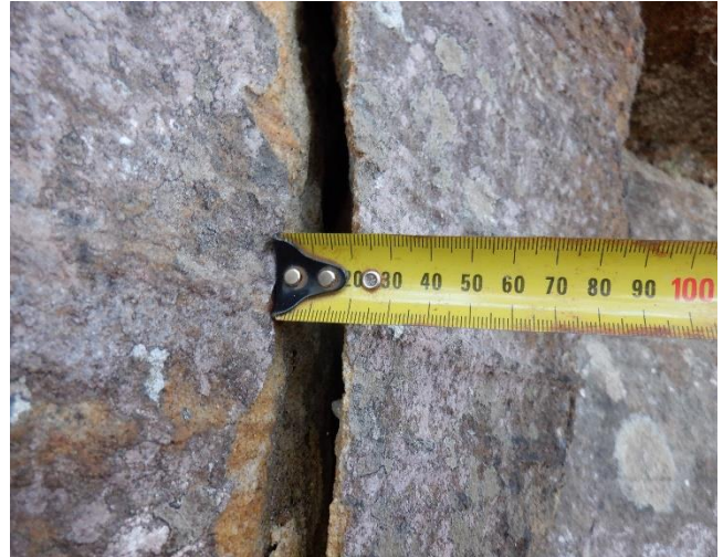
Photo 8: DA3B_LW18_015 , showing width of rock fracture. Taken 16/08/2022.
