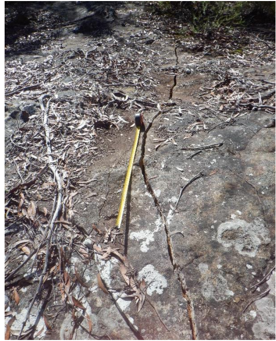
Photo 24 DA3B_LW18_021 , showing section of rock fracturing. Taken 16/08/2022.
