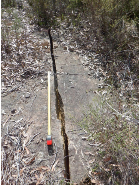
Photo 71: DA3B_LW18_021 , showing overview of largest fracture. Taken 16/08/2022.
