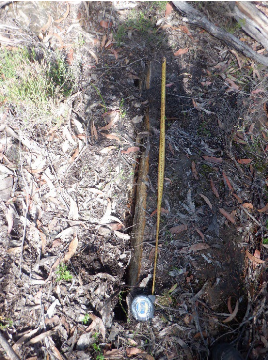
Photo 22: DA3B_LW18_003 , showing a section of rock fracturing. Taken 31/01/2022.
