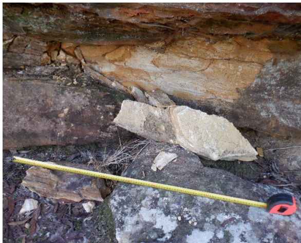
Photo 54: DA3B_LW18_014 , showing rockfall debris. Taken 16/08/2022.
