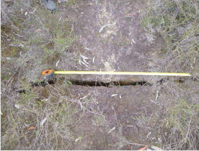
Photo 46: DA3B_LW18_012 , showing a section of soil cracking. Taken 30/06/2022.
