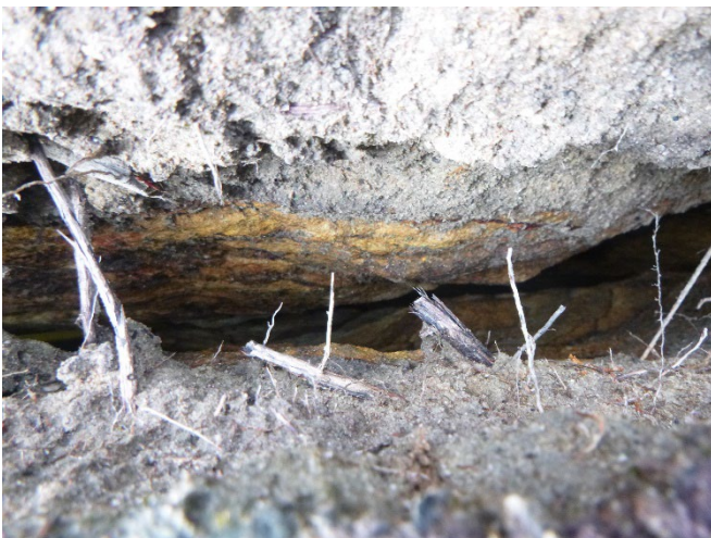
Photo 48: DA3B_LW18_012 , showing exposed rock within the cracking. Taken 30/06/2022.
