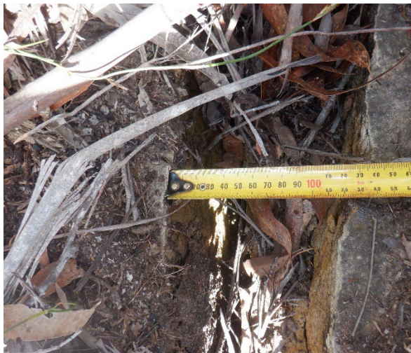
Photo 70: DA3B_LW18_021 , showing maximum width of rock fracturing. Taken 16/08/2022.
