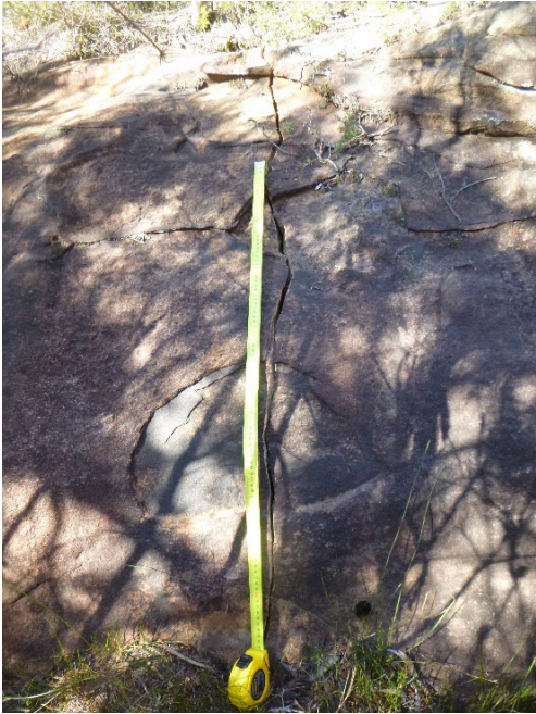
Photo 35: DA3B_LW18_007 , showing a section of rock fracturing. Taken 8/06/2022.
