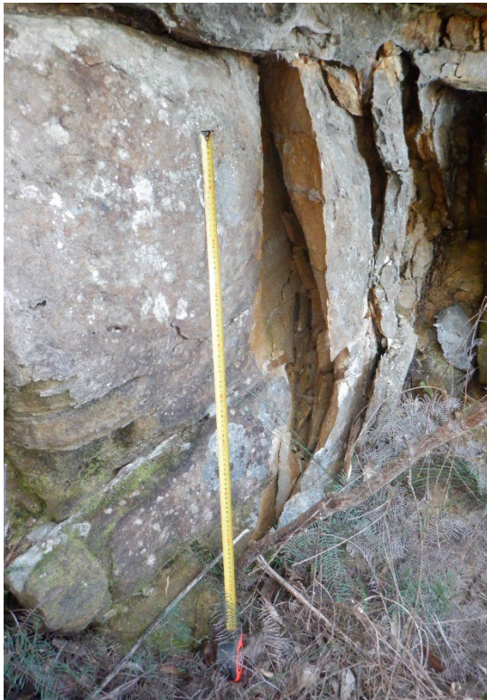
Photo 59: DA3B_LW18_017, showing rock displacement. Taken 16/08/2022.
