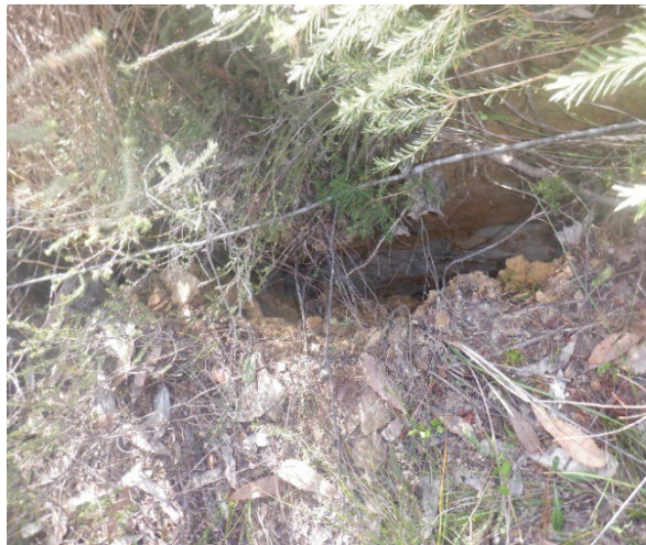
Photo 76: DA3B_LW18_023, showing maximum width of soil cracking. Taken 16/08/2022.
