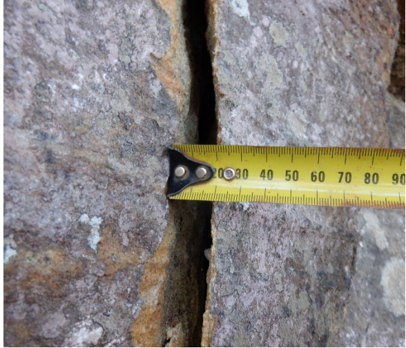
Photo 56: DA3B_LW18_015 , showing width of rock fracture. Taken 16/08/2022.
