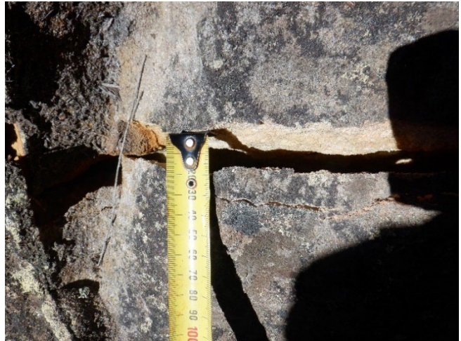
Photo 26: DA3B_LW18_004 , showing the width of the fracturing. Taken 9/02/2022.
