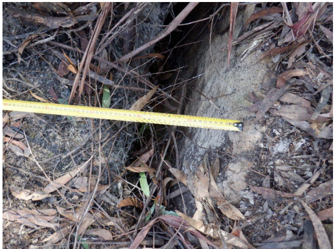
Photo 40: DA3B_LW18_009, showing the width of rock displacement. Taken 9/06/2022.
