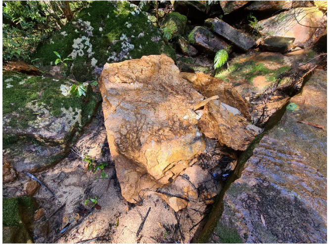
Photo 12: DA3B_LW17_041 , showing a section of potential rock fall. Taken 2/08/2022.
