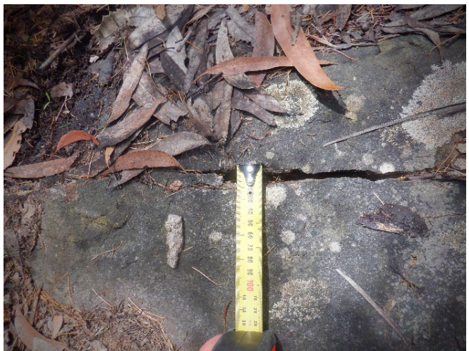
Photo 18: DA3B_LW18_001, showing the width of the fracturing. Taken 14/12/2021.
