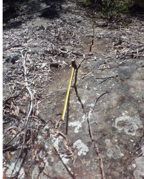
Photo 72: DA3B_LW18_021 , showing section of rock fracturing. Taken 16/08/2022.
