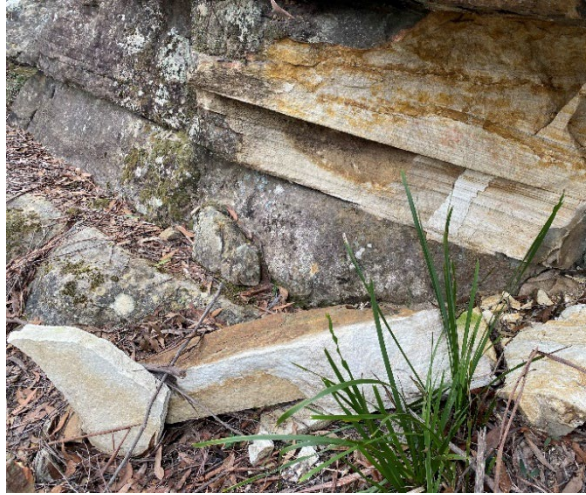
Photo 62: DA3B_LW18_018 , showing section of rockfall. Taken 16/08/2022.
