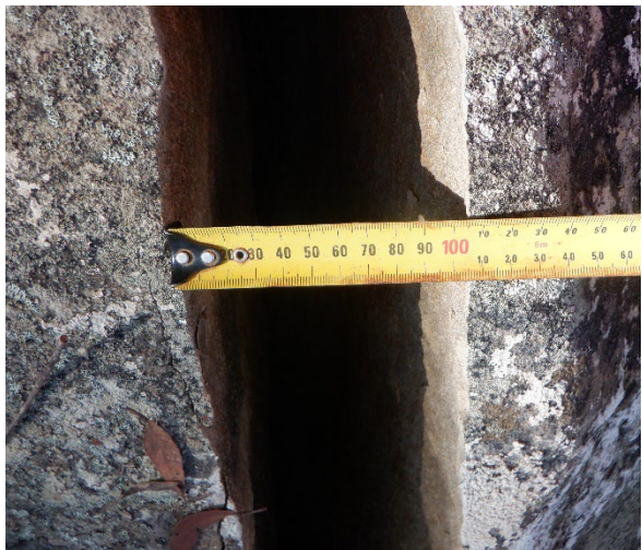
Photo 58: DA3B_LW18_016 , showing maximum width of rock fracturing. Taken 16/08/2022
