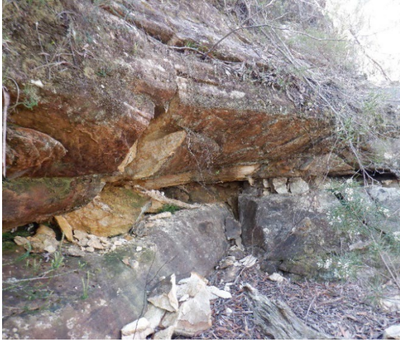
Photo 61: DA3B_LW18_018 , showing section of rockfall and rock fracturing. Taken 16/08/2022.
