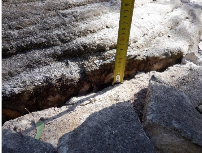
Photo 8: DA3B_LW17_012 , displacement of rockbar on LA2. Taken on 10/09/2021.
