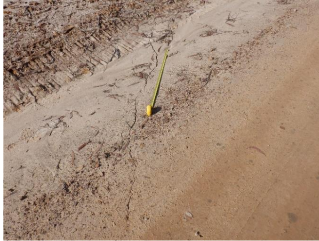
Photo 33: DA3B_LW17_018 , soil cracking on Fire Road 6A. Taken on 25/05/2021.
