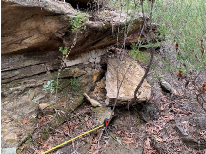
Photo 26: DA3B_LW17_035 , rock fracturing and rockfall west of Fire Road 6A . Taken on 15/09/2021.
