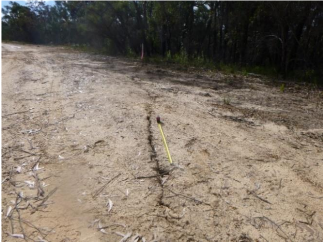
Photo 38: DA3B_LW17_030 , soil cracking on Fire Road 6A . Taken on 26/07/2021.
