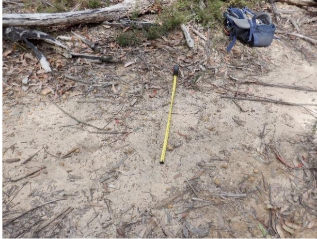
Photo 39: DA3B_LW17_033 , soil cracking on access track. Taken on 23/08/2021.
