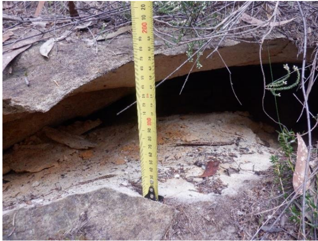
Photo 2: DA3B_LW17_002, width of rock fracturing on LA2. Taken on 10/09/2021.
