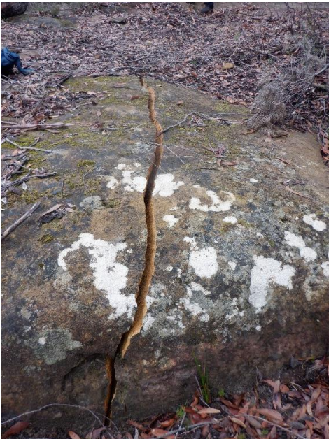
Photo 23: DA3B_LW17_023 , rock fracturing east of Fire Road 6A . Taken on 22/06/2021.
