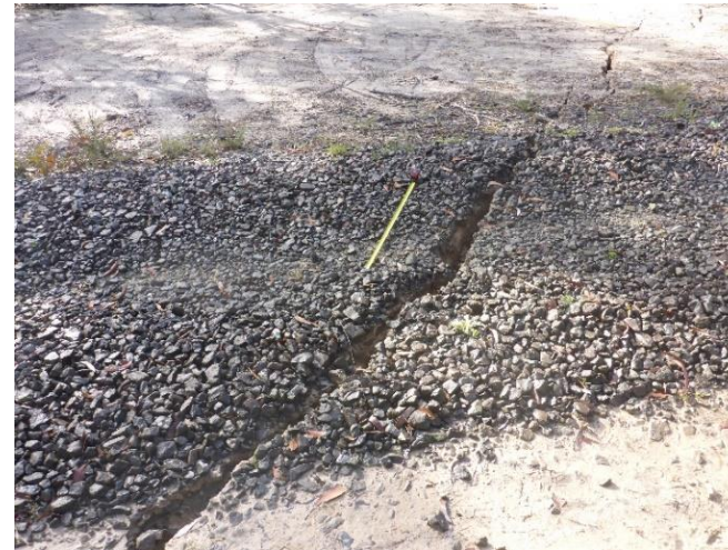
Photo 41: DA3B_LW17_027, soil cracking extending over railway corridor. Taken on 15/07/2021.
