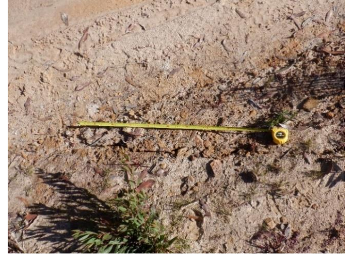
Photo 34: DA3B_LW17_020 , soil cracking on Fire Road 6A. Taken on 8/06/2021.
