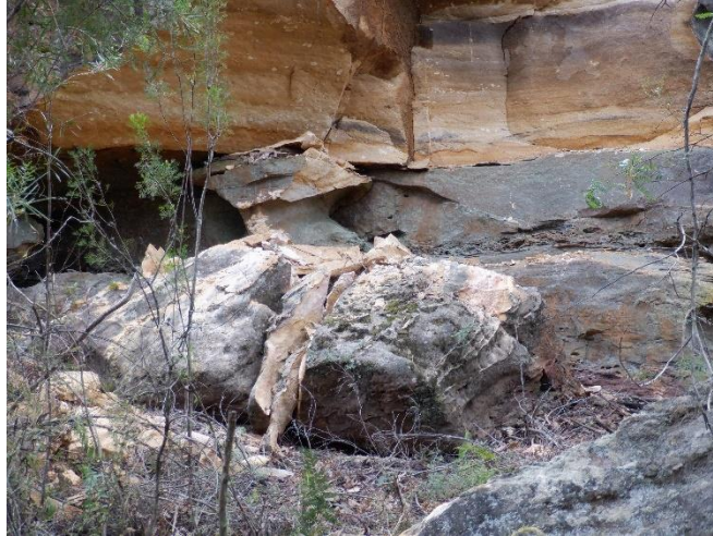
Photo 15: DA3B_LW17_009, rockfall north of LA2. Taken on 10/03/2021.
