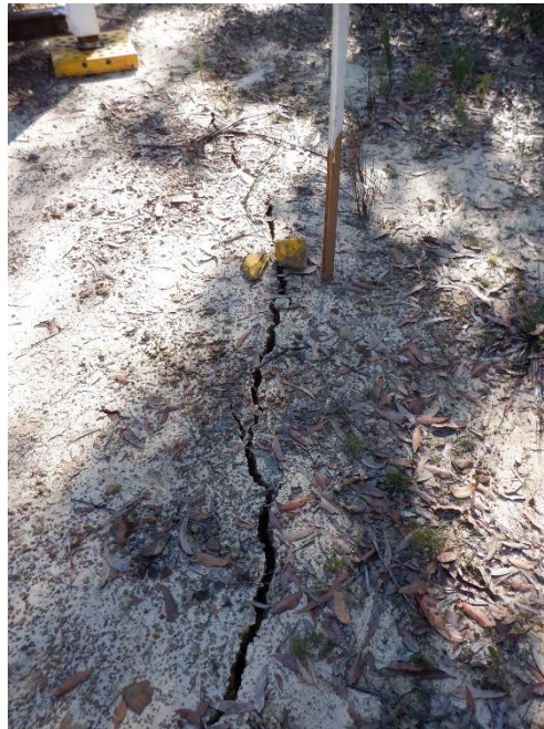
Photo 40: DA3B_LW17_014, soil cracking extending over Fire Road 6A . Taken on 18/05/2021.
