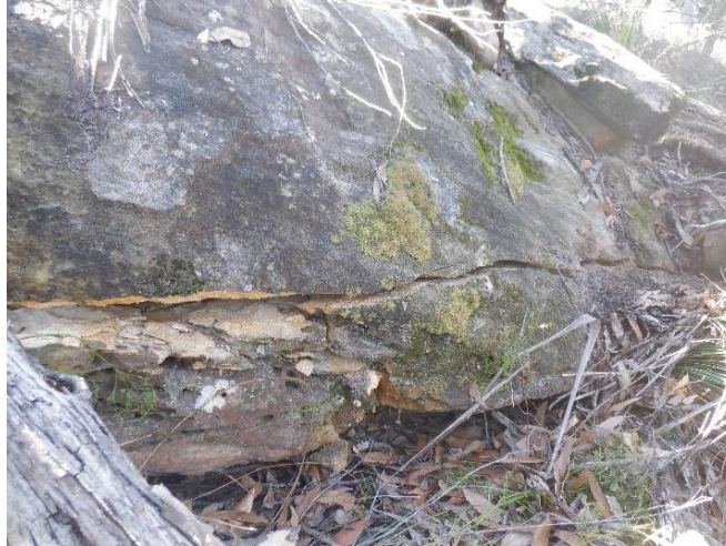
Photo 21: DA3B_LW17_021 , rock fracturing west of Fire Road 6A . Taken on 8/06/2021.
