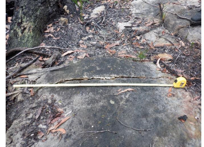
Photo 22: DA3B_LW17_022 , rock fracturing east of Fire Road 6A . Taken on 22/06/2021.
