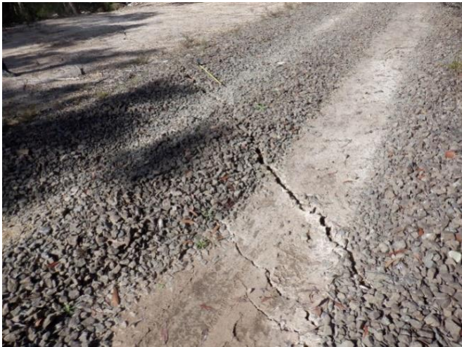
Photo 35: DA3B_LW17_026 , soil cracking on railway corridor. Taken on 7/07/2021.
