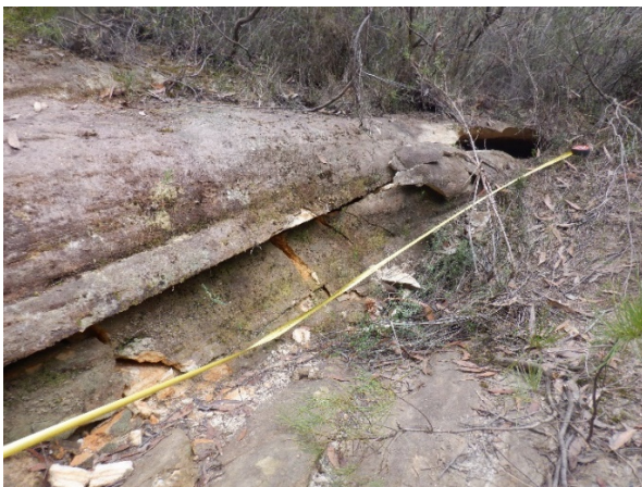
Photo 18: DA3B_LW17_002, looking at a section of rock fracturing. Taken on 10/09/2021.
