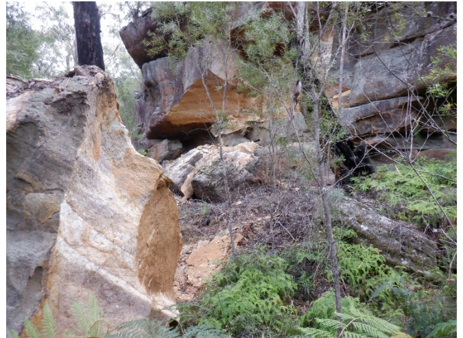
Photo 58: DA3B_LW17_009, looking at a section of rockfall. Taken on 10/03/2021.
