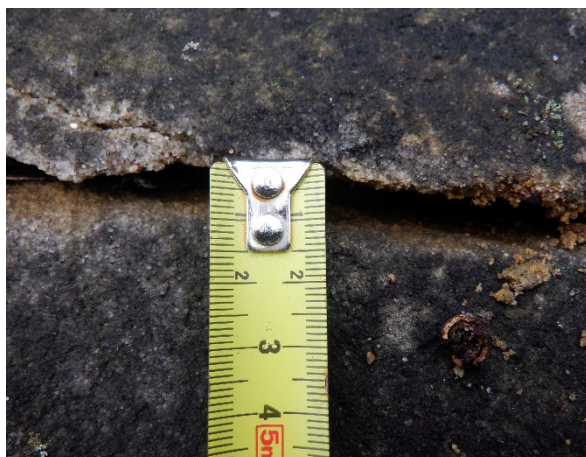
Photo 77: DA3B_LW17_022, looking at width of fracture. Taken on 22/06/2021.
