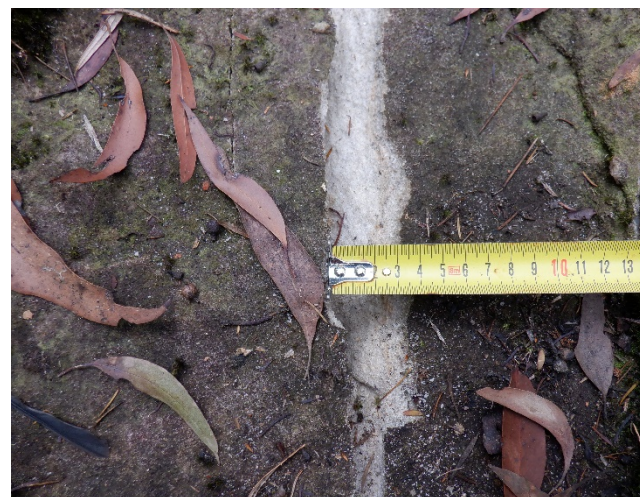
Photo 17: DA3B_LW17_007, looking at the width of the rock fracturing. Taken on 10/03/2021.
