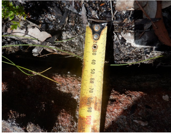
Photo 100: DA3B_LW17_039 showing the width of the void. Taken 21/10/2021.
