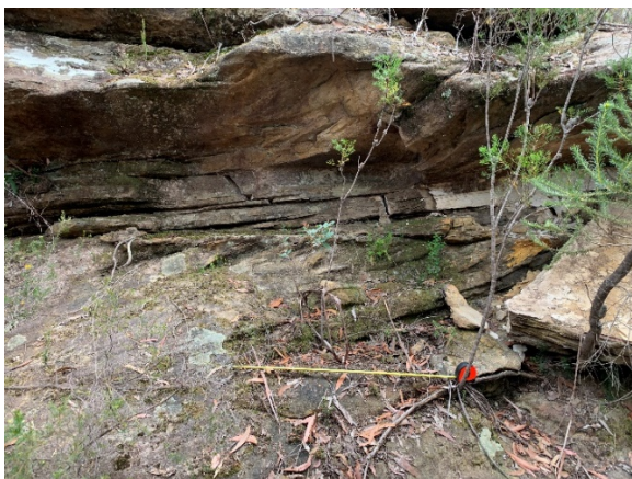
Photo 86: DA3B_LW17_035, showing the length of rock fracturing. Taken 15/9/2021.
