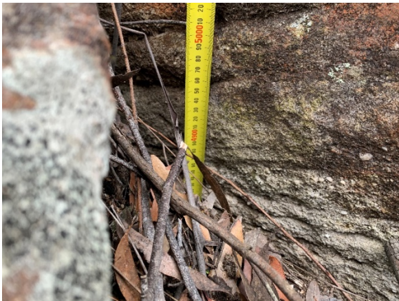
Photo 98: DA3B_LW17_038, looking at the depth of rock displacement. Taken 15/9/2021
