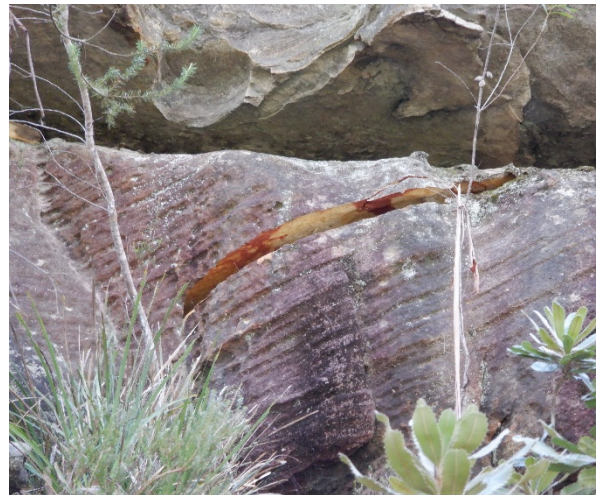
Photo 66: DA3B_LW17_011, zoomed in photo of fracture to step. Taken on 13/04/2021.
