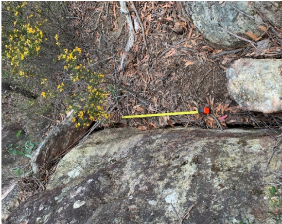
Photo 96: DA3B_LW17_038, looking at a section of rock displacement/ soil cracking. Taken 15/9/2021.
