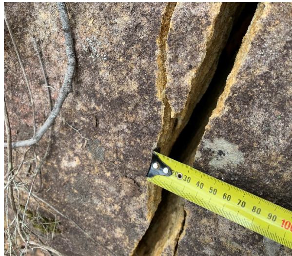
Photo 90: DA3B_LW17_036, looking at the width of the rock fracture. Taken 15/9/2021.
