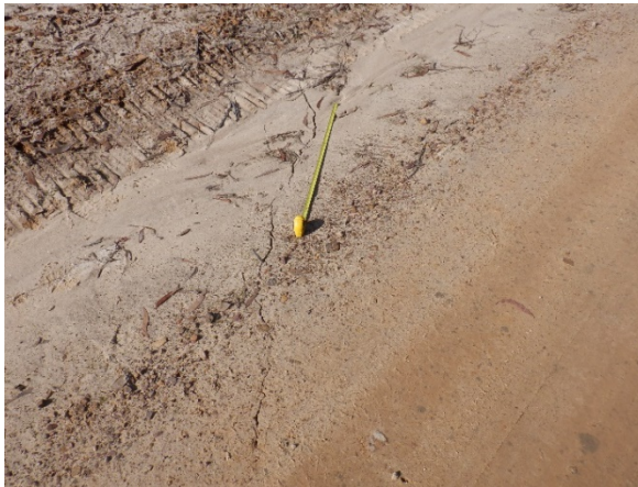
Photo 109: DA3B_LW17_018 – section of soil cracking. Taken on 25/05/2021.
