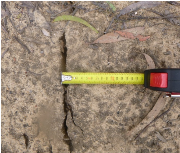
Photo 115: DA3B_LW17_028- soil cracking on access track. Taken on 26/07/2021.
