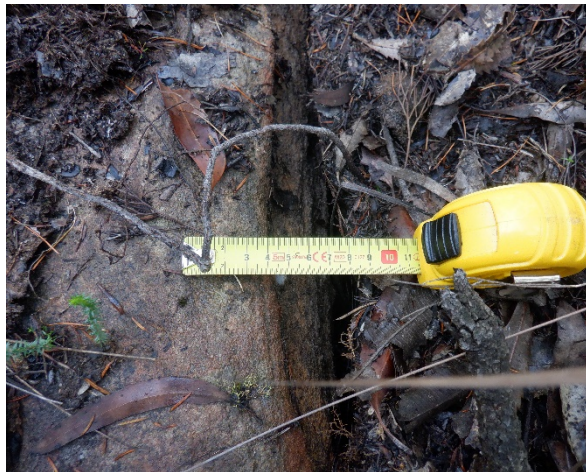
Photo 70: DA3B_LW17_017 – width of rock displacement. Taken on 25/05/2021.
