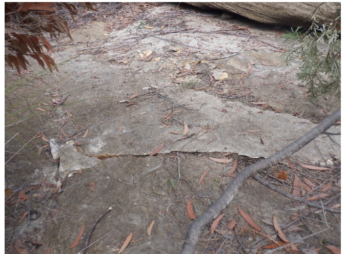
Photo 25: DA3B_LW17_012, additional smaller fracture and uplift. Taken on 10/09/2021.
