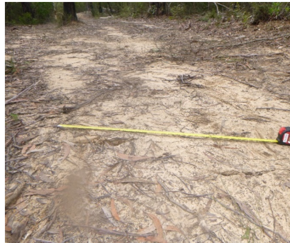
Photo 116: DA3B_LW17_028- soil cracking on access track. Taken on 26/07/2021.
