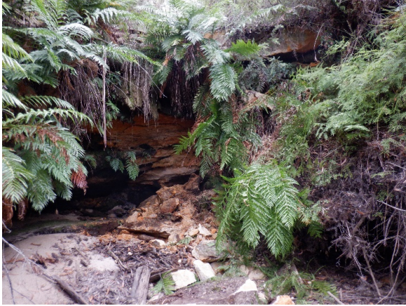
Photo 20: DA3B_LW17_003, rockfall to step as shown in previous update report. Taken on 10/03/2021.
