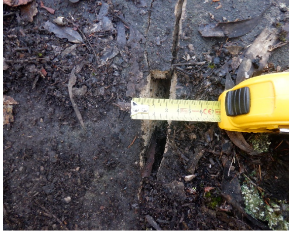
Photo 68: DA3B_LW17_016 – width of rock fracturing. Taken on 25/05/2021.
