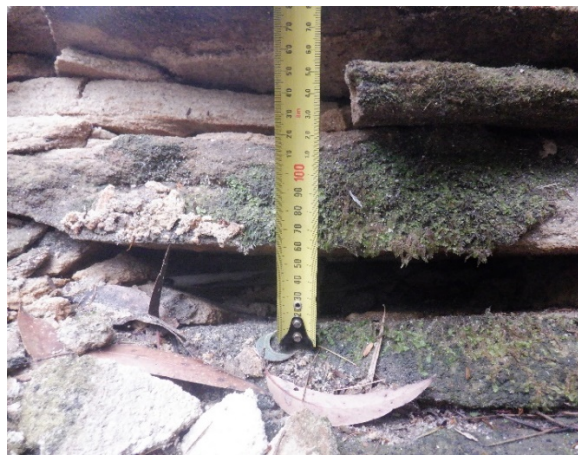
Photo 14: DA3B_LW17_006, looking at the width of the rock fracturing. Taken on 10/09/2021.
