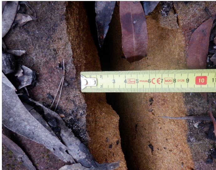
Photo 79: DA3B_LW17_023- showing width of fracture. Taken on 22/06/2021.
