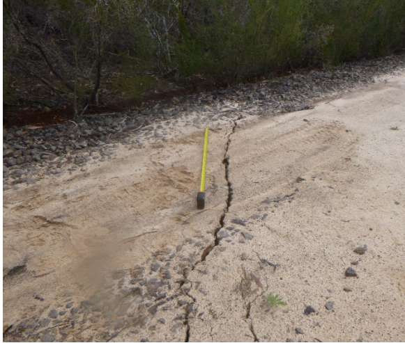
Photo 117: DA3B_LW17_029- soil cracking across rail corridor ballast. Taken on 26/07/2021.
