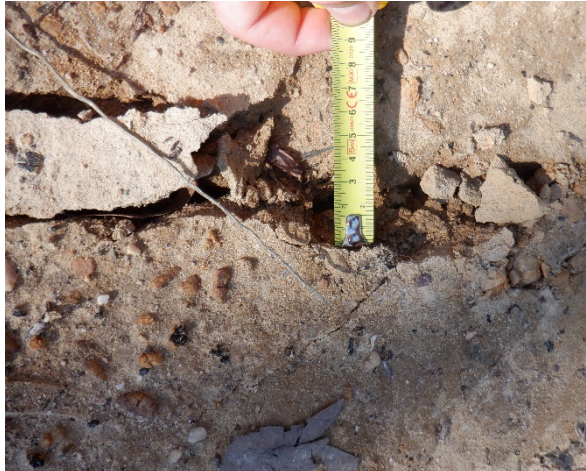
Photo 108: DA3B_LW17_015- showing width of soil crack on access track. Taken on 18/05/2021.
