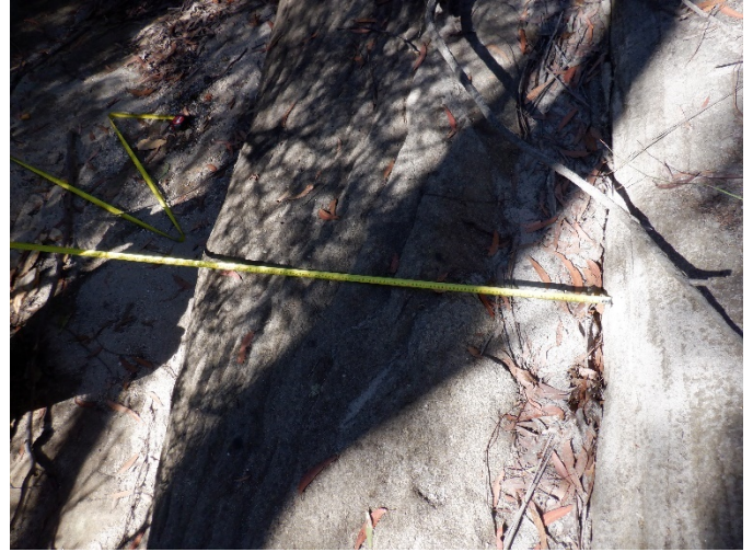
Photo 23: DA3B_LW17_012, looking at width of displaced slab. Taken on 13/04/2021.
