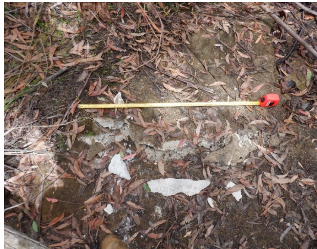
Photo 6: DA3B_LW17_001, looking at a section of rock fracturing, uplift and fragmentation. Taken on 5/02/2021.
