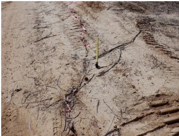
Photo 123: DA3B_LW17_014- Impact has been partially remediated. Some smaller cracks remain. Taken on 16/09/2021.
