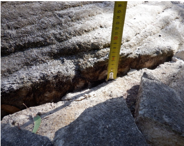
Photo 24: DA3B_LW17_012, looking at level of displacement fracture to step. Taken on 13/04/2021.
