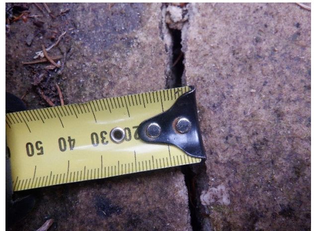
Photo 30: DA3B_LW17_034, showing the width of rock fracturing. Taken 10/9/2021.
