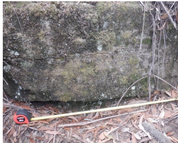
Photo 62: DA3B_LW17_010, fracturing along step. Taken on 10/09/2021.
