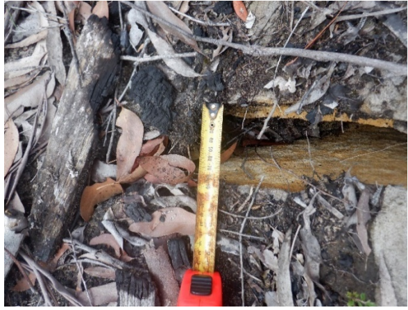
Photo 103: DA3B_LW17_040, showing width of the rock fracturing. Taken 21/10/2021
