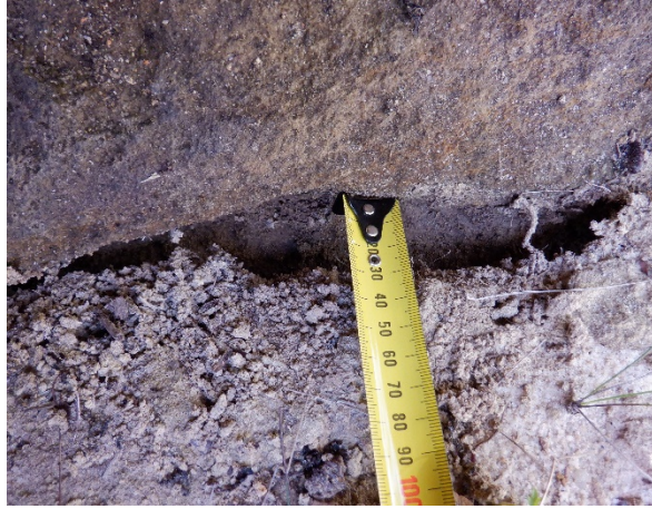
Photo 85: DA3B_LW17_032, showing the width of the displacement. Taken on 17/08/2021.
