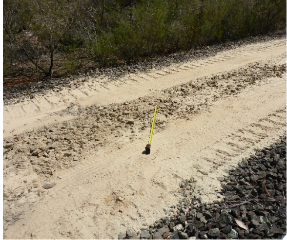
Photo 118: DA3B_LW17_029- Remediated soil cracking across rail corridor ballast. Taken on 22/09/2021.
