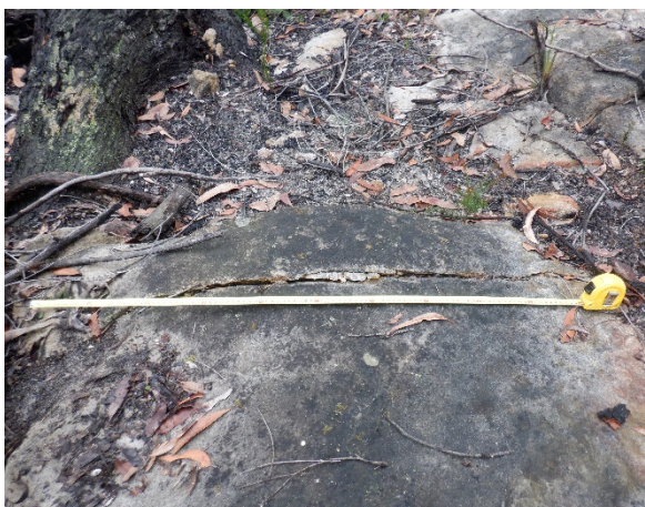
Photo 76: DA3B_LW17_022, looking at length of fracture. Taken on 22/06/2021.
