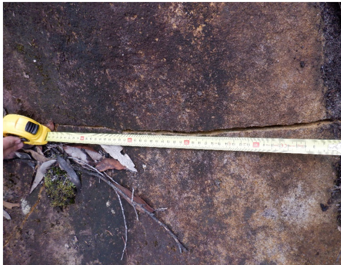
Photo 81: DA3B_LW17_023- looking at smaller fracture. Taken on 22/06/2021
