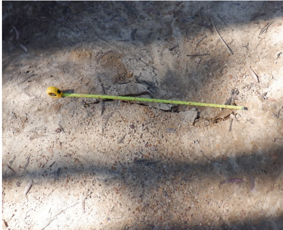
Photo 107: DA3B_LW17_015- soil crack on access track. Taken on 18/05/2021.
