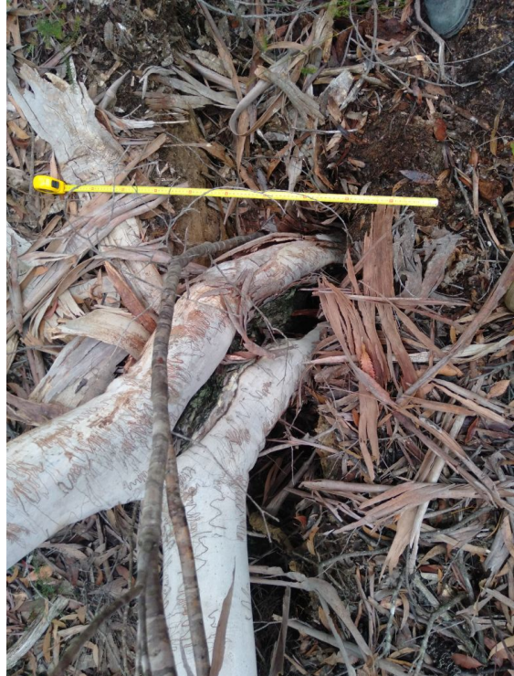
Photo 72: DA3B_LW17_019, looking at the maximum width of the soil cracking. Taken on 8/06/2021.
