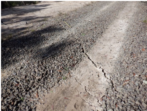
Photo 113: DA3B_LW17_26, cracking extending across railway corridor. Taken on 7/07/2021.
