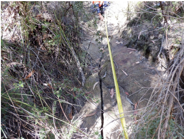
Photo 26: DA3B_LW17_013, fractures running along channel. Taken on 13/04/2021.
