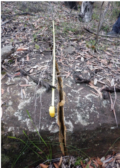
Photo 80: DA3B_LW17_023- looking fracture. Taken on 22/06/2021
