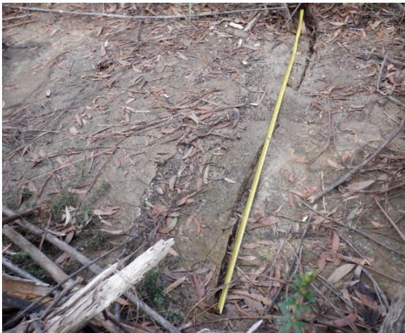
Photo 5: DA3B_LW17_001, looking at a section of rock fracturing. Taken on 10/09/2021.
