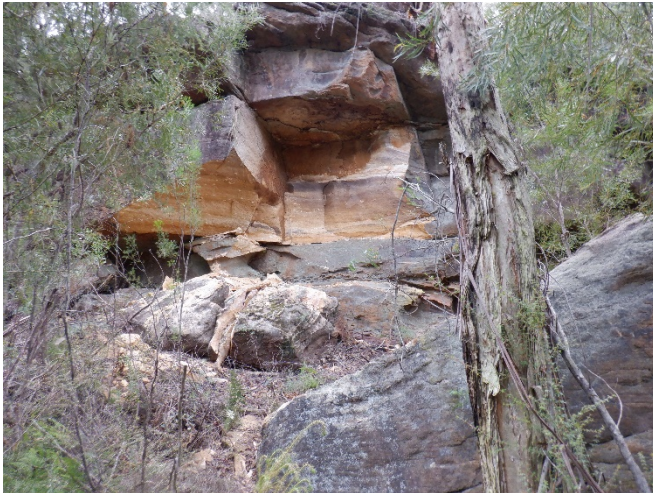
Photo 57: DA3B_LW17_009, looking at a section of rockfall. Taken on 10/03/2021.
