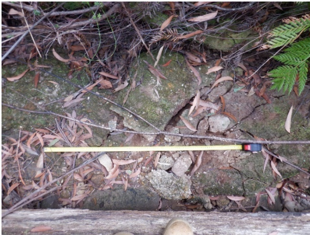
Photo 15: DA3B_LW17_006, looking at a section of soil cracking. Taken on 10/03/2021.
