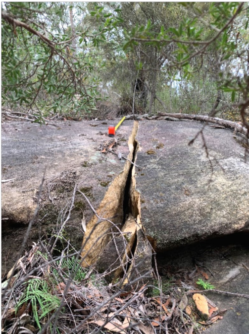
Photo 94: DA3B_LW17_037, looking at a section of rock fracturing. Taken 15/9/2021.
