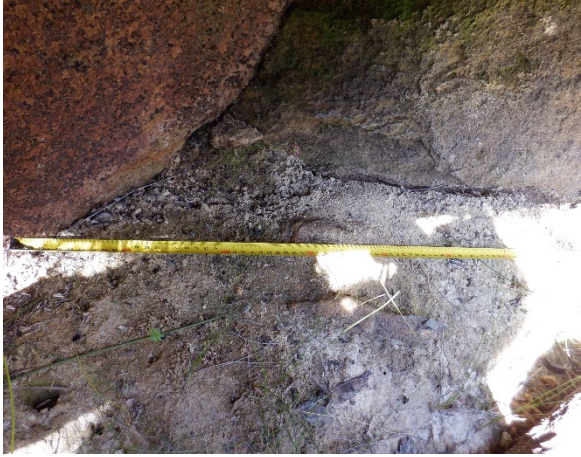
Photo 84: DA3B_LW17_032, showing the length of displacement. Taken on 17/08/2021.
