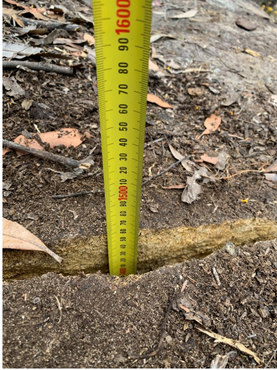
Photo 91: DA3B_LW17_036, Looking at a section of rock fracturing. Taken 15/9/2021
