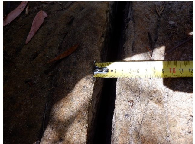
Photo 27: DA3B_LW17_013, looking at width of fracture. Taken on 13/04/2021.
