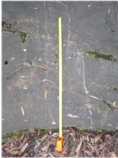
Photo 13: DA3B_LW16_018, looking at a section of rock fracturing. Taken on 16/06/2020.
