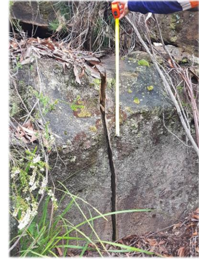
Photo 9: DA3B_LW16_012, looking at a section of rock fracturing. Taken on 28/04/2020.
