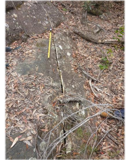
Photo 27: DA3B_LW16_048, looking at the length of rock fracturing. Taken on 30/11/2020.
