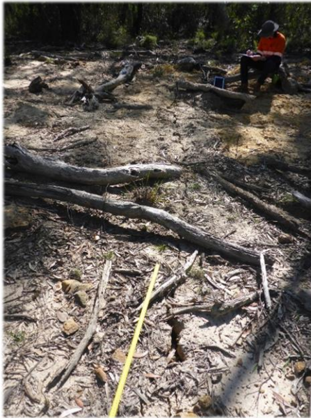
Photo 37: DA3B_LW16_005, soil cracking to access track between Lake Avon and FR6A . Taken on 22/04/2020.
