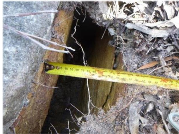
Photo 23: DA3B_LW16_044, looking at width of rock fracturing. Taken on 10/11/2020.
