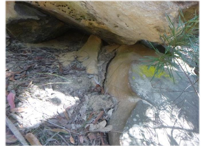
Photo 21: DA3B_LW16_035, looking at a section of displacement. Taken on 28/09/2020.
