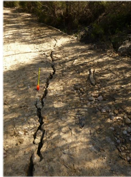
Photo 38: DA3B_LW16_013, soil cracking to access track between Lake Avon and FR6A . Taken on 12/05/2020.
