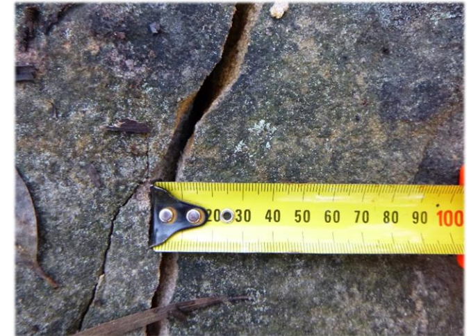
Photo 12: DA3B_LW16_017, looking at width of rock fracturing. Taken on 16/06/2020.
