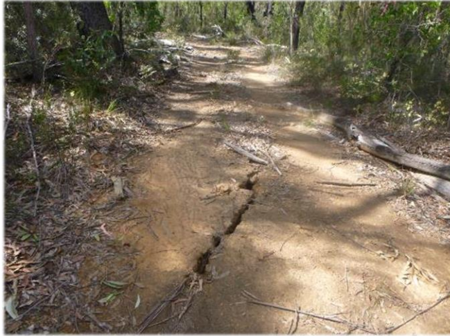
Photo 35: DA3B_LW16_027 , soil cracking across Fire Road 6P. Taken on 21/08/2020.
