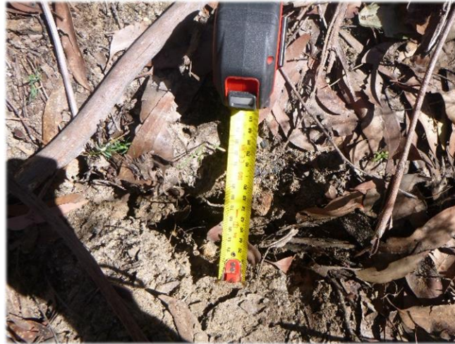
Photo 20: DA3B_LW16_032, looking at the width of soil cracking. Taken on 28/09/2020.
