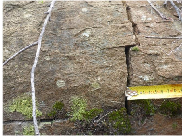
Photo 32: DA3B_LW15_002 , looking at a section of rock fracturing. Taken on 2/12/2020.
