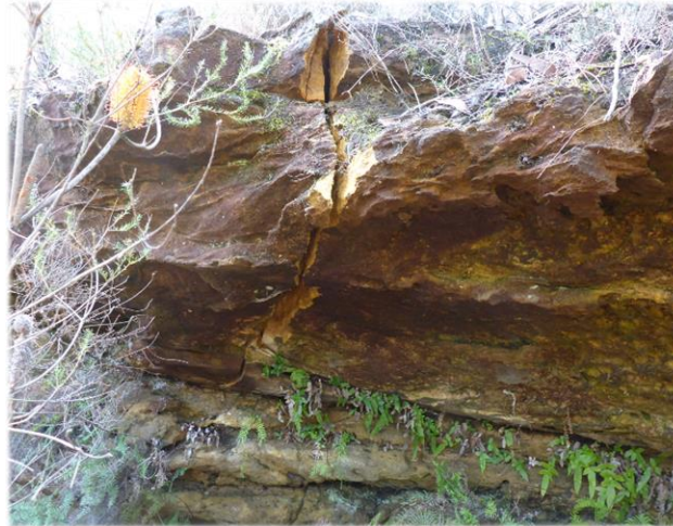
Photo 14: DA3B_LW16_021, looking at fracture on step. Taken on 30/06/2020.
