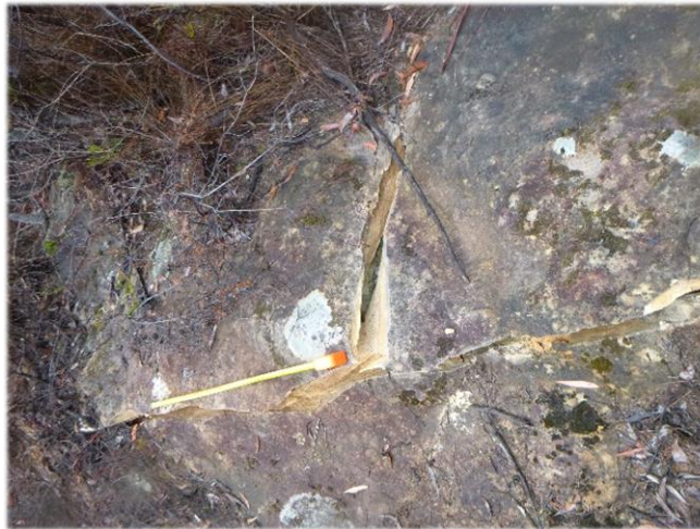
Photo 5: DA3B_LW14_019, looking at a section of rock fracturing and uplift. Taken on 9/09/2020.
