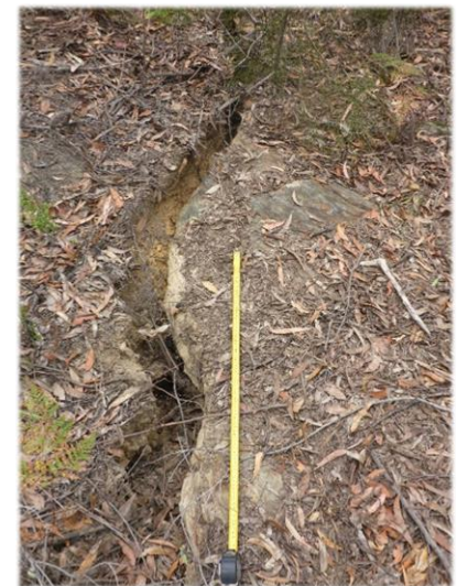
Photo 30: DA3B_LW16_051, looking at a section of soil cracking and rock fracturing. Taken on 30/11/2020.
