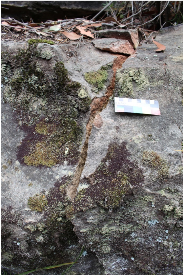
Plate 11: Close up of vertical cracking located at the base of the northern exterior of the shelter cavern area. Photo taken: 20 January 2021.
