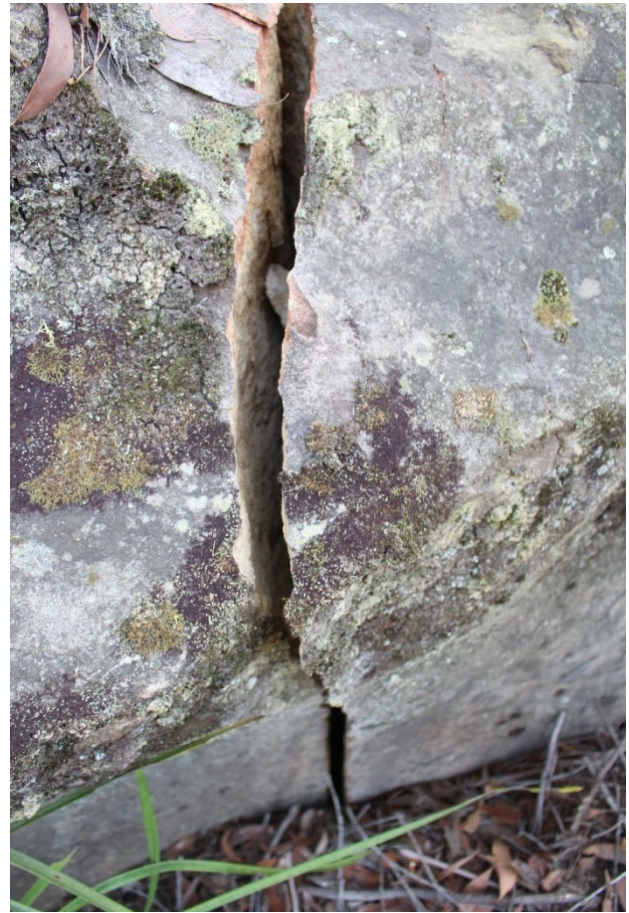
Plate 12: Close up of vertical cracking located at the base of the northern exterior of the shelter cavern area. Recorded by Niche (2020) for the Longwall 15 EoP. Photo taken: 15 April 2020.
