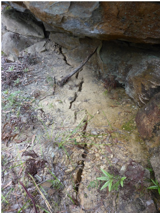
Photo 58: DA3B_LW16_029, looking at soil cracking. Taken on 25/11/2020.
