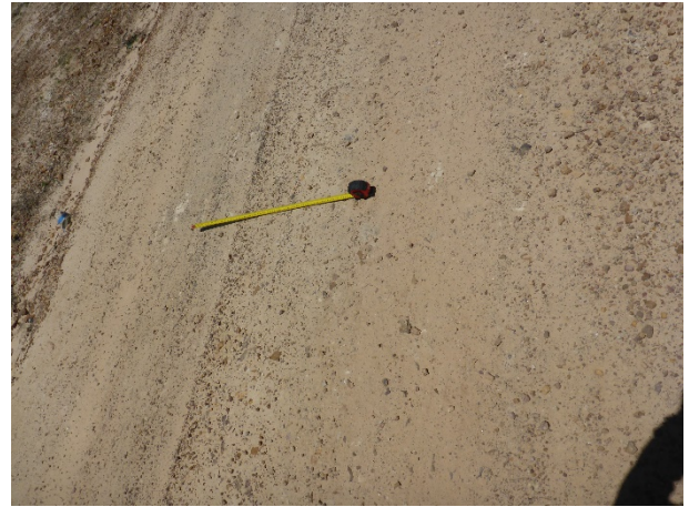
Photo 120: DA3B_LW16_020, soil cracking naturally remediated. Taken on 19/11/2020.
