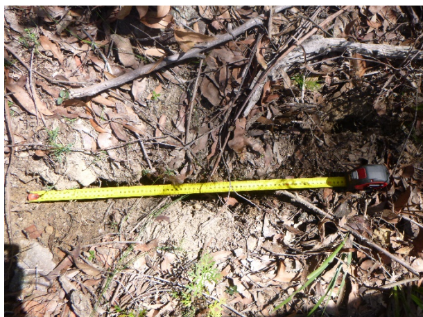
Photo 66: DA3B_LW16_032, looking at the length of soil cracking. Taken on 28/09/2020.
