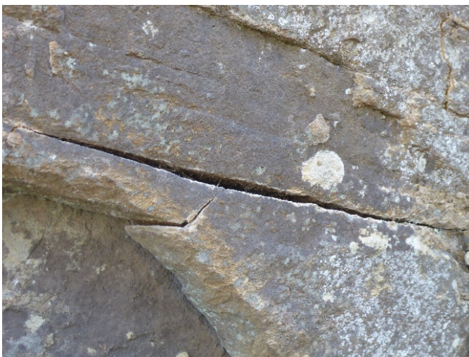
Photo 54: DA3B_LW16_026 , looking at a section of rock fracturing. Taken on 06/08/2020.
