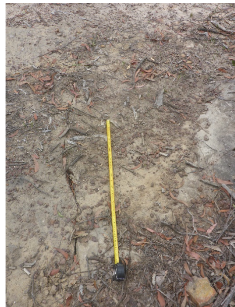
Photo 134: DA3B_LW16_040, no change to soil cracking. Taken on 30/11/2020.
