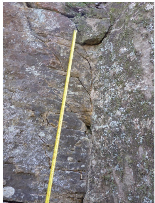
Photo 55: DA3B_LW16_026 , looking at a section of rock fracturing. Taken on 06/08/2020.
