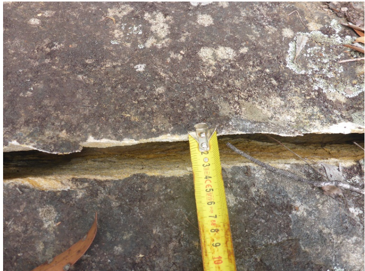
Photo 84: DA3B_LW16_048, looking at the width of rock fracturing. Taken on 30/11/2020.
