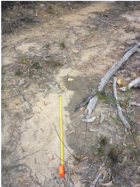
Photo 135: DA3B_LW16_041, soil cracking to access track east of Swamp 14. Taken on 7/10/2020.
