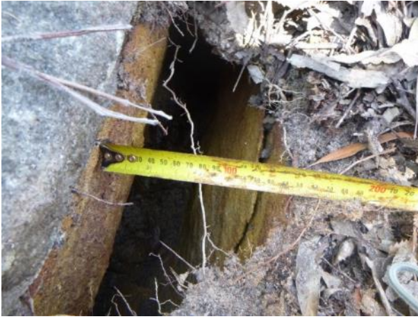
Photo 74: DA3B_LW16_044, looking at width of rock fracturing. Taken on 10/11/2020.
