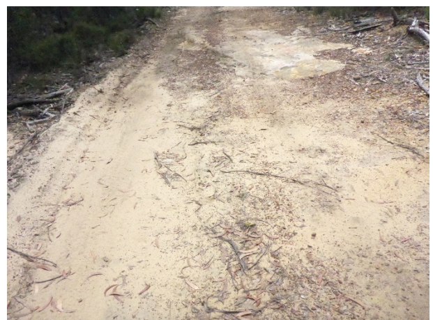
Photo 116: DA3B_LW16_014, soil cracking naturally remediated. Taken on 19/11/2020.
