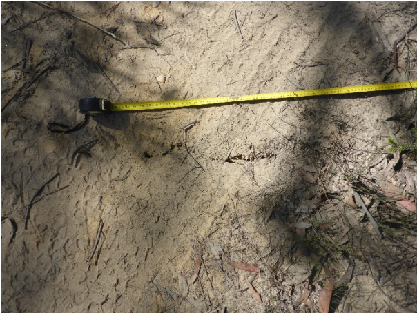
Photo 107: DA3B_LW16_006, soil cracking on access track between Lake Avon and FR6A. Taken on 22/04/2020.
