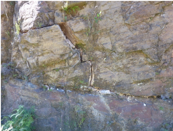
Photo 47: DA3B_LW16_022, fracturing down face of cut-through. Taken on 6/08/2020.
