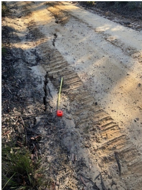
Photo 149: DA3B_LW16_019, looking at length of soil cracking on FR6A. Taken on 23/06/2020.
