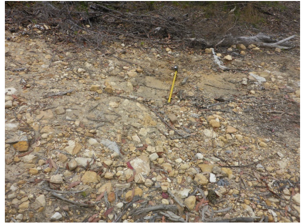
Photo 126: DA3B_LW16_033, soil cracking naturally remediated. Taken on 30/11/2020.
