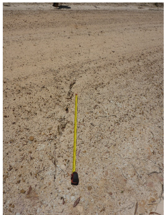
Photo 122: DA3B_LW16_023, cracking partly naturally remediated. Taken on 7/07/2020.
