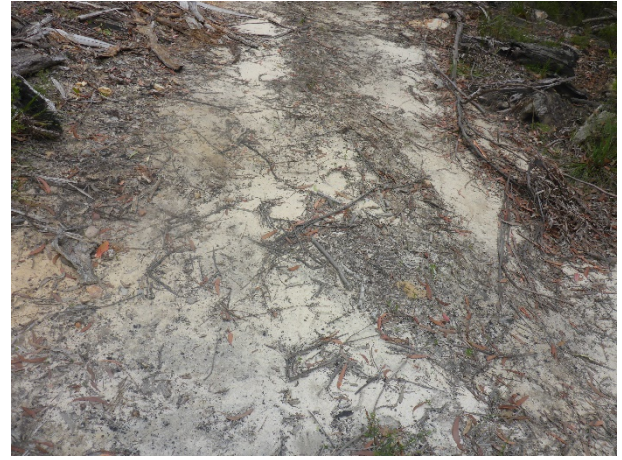
Photo 142: DA3B_LW16_043, soil cracking naturally remediated. Taken on 30/11/2020.
