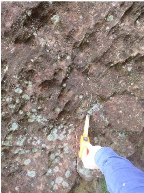
Photo 79: DA3B_LW16_046, looking at the rock fracture. Taken on 25/11/2020.
