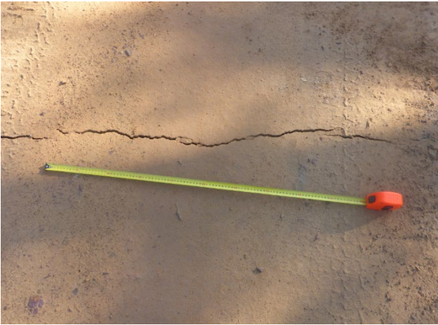
Photo 119: DA3B_LW16_020, soil cracking on FR6A. Taken on 30/06/2020.
