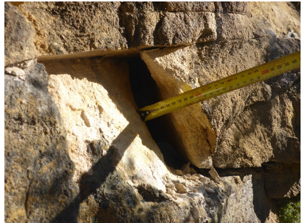
Photo 48: DA3B_LW16_022, looking at a section of rock fracturing. Taken on 6/08/2020.
