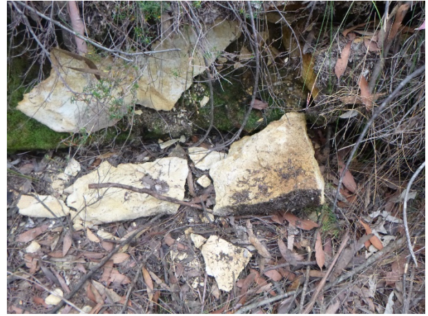
Photo 27: DA3B_LW16_011, an overview of the rockfall. Taken on 27/04/2020.
