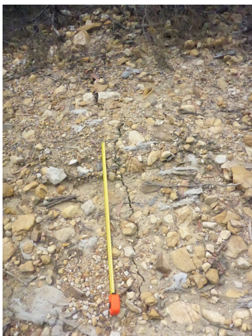
Photo 139: DA3B_LW16_042, soil cracking to access track east of Swamp 14. Taken on 7/10/2020.
