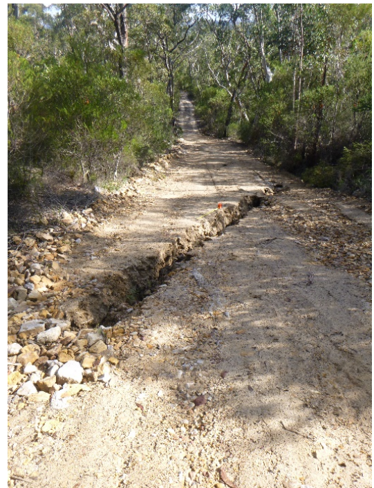
Photo 146: DA3B_LW16_013, soil cracking following a rainfall event. Taken on 28/05/2020.
