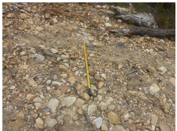
Photo 140: DA3B_LW16_042, soil cracking naturally remediated. Taken on 30/11/2020.
