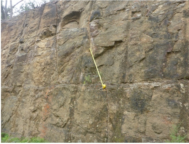
Photo 45: DA3B_LW16_022, fracturing down face of cut-through. Taken on 7/07/2020.
