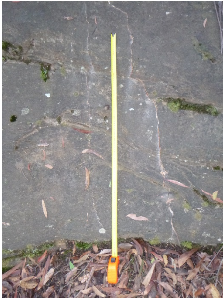
Photo 39: DA3B_LW16_018, looking at a section of rock fracturing. Taken on 16/06/2020.
