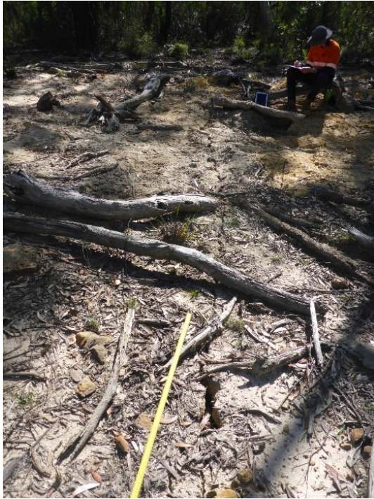
Photo 143: DA3B_LW16_005, soil cracking to access track between Lake Avon and FR6A. Taken on 22/04/2020.
