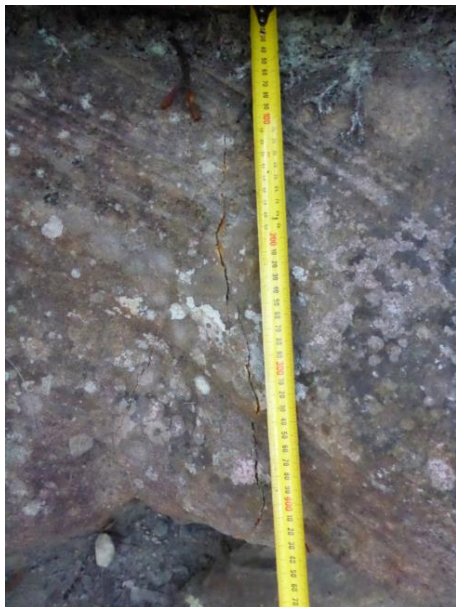
Photo 97: DA3B_LW15_026, looking at a section of rock fracturing. Taken on 24/08/2020.
