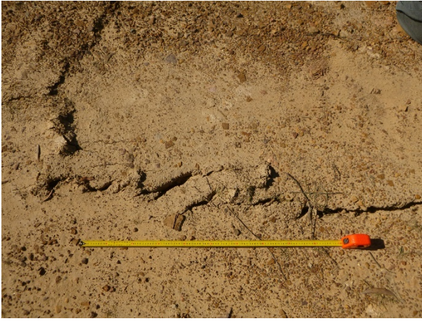
Photo 117: DA3B_LW15_008 (Update), soil cracking and uplift on FR6A. Taken on 12/05/2020.
