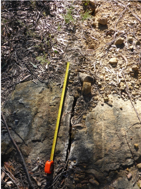
Photo 49: DA3B_LW16_024, looking at a section of rock fracturing. Taken on 06/08/2020.
