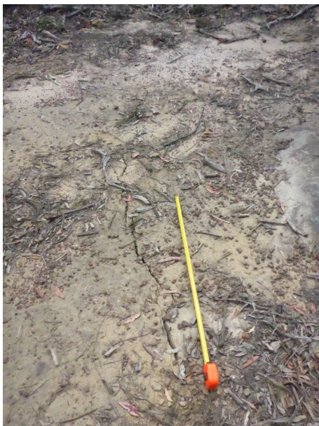
Photo 133: DA3B_LW16_040, soil cracking to access track east of Swamp 14. Taken on 7/10/2020.
