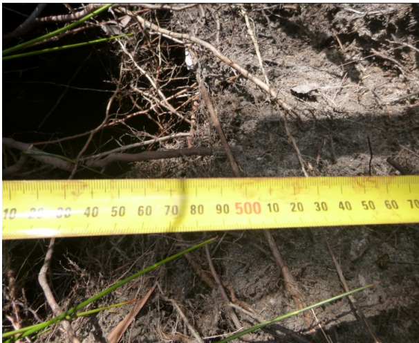
Photo 62: DA3B_LW16_030, looking at width of localised erosion. Taken on 31/08/2020.
