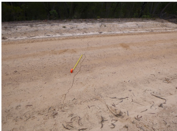
Photo 121: DA3B_LW16_023, cracking across Fire Road 6A. Taken on 7/07/2020.
