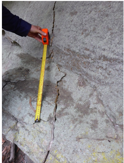
Photo 59: DA3B_LW16_029, looking at rock fracturing. Taken on 25/11/2020.
