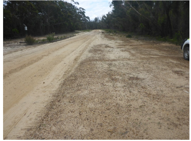
Photo 118: DA3B_LW15_008 (Update), soil cracking and uplift naturally remediated. Taken on 24/11/2020.
