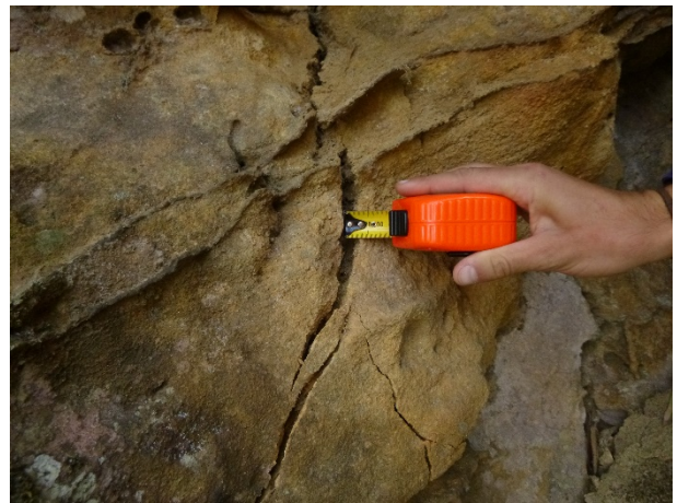
Photo 32: DA3B_LW16_015, looking at the width of rock fracturing. Taken on 15/05/2020.
