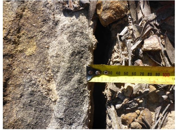
Photo 50: DA3B_LW16_024, looking at the width of rock fracturing. Taken on 06/08/2020.
