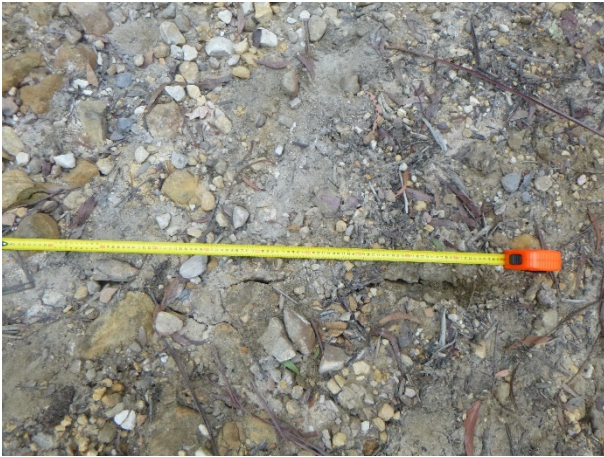
Photo 101: DA3B_LW16_002, soil cracking on access track between Lake Avon and FR6A. Taken on 16/04/2020.
