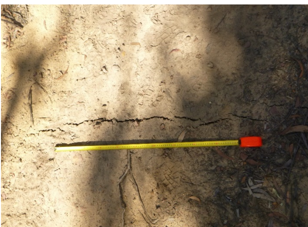
Photo 115: DA3B_LW16_014, soil cracking on access track between Lake Avon and FR6A. Taken on 12/05/2020.
