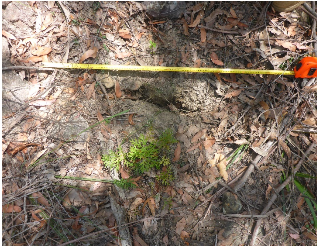
Photo 92: DA3B_LW16_052, looking at a section of soil cracking. Taken on 1/12/2020.
