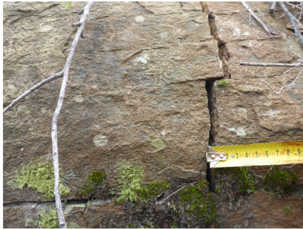
Photo 96: DA3B_LW15_002, looking at a section of rock fracturing. Taken on 2/12/2020.
