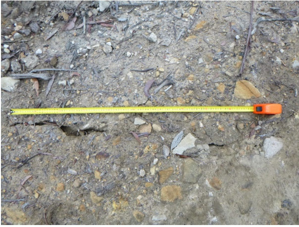
Photo 99: DA3B_LW16_001, soil cracking on access track between Lake Avon and FR6A. Taken on 16/04/2020.
