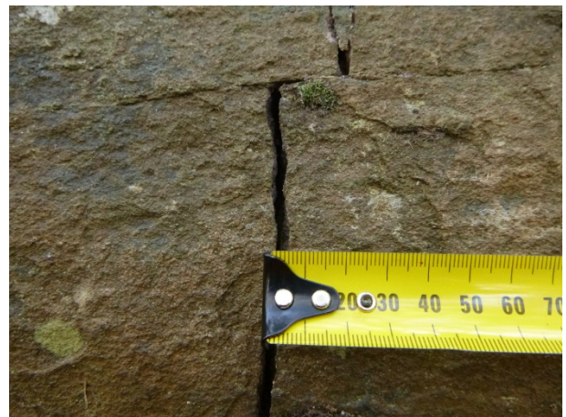
Photo 95: DA3B_LW15_002, looking at the width of rock fracturing. Taken on 05/05/2020.
