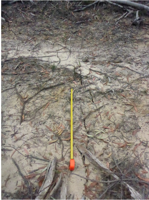
Photo 141: DA3B_LW16_043, soil cracking to access track east of Swamp 14. Taken on 7/10/2020.
