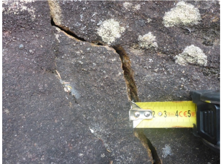
Photo 82: DA3B_LW16_047, looking at the width of the rock fracturing. Taken on 30/11/2020.
