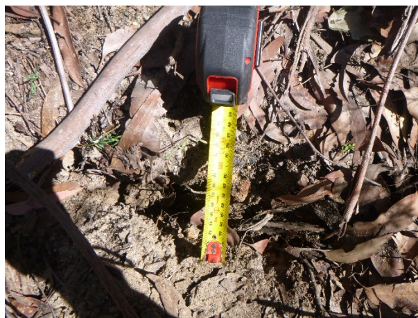
Photo 67: DA3B_LW16_032, looking at the width of soil cracking. Taken on 28/09/2020.
