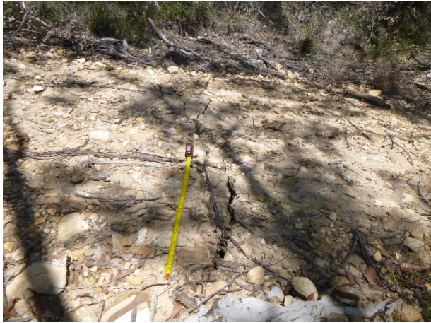
Photo 125: DA3B_LW16_033, section of soil cracking on access track parallel to WC15. Taken on 28/09/2020.
