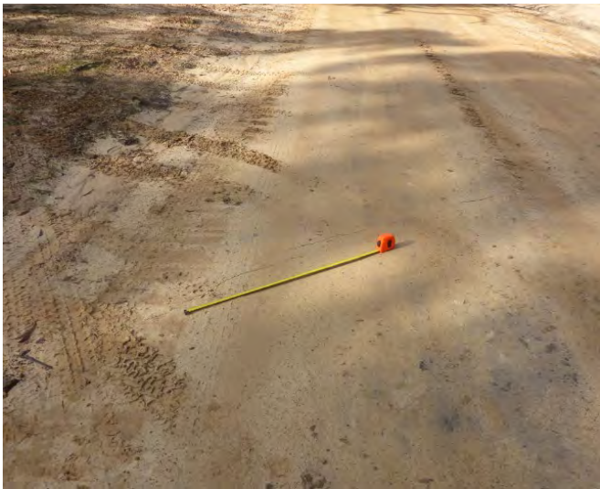
Photo 1: DA3B_LW16_020 , looking at the cracking across fire road. Taken on 30/06/2020.
