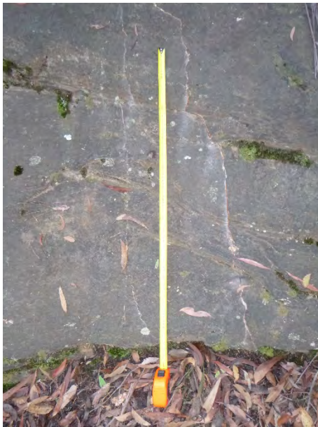
Photo 3: DA3B_LW16_018, looking at a section of rock fracturing. Taken on 16/06/2020.
