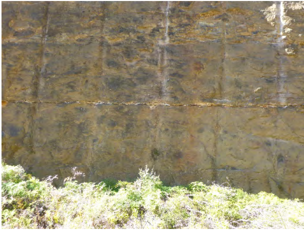
Photo 3: DA3B_LW16_022, looking at a section of rock fracturing. Taken on 6/08/2020.
