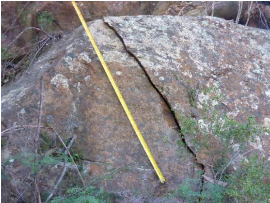
Photo 13: DA3B_LW16_025, looking at a section of rock fracturing. Taken on 6/08/2020.
