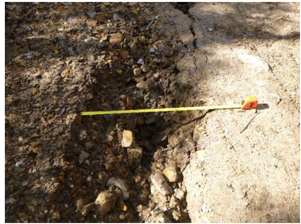
Photo 2: DA3B_LW16_013, looking at the width of surface erosion. Taken on 28/05/2020.
