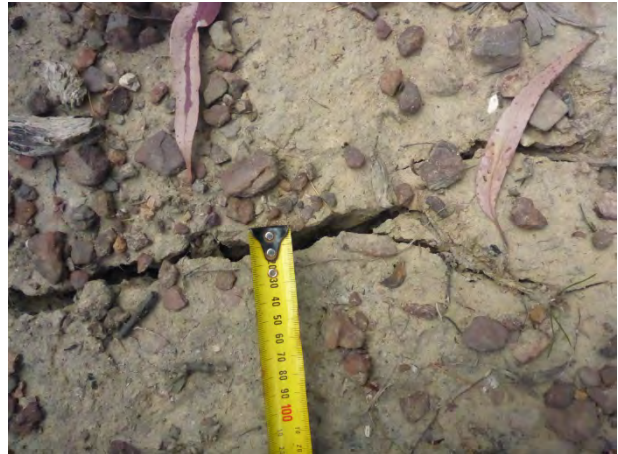
Photo 4: DA3B_LW16_040 - soil cracking to access track. Taken on 7/10/2020.
