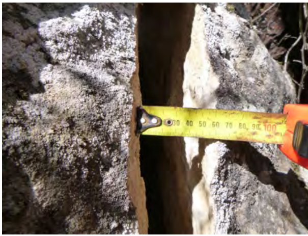
Photo 7: DA3B_LW16_045, looking at width of rock fracturing. Taken on 10/11/2020.
