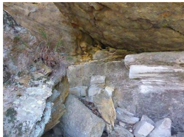
Photo 2: DA3B_LW16_031 , looking at the rockfall. Taken on 28/09/2020.
