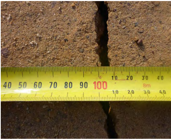
Photo 3: DA3B_LW16_020 , looking at width of cracking across fire road. Taken on 30/06/2020.
