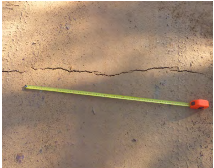
Photo 2: DA3B_LW16_020 , looking at the cracking across fire road. Taken on 30/06/2020.
