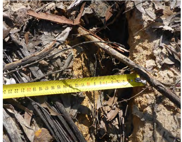
Photo 4: DA3B_LW16_004, looking at the width of the soil cracking. Taken on 22/04/2020.
