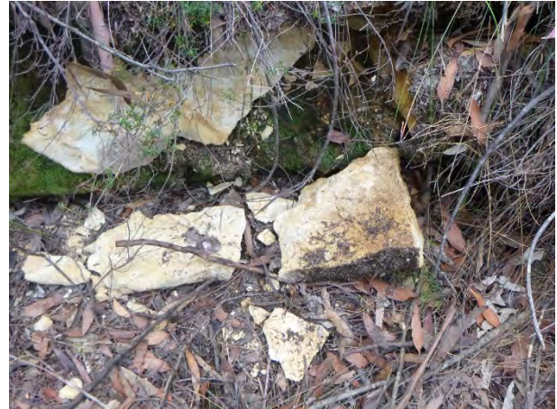
Photo 9: DA3B_LW16_011, overview of the rockfall. Taken on 27/04/2020.
