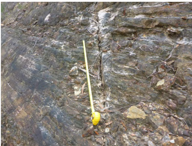
Photo 7: DA3B_LW16_022- fracturing down face of cut-through. Taken on 7/07/2020.
