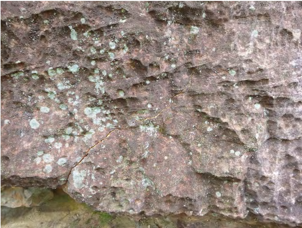
Photo 2: DA3B_LW16_046, looking at the rock fracture. Taken on 25/11/2020.
