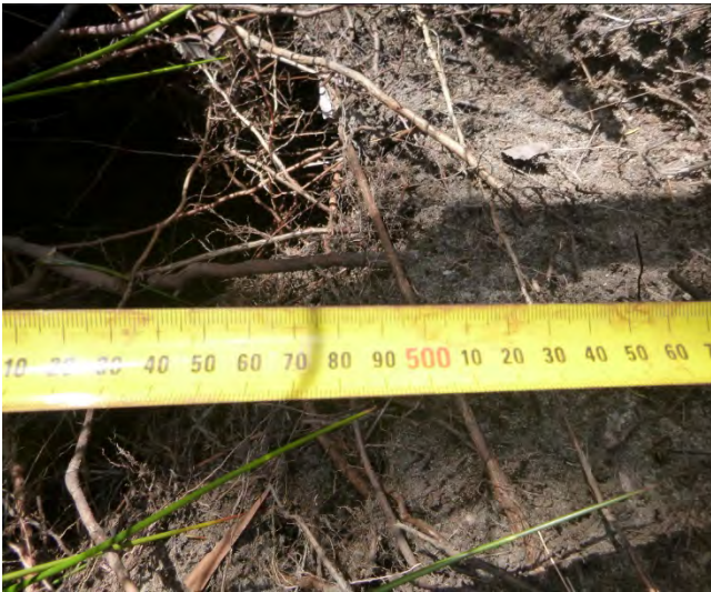
Photo 10: DA3B_LW16_030- localised erosion, looking at width. Taken on 31/08/2020.
