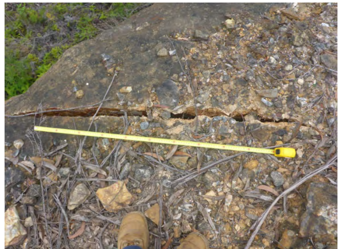
Photo 2: DA3B_LW16_022- fracturing fracture to top of cut-through. Taken on 7/07/2020.
