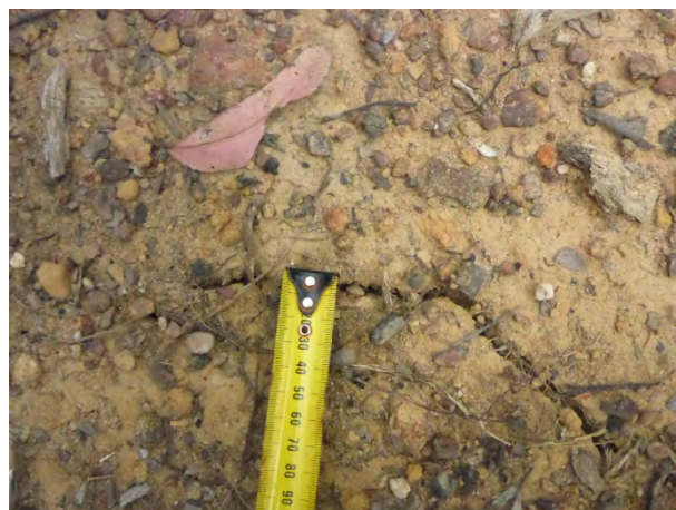
Photo 2: DA3B_LW16_039 soil cracking to access track. Taken on 7/10/2020.
