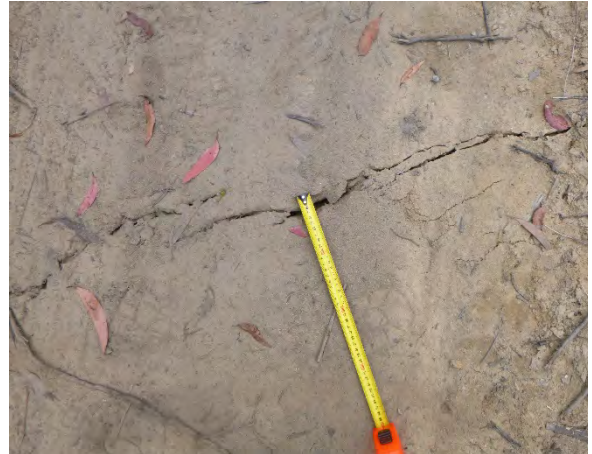
Photo 2: DA3B_LW16_008, looking at the width of the soil cracking. Taken on 27/04/2020.
