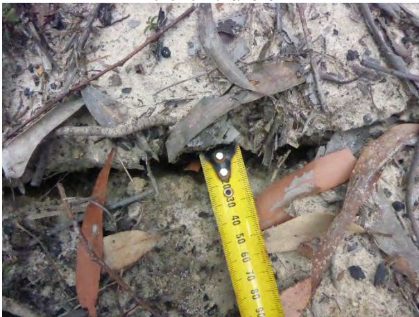
Photo 15: DA3B_LW16_043- soil cracking to access track. Taken on 7/10/2020.
