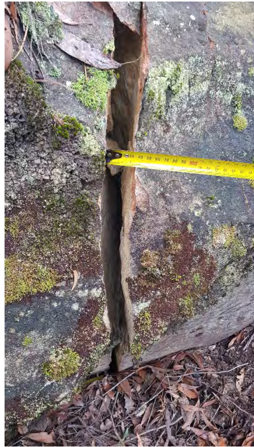
Photo 11: DA3B_LW16_012, looking at the maximum width of the rock fracture. Taken on 28/04/2020.
