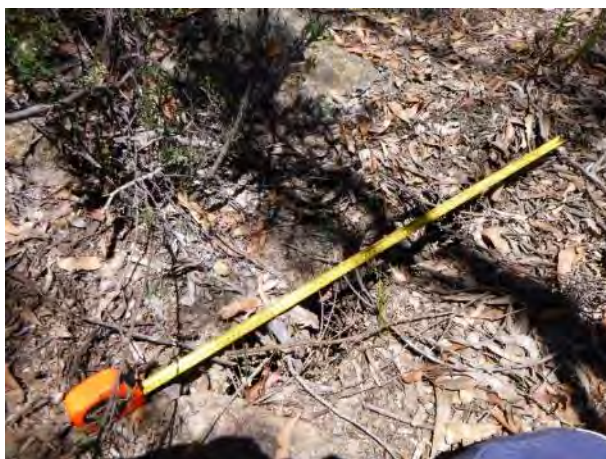
Photo 1: DA3B_LW16_044, looking at length of soil cracking. Crack runs in orientation of tape measure. Taken on 10/11/2020.
