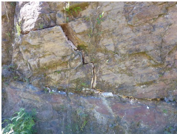
Photo 1: DA3B_LW16_022 , looking at a section of rock fracturing. Taken on 6/08/2020.
