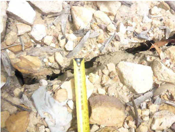
Photo 11: DA3B_LW16_042- soil cracking to access track. Taken on 7/10/2020.
