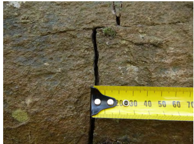
Photo 7: DA3B_LW15_002, looking at the width of soil cracking. Taken on 05/05/2020.
