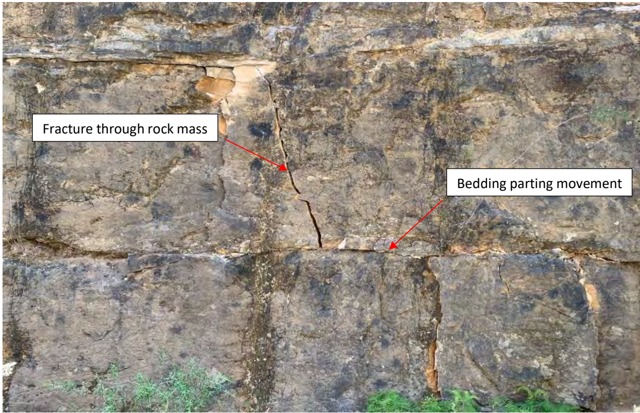
Figure 6 New fracturing through rock mass between bedding parting displacement (south west facing cut)
