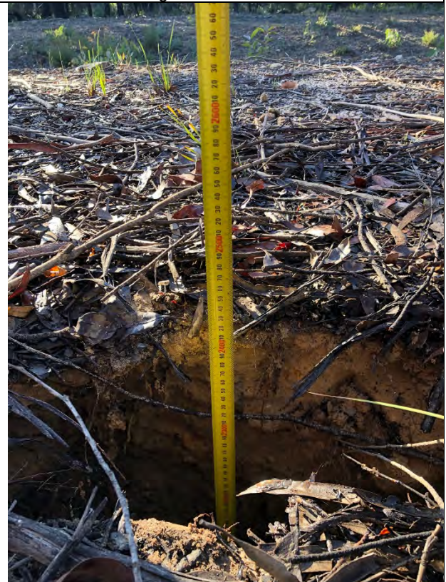
Photo 4: DA3B_LW16_019, looking at depth of cracking. Taken on 23/06/2020.
