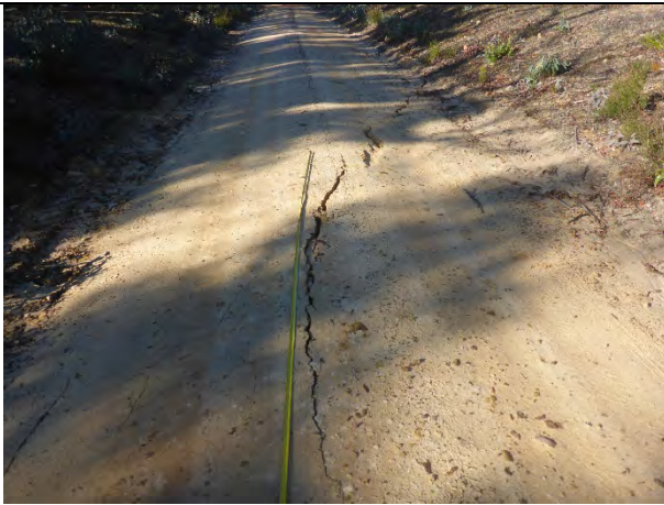
Photo 1: DA3B_LW16_019, looking at the length of initial cracking. Taken on 19/06/2020.
