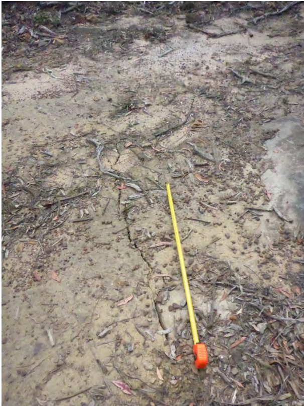
Photo 3: DA3B_LW16_040 - soil cracking to access track. Taken on 7/10/2020.
