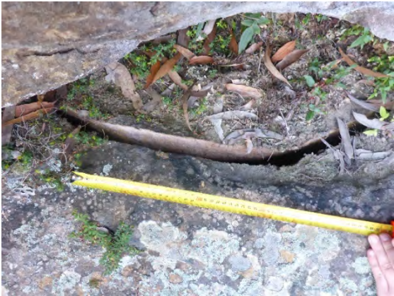
Photo 14: DA3B_LW16_025, looking at a section of rock fracturing. Taken on 6/08/2020.
