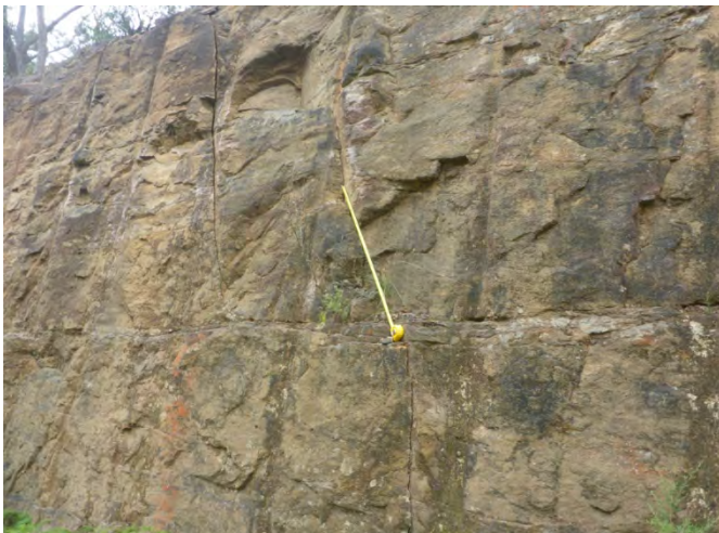
Photo 1: DA3B_LW16_022- fracturing down face of cut-through. Taken on 7/07/2020.
