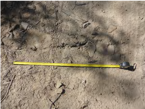
Photo 8: DA3B_LW16_007, looking at the soil cracking. Taken on 22/04/2020.
