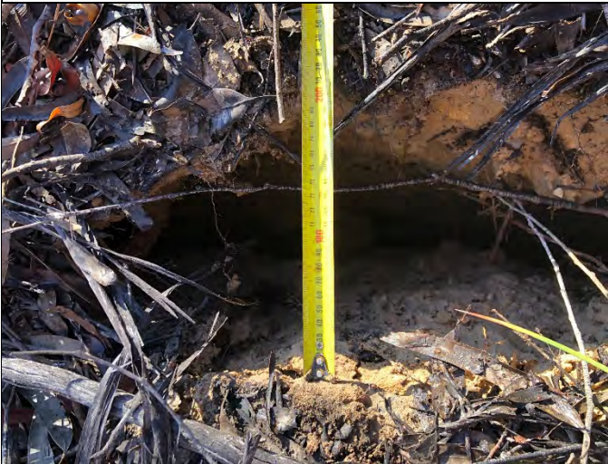
Photo 3: DA3B_LW16_019, looking at width of cracking. Taken on 23/06/2020.
