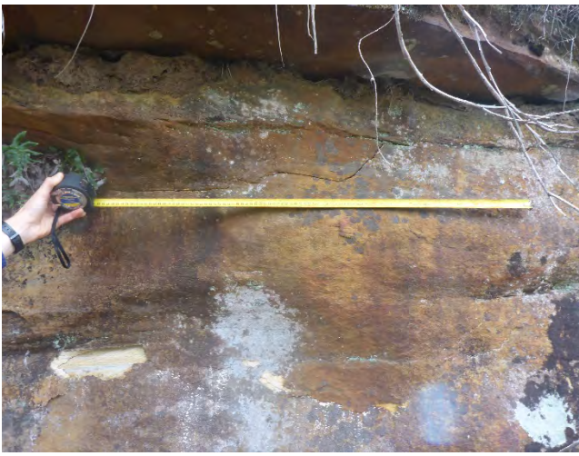
Photo 5: DA3B_LW16_049 , looking at a section of rock fracturing. Taken on 30/11/2020.
