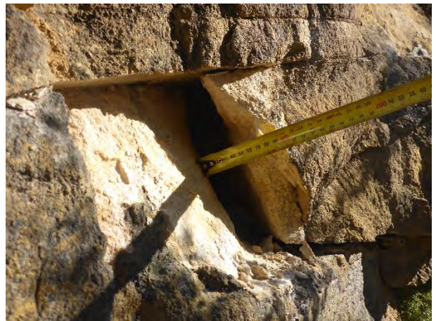
Photo 8: DA3B_LW16_022, looking at a section of rock fracturing. Taken on 6/08/2020.
