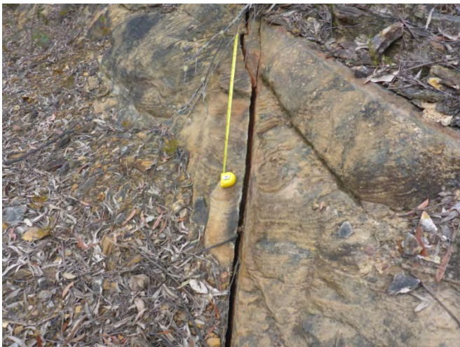
Photo 5: DA3B_LW16_022- fracturing down face of cut-through. Taken on 7/07/2020.
