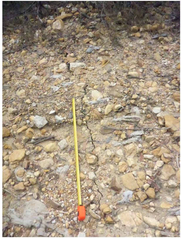
Photo 10: DA3B_LW16_042- soil cracking to access track. Taken on 7/10/2020.
