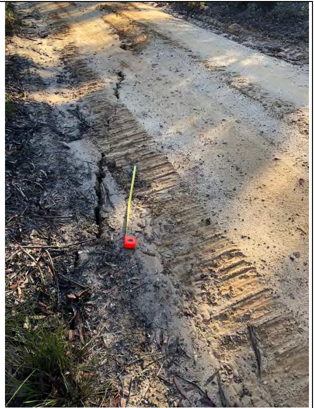
Photo 2: DA3B_LW16_019, looking at width of rock fracturing. Taken on 23/06/2020.
