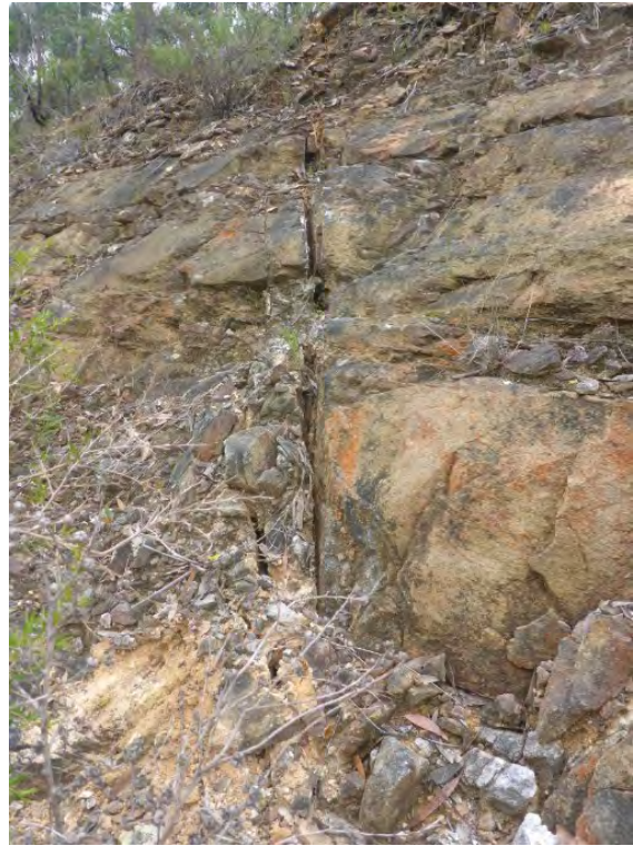
Photo 4: DA3B_LW16_022- fracturing down face of cut-through. Taken on 7/07/2020.
