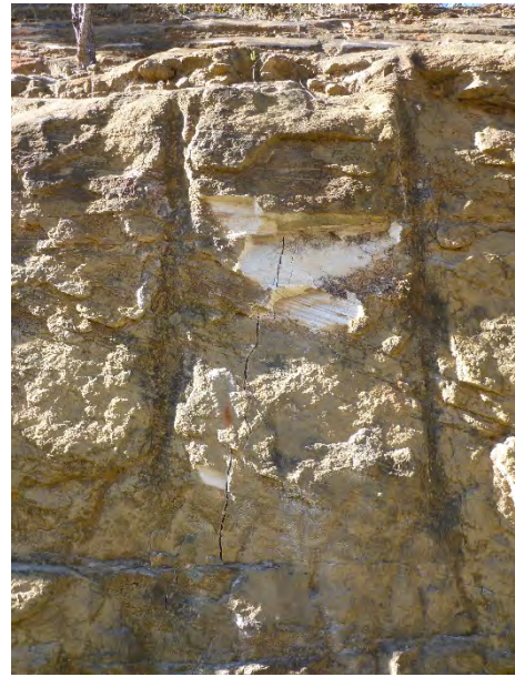
Photo 6: DA3B_LW16_022, looking at a section of rock fracturing and rockfall. Taken on 6/08/2020.
