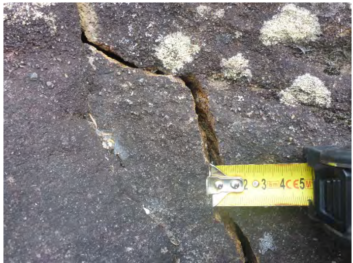
Photo 2: DA3B_LW16_047 , looking at the width of the rock fracturing. Taken on 30/11/2020.
