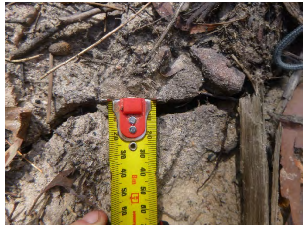
Photo 13: DA3B_LW16_037, looking at the width of soil cracking. Taken on 28/09/2020.
