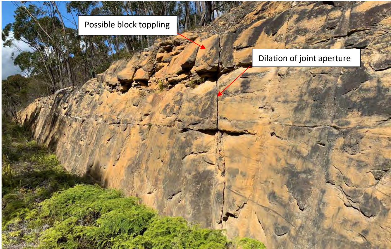
Figure 4 Dilation along dominant joint set (looking south)
