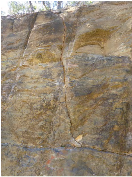
Photo 5: DA3B_LW16_022, looking at a section of rock fracturing. Taken on 6/08/2020.
