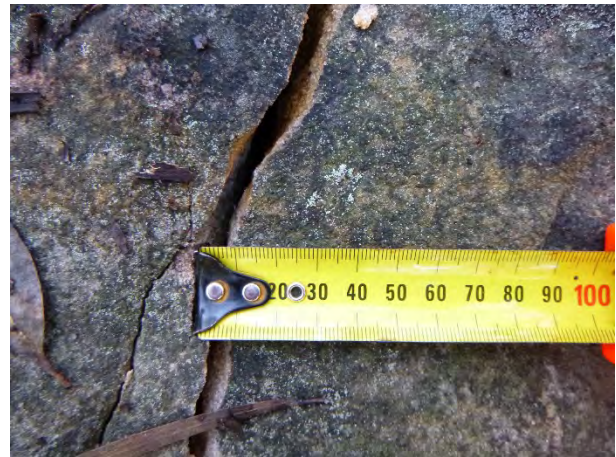
Photo 2: DA3B_LW16_017 , looking at width of rock fracturing. Taken on 16/06/2020.
