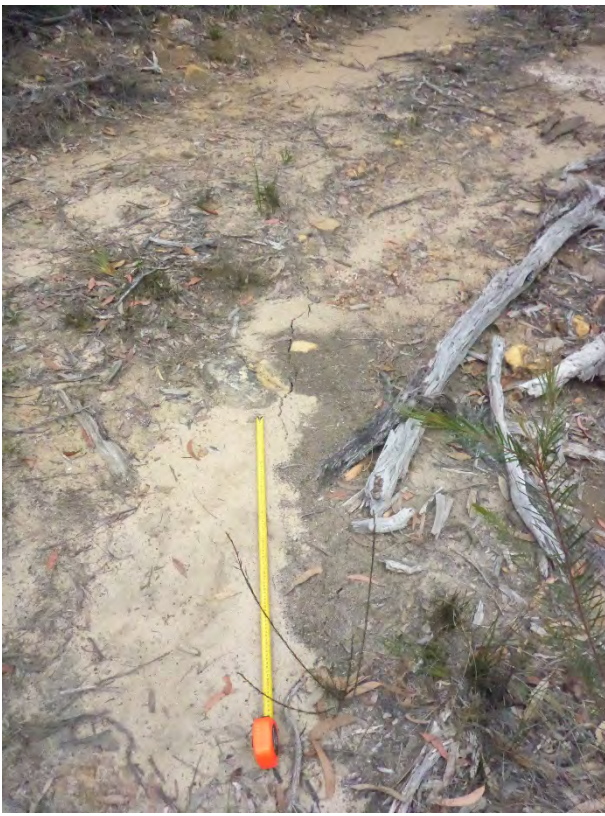
Photo 5: DA3B_LW16_041- soil cracking to access track. Taken on 7/10/2020.
