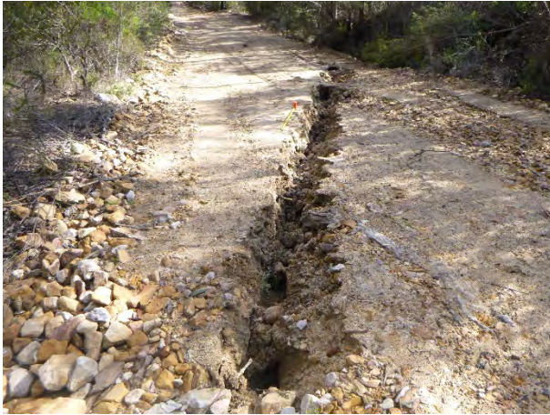
Photo 3: DA3B_LW16_013, looking at a section of soil cracking. Taken on 28/05/2020.
