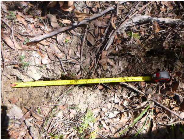
Photo 3: DA3B_LW16_032, looking at the length of soil cracking. Taken 28/09/2020.
