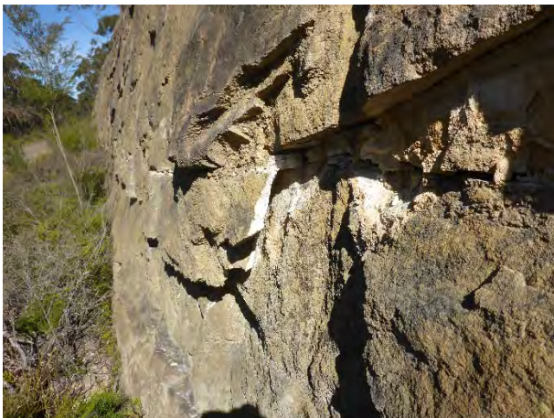
Photo 7: DA3B_LW16_022, looking at a section of rock fracturing. Taken on 6/08/2020.
