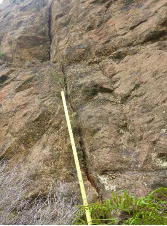
Photo 3: DA3B_LW16_022- fracturing down face of cut-through. Taken on 7/07/2020.
