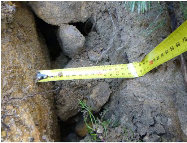
Photo 1: DA3B_LW16_013, looking at the width of soil cracking. Taken on 28/05/2020.
