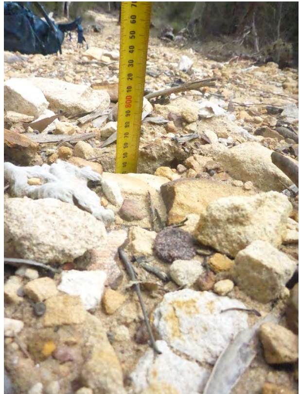
Photo 12: DA3B_LW16_042- depth measurement of soil cracking. Taken on 7/10/2020.
