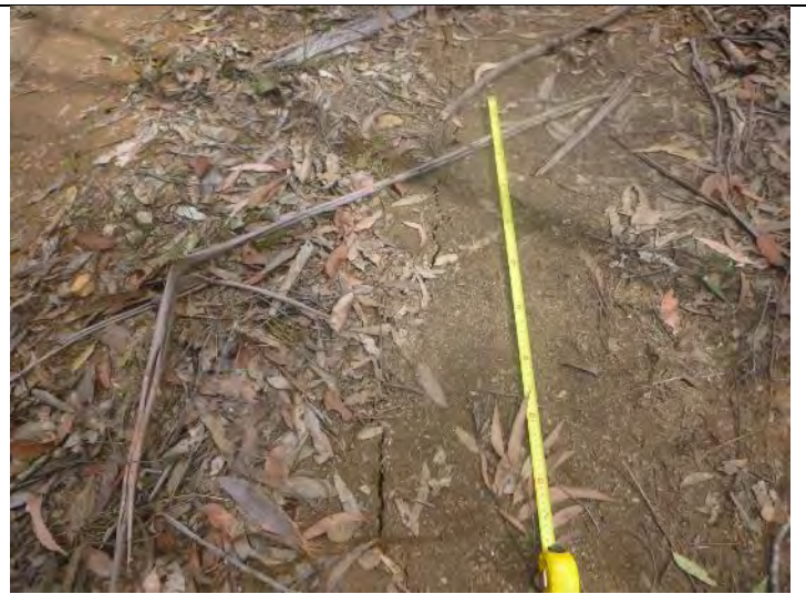
Photo 4: DA3B_LW16_027, showing narrower section of cracking. Taken on 21/08/2020.
