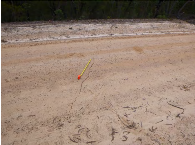
Photo 8: DA3B_LW16_023- cracking across Fire Road 6A. Taken on 7/07/2020.
