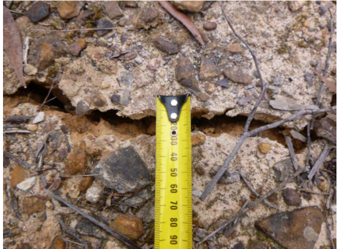
Photo 9: DA3B_LW16_023- cracking adjacent to Fire Road 6A. Taken on 7/07/2020.
