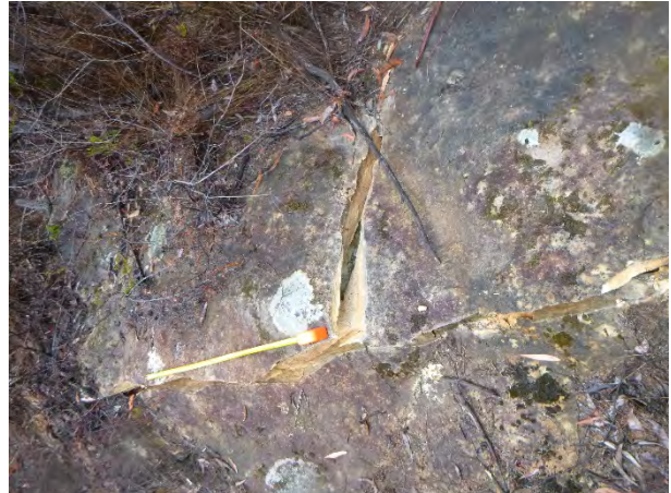
Photo 8: DA3B_LW14_019, looking at a section of rock fracturing and uplift. Taken on 9/09/2020.
