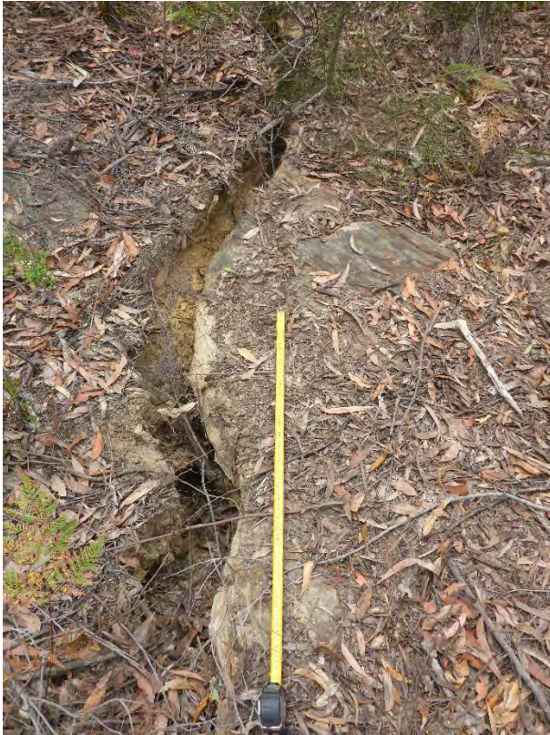
Photo 9: DA3B_LW16_051, looking at a section of soil cracking and rock fracturing. Taken on 30/11/2020.
