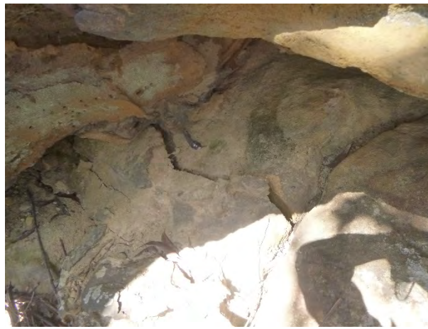
Photo 11: DA3B_LW16_036, looking at a section of rock fracturing. Taken 28/09/2020.
