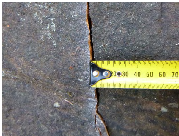
Photo 5: DA3B_LW16_018, looking at the width of rock fracturing. Taken on 16/06/2020.
