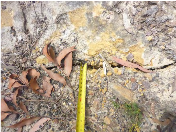
Photo 7: DA3B_LW16_041- soil cracking and displacement on access track. Taken on 7/10/2020.
