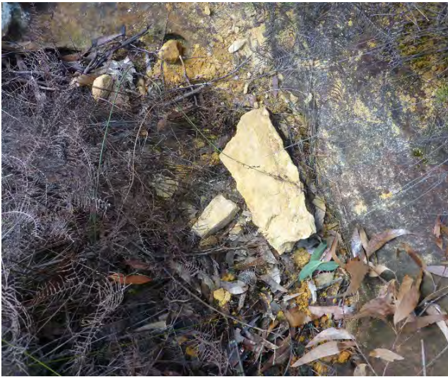
Photo 6: DA3B_LW16_021 , looking at small rock fragments fallen from step. Taken on 30/06/2020.
