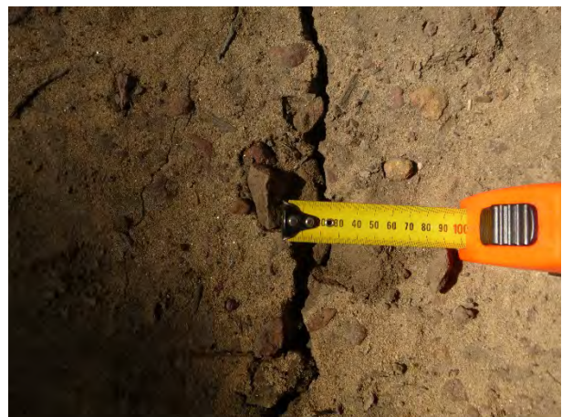
Photo 5: DA3B_LW16_014 , looking at the width of soil cracking. Taken on 12/05/2020.
