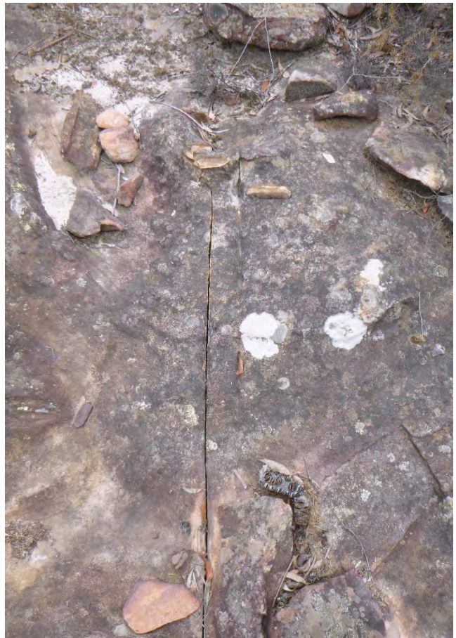
Photo 7: DA3B_LW16_010, an overview of the rock fracture. Taken on 27/04/2020.
