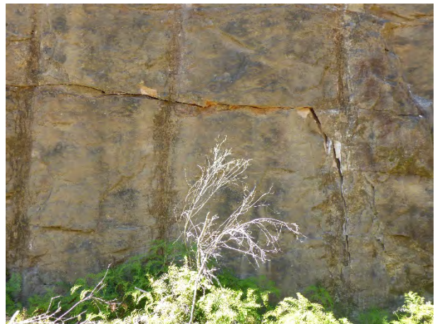
Photo 2: DA3B_LW16_022 , looking at a section of rock fracturing. Taken on 6/08/2020.
