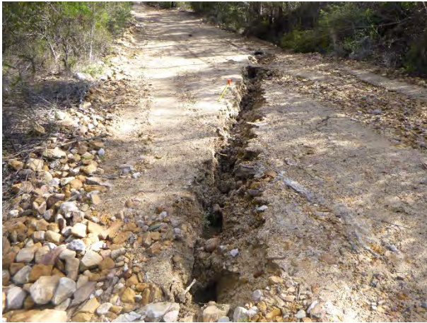
Photo 6: DA3B_LW16_013, looking at a section of soil cracking. Taken on 28/05/2020.
