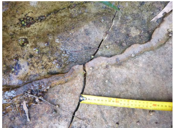
Photo 2: DA3B_LW16_028- rock fracture across rockbar. Taken on 31/08/2020.
