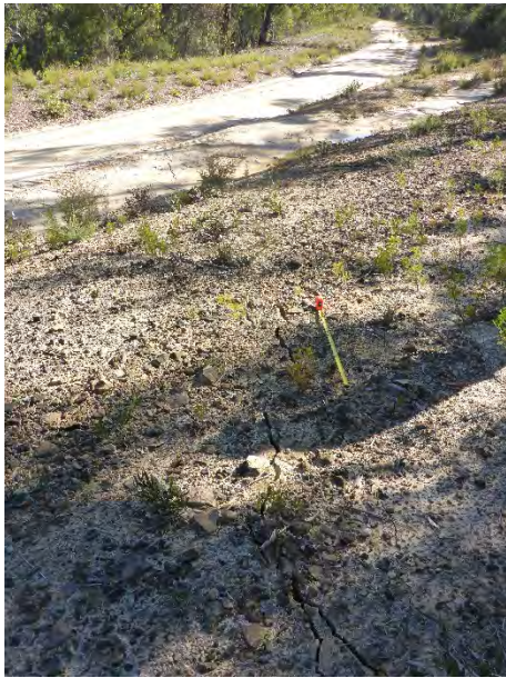
Photo 3: DA3B_LW16_019, looking at a section of soil cracking. Taken on 25/06/2020.
