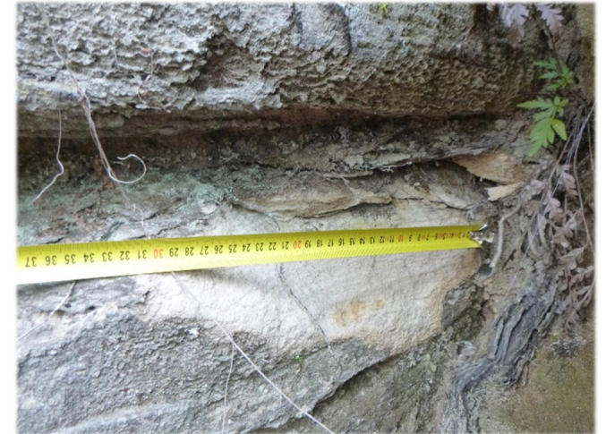
Photo 20: DA3B_LW15_021, looking at the area of rockfall. Taken on 27/02/2020.
