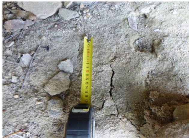
Photo 25: DA3B_LW15_026, looking at the soil cracking. Taken on 27/02/2020.
