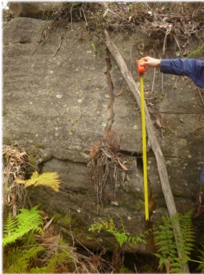
Photo 12: DA3B_LW15_007 , looking at fracturing on the step. Taken on 26/02/2020
