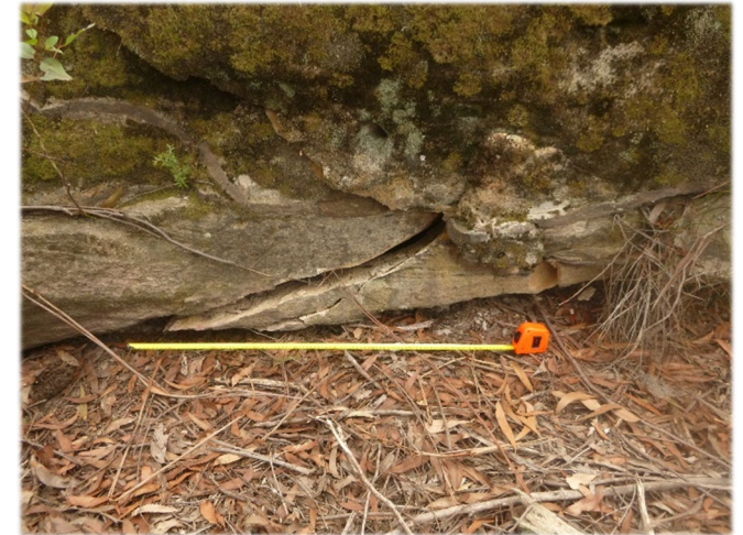
Photo 14: DA3B_LW15_013 , looking at a section of rock fracturing. Taken on 26/02/2020
