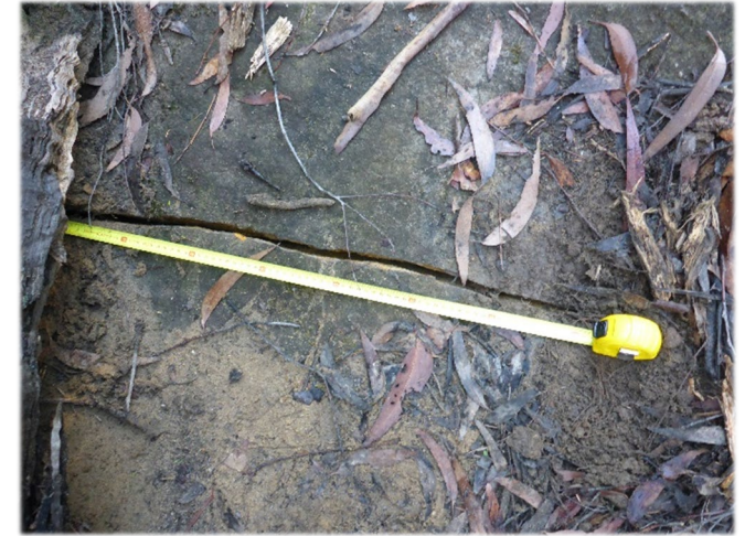
Photo 11: DA3B_LW15_006 , looking at the rock fracture. Taken on 09/07/2019.
