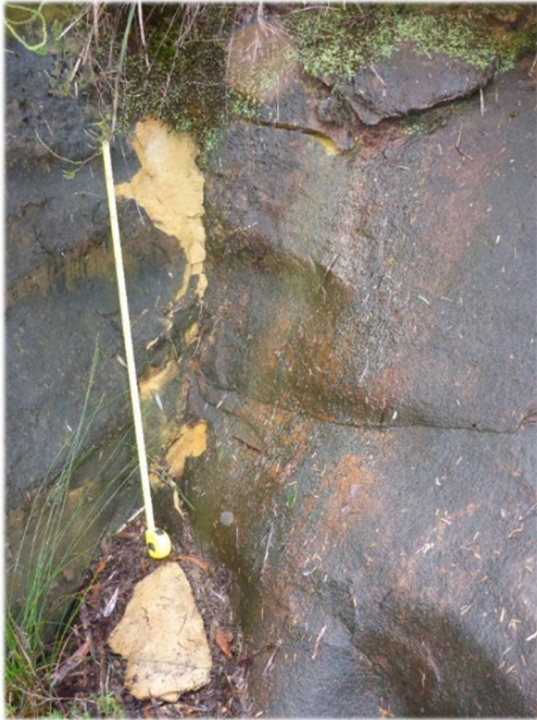
Photo 1: DA3B_LW15_003, looking at fracturing and dislodged rock segments. Taken on 17/06/2019.
