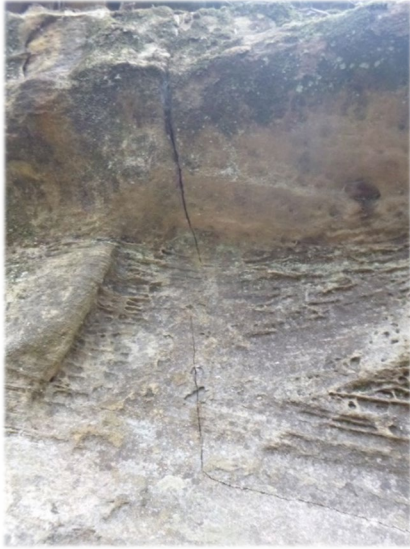
Photo 21: DA3B_LW15_022, looking at the rock fracture. Taken on 27/02/2020.
