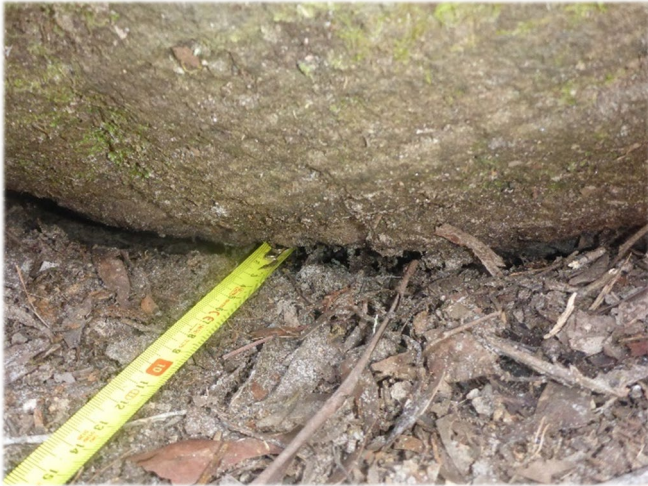
Photo 15: DA3B_LW15_016, looking at the width of displacement. Taken on 25/10/2019.
