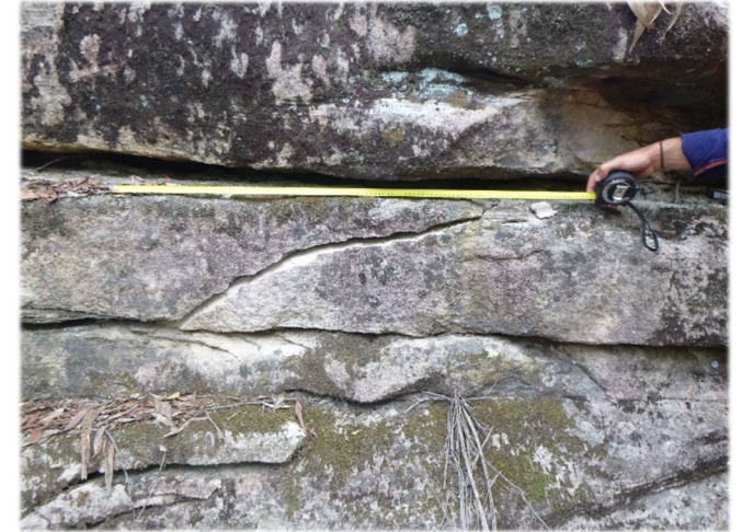
Photo 17: DA3B_LW15_018, looking at the rock fracture. Taken on 27/02/2020.
