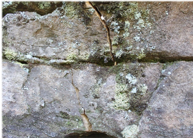
Photo 32: DM 21, Two vertical fractures located at the northern exterior of the shelter cavern area. Taken: 15th March 2020.
