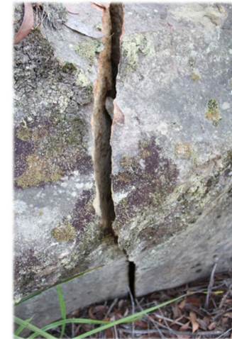
Photo 33: DM 21, Close up of vertical fracturing located at the base of the northern exterior of the shelter cavern area. Taken: 15th March 2020.
