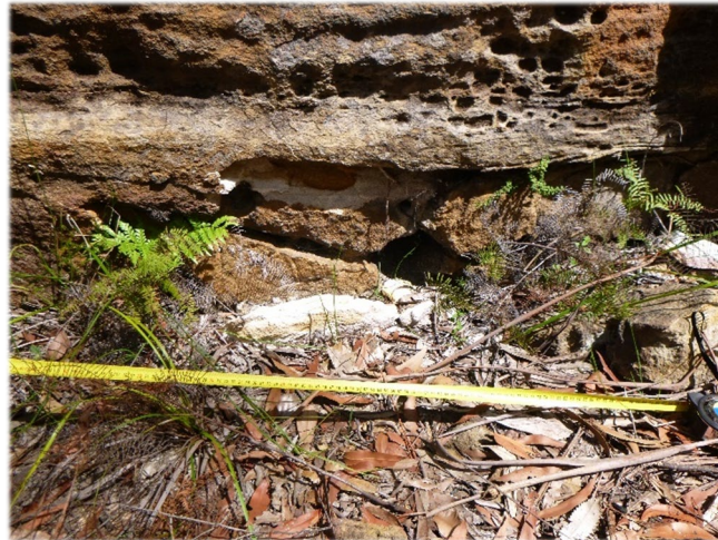
Photo 19: DA3B_LW15_020, looking at area of rockfall. Taken on 27/02/2020.
