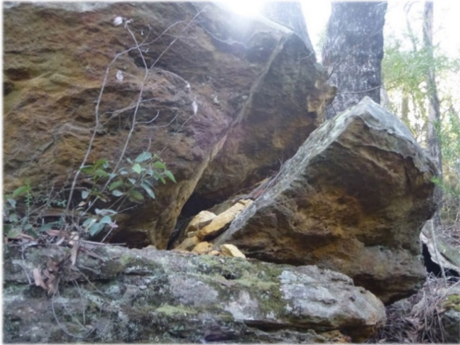
Photo 9: DA3B_LW15_001 , looking at a section of the rockfall. Taken on 29/05/2019.
