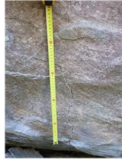
Photo 23: DA3B_LW15_024, looking at the rock fracturing. Taken on 21/01/2020.
