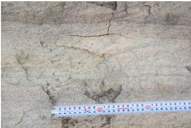
Plate 12: Fissuring above Art Panel to the south of the shelter.
