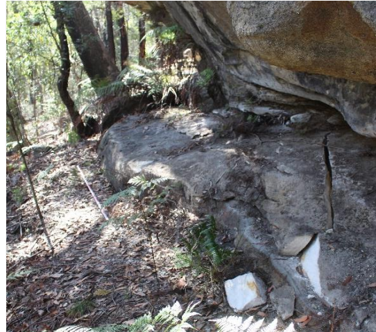
Plate 5: Comparison photo from Niche (2019) Longwall 14 monitoring of cracking and minor block fall at the south end of the shelter facing south.
