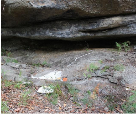
Plate 4: Location of crack 1 and 2 facing west.
