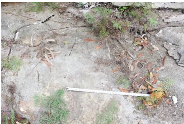
Plate 7: Location of cracks 5 and 6 from an aerial aspect.
