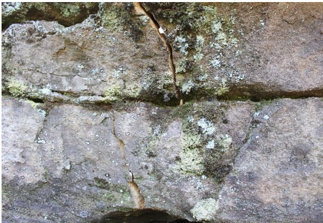
Plate 37: Two new instances of vertical cracking located northern exterior of the shelter cavern area.
