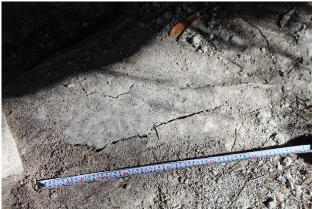
Plate 18: New floor cracking in the southern end of the shelter.
