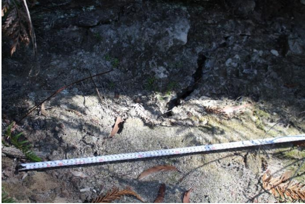
Plate 11: Soil displacement over suspected crack 7.
