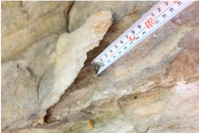
Plate 19: Flaking of sandstone the southern back wall of the shelter.
