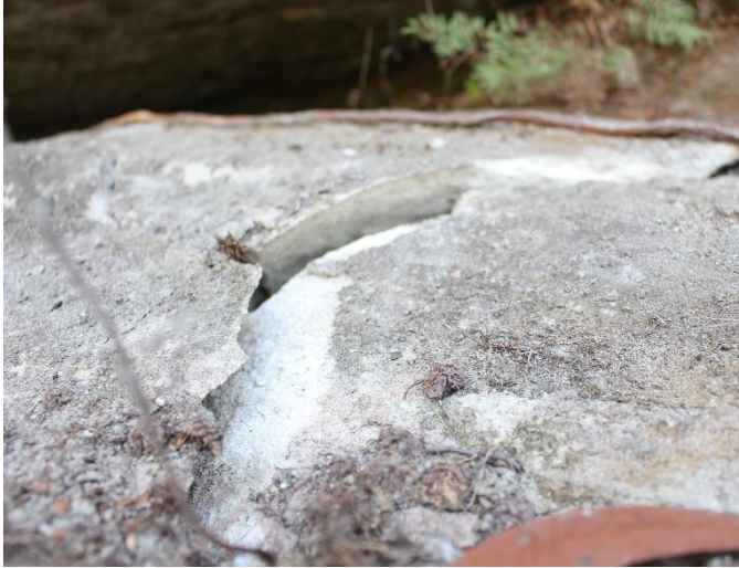
Plate 8: Convergent slip of rock platform at crack 3.
