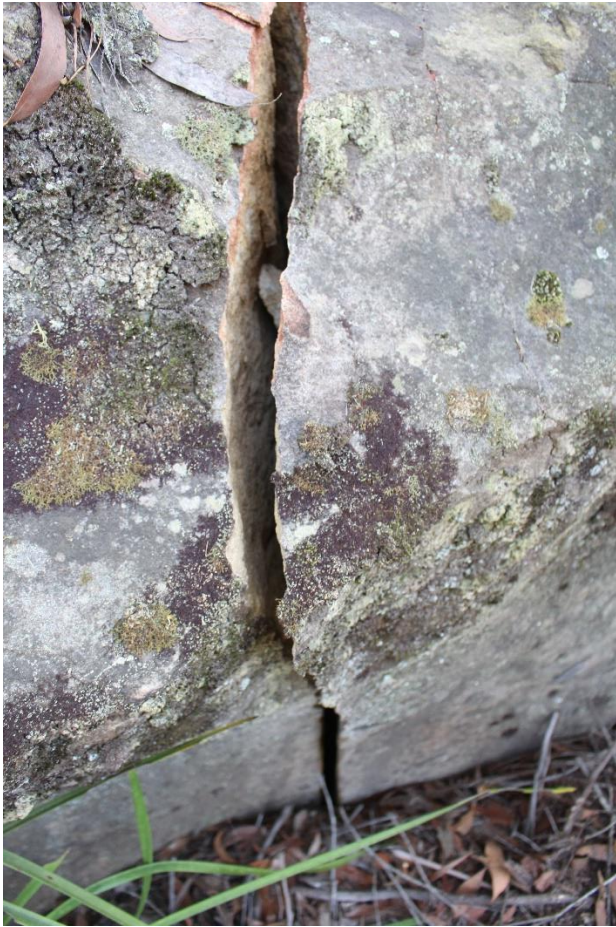
Plate 38: Close up of vertical cracking located at the base of the northern exterior of the shelter cavern area.
