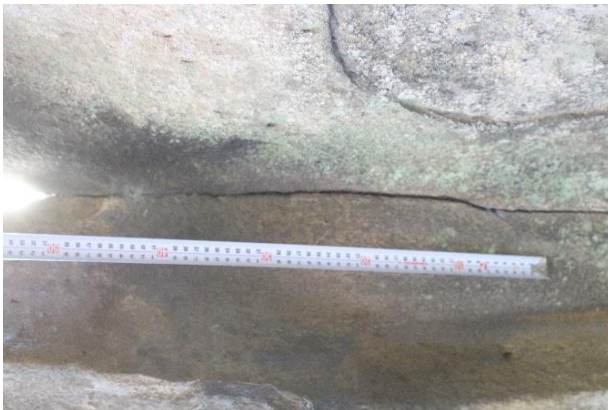
Plate 33: Natural fissuring located on southern extent of the shelter.
