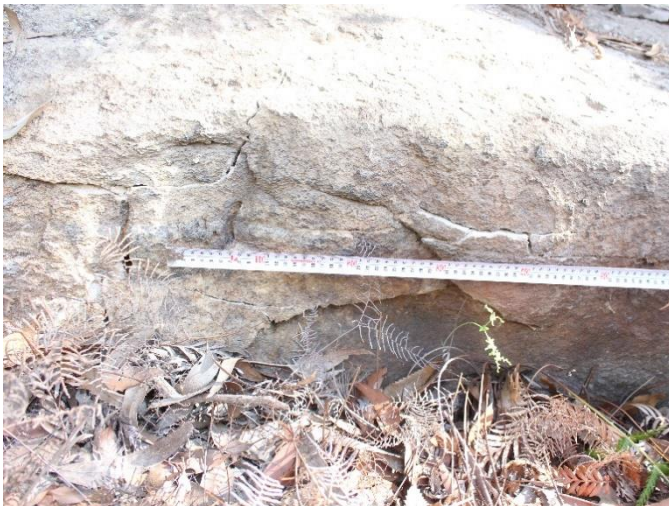
Plate 9: Many minor cracks at the base of shelter below crack 4.
