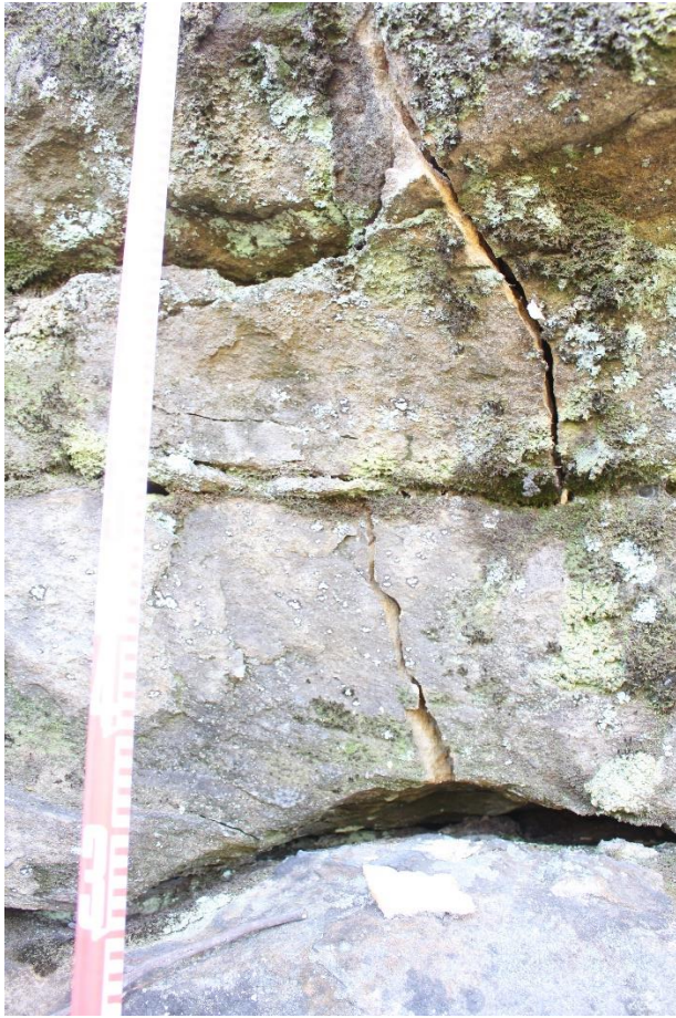
Plate 39: Close up of diagonal cracking located northern exterior of the shelter cavern area.
