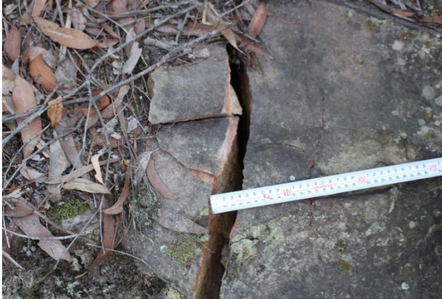
Plate 35: Close up of vertical cracking located northern exterior of the shelter cavern area.
