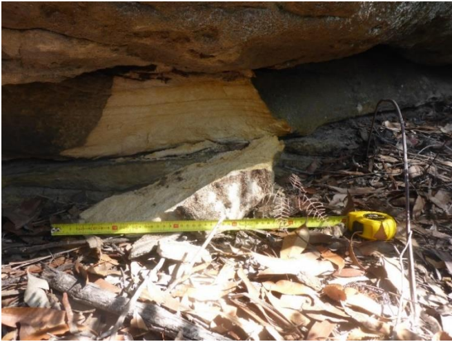
Photo 66: DA3B_LW15_017, looking at the area of rockfall. Taken on 25/10/2019.
