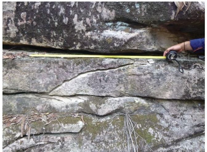
Photo 69: DA3B_LW15_018, looking at the rock fracture. Taken on 27/02/2020.
