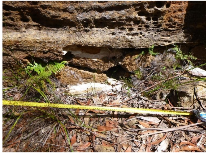
Photo 74: DA3B_LW15_020, looking at area of rockfall. Taken on 27/02/2020.
