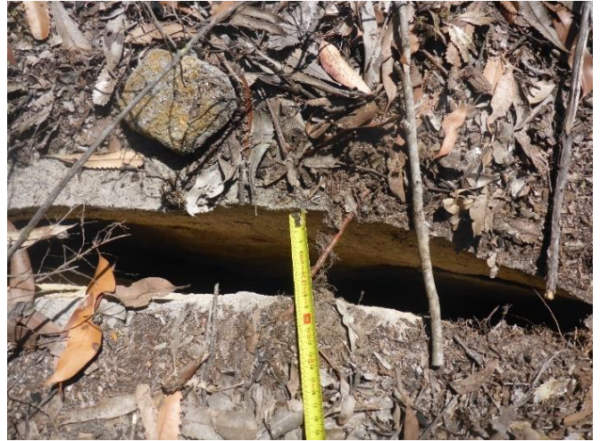
Photo 81: DA3B_LW15_023, looking at width of rock fracture. Taken on 25/10/2019.
