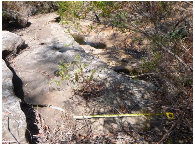
Photo 32: DA3B_LW14_016, looking at the rock fracture and displacement. Taken on 21/01/2020.
