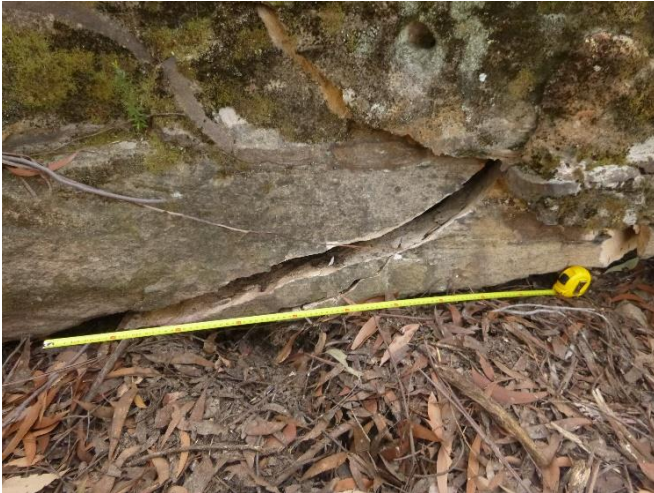
Photo 60: DA3B_LW15_013, looking at a section of rock fracturing. Taken on 05/09/2019.
