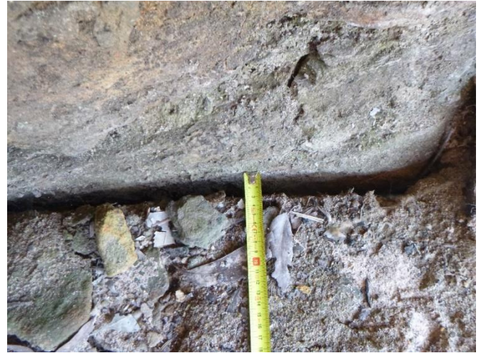
Photo 91: DA3B_LW15_026, looking at width of soil displacement. Taken on 21/01/2020.
