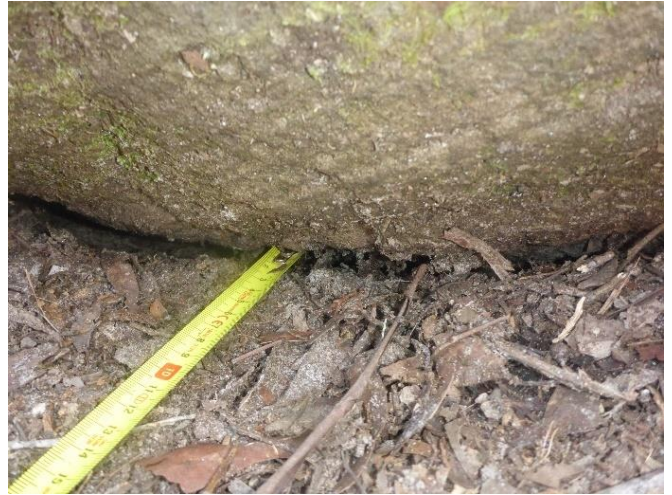
Photo 64: DA3B_LW15_016, looking at the width of displacement. Taken on 25/10/2019.
