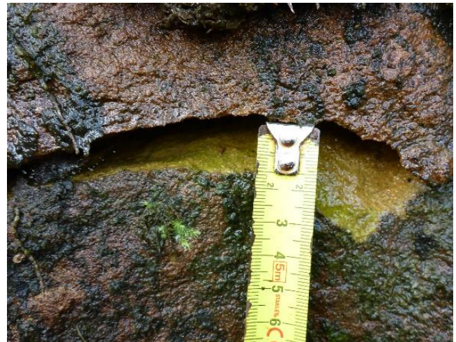
Photo 6: DA3B_LW15_003, looking at a section of rock fracturing. Taken on 17/06/2019.
