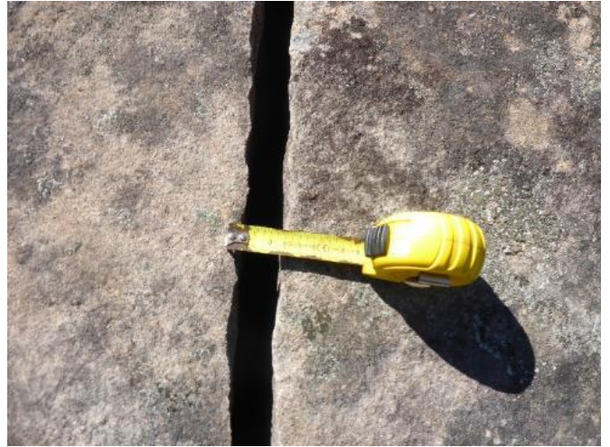
Photo 101: DA3A_LW7_001, looking at width of cracking. Taken on 20/08/2019.
