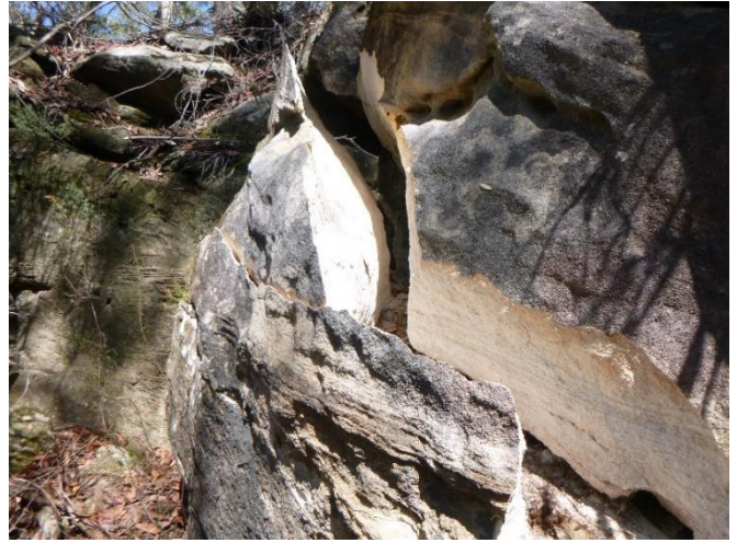
Photo 87: DA3B_LW15_025, looking at the rockfall. Taken on 21/01/2020.
