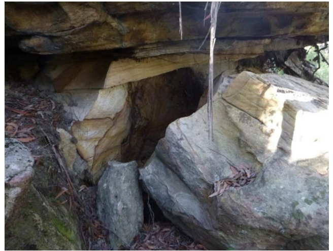
Photo 49: DA3B_LW15_002, looking at the rockfall. Taken on 29/05/2019.
