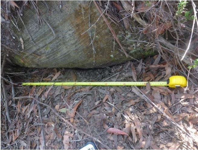
Photo 63: DA3B_LW15_016, looking at a section of displacement. Taken on 25/10/2019.
