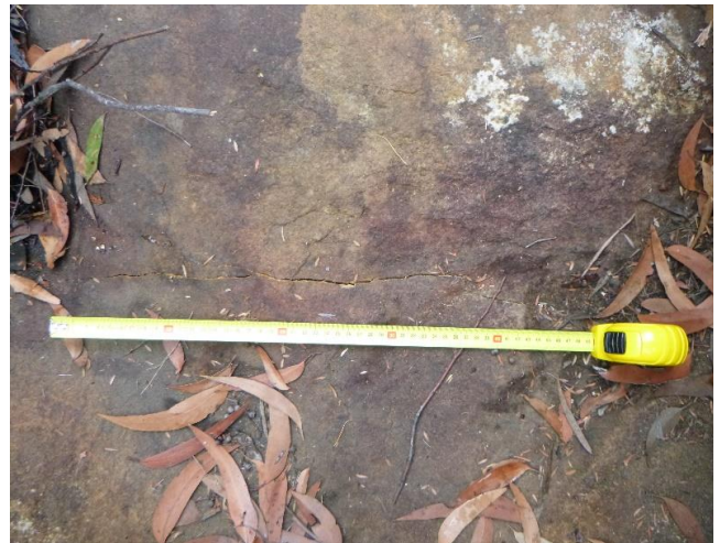
Photo 13: DA3B_LW15_015 , looking at a section of rock fracturing. Taken on 11/10/2019.
