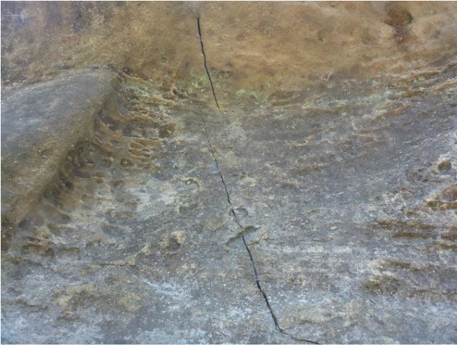
Photo 77: DA3B_LW15_022, looking at rock fracture. Taken on 25/10/2019.
