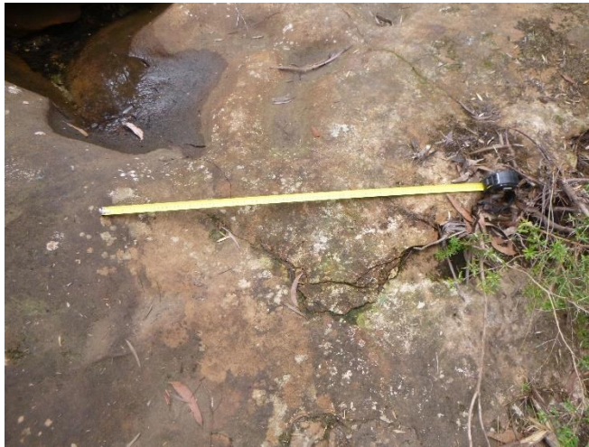
Photo 14: DA3B_LW15_015, looking at a section of rock fracturing. Taken on 02/27/2020.
