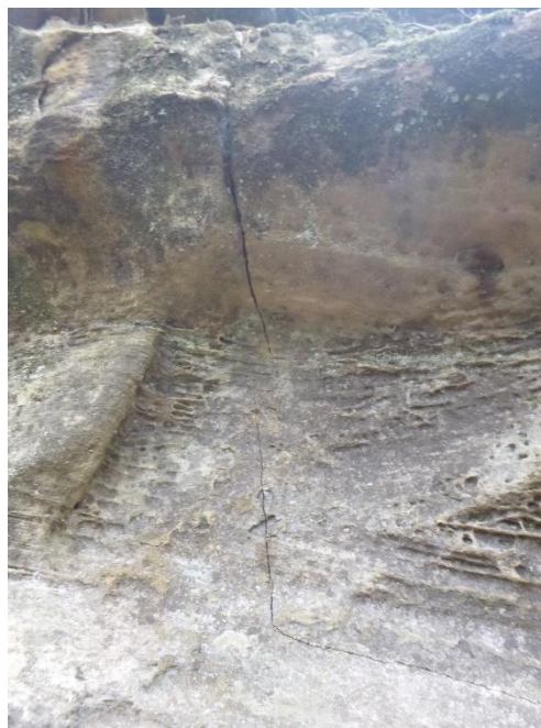
Photo 79: DA3B_LW15_022, looking at rock fracture. Taken on 27/02/2020.
