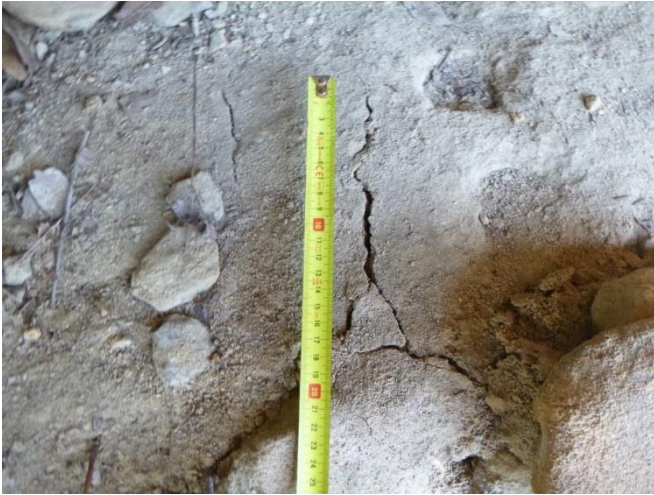
Photo 90: DA3B_LW15_026, looking at soil cracking. Taken on 21/01/2020.
