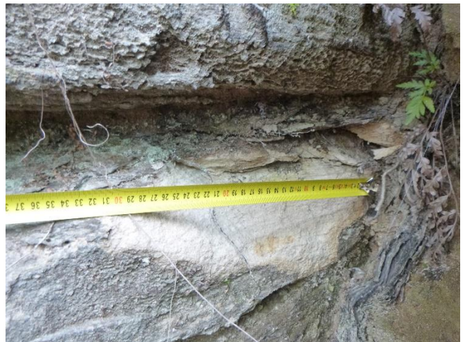
Photo 76: DA3B_LW15_021, looking at the area of rockfall. Taken on 27/02/2020.
