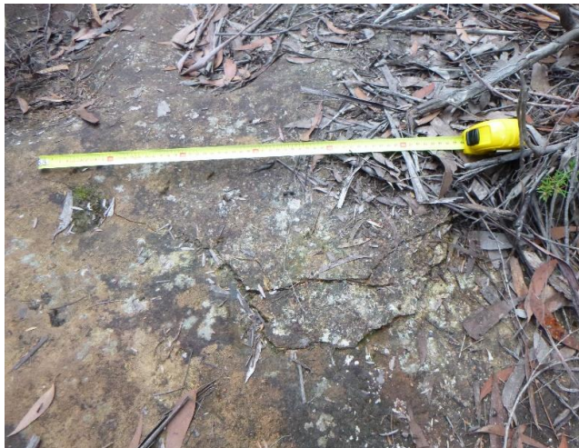
Photo 12: DA3B_LW15_015 , looking at a section of rock fracturing. Taken on 11/10/2019.
