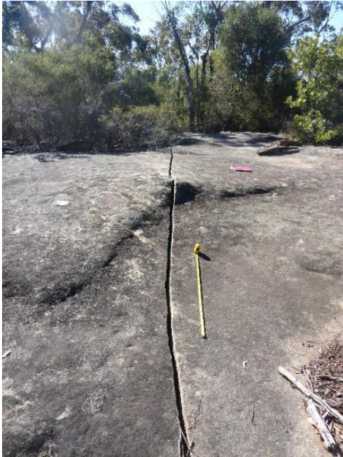
Photo 100: DA3A_LW7_001, looking at section of cracking. Taken on 20/08/2019.
