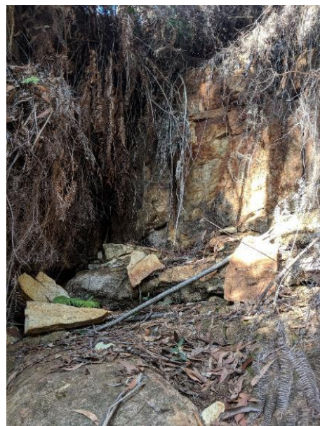
Photo 16: DA3B_LW13_010, showing rockfall at step. Taken on 21/08/2019.
