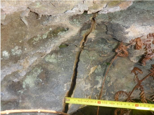
Photo 70: DA3B_LW15_019, looking at width of rock fracture. Taken on 25/10/2019.
