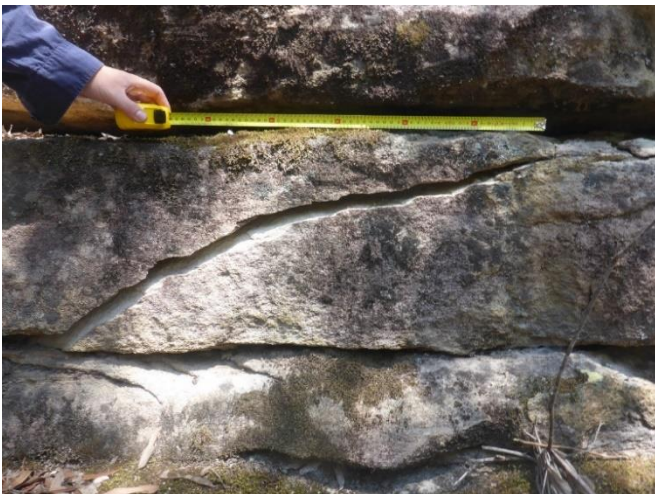
Photo 68: DA3B_LW15_018, looking at the rock fracture. Taken on 25/10/2019.
