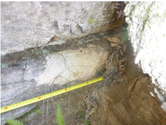
Photo 75: DA3B_LW15_021, looking at the area of rockfall. Taken on 25/10/2019.
