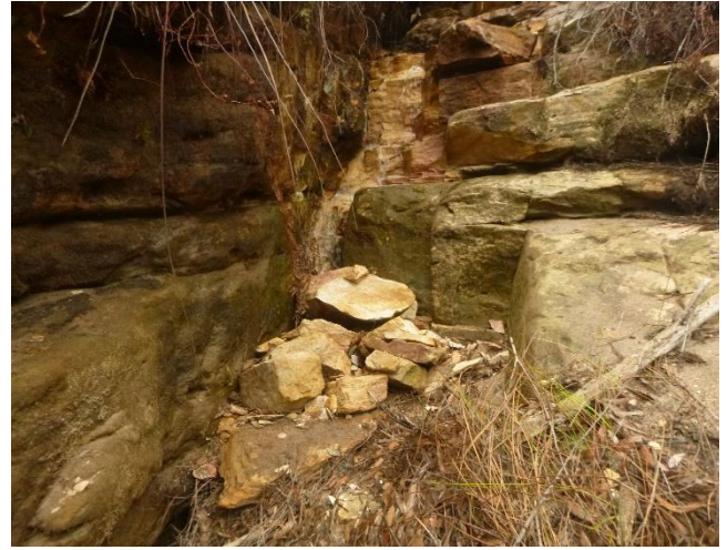
Photo 18: DA3B_LW13_010, showing rockfall at step. Taken on 26/02/2020.
