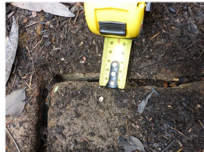
Photo 3: DA3B_LW14_018, looking at the width of the fracturing. Taken 20/02/2019.
