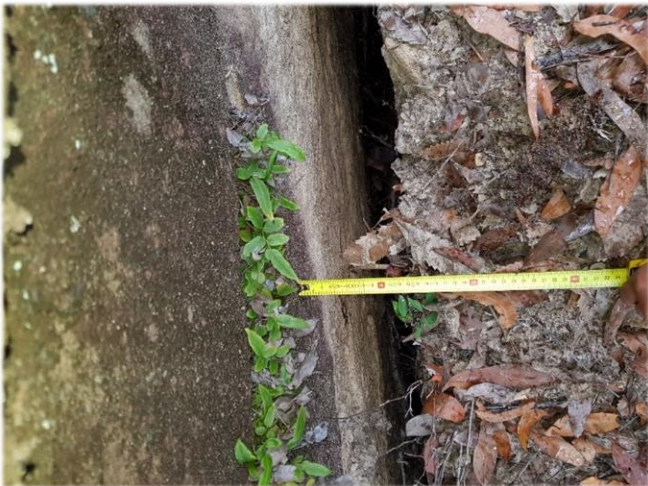
Photo 18: DA3B_LW14_026, looking at the width of the fracturing. Taken 10/05/2019.
