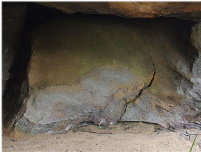
Photo 19: DA3B_LW14_027, looking at a section of rock fracturing. Taken 10/05/2019.
