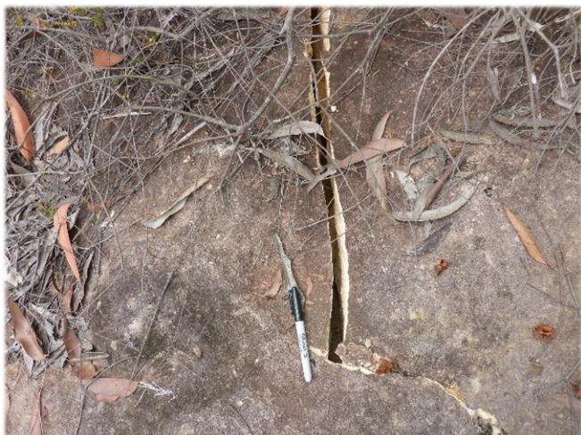
Photo 4: DA3B_LW14_019, looking at a section of rock fracturing. Taken 20/02/2019.
