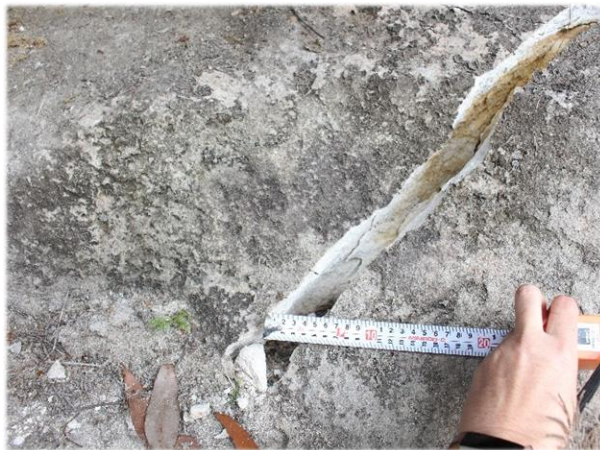
Photo 22: Subsidence cracking at the west end of the Browns Road Site 11 shelter. Taken: 10 th May 2019.
