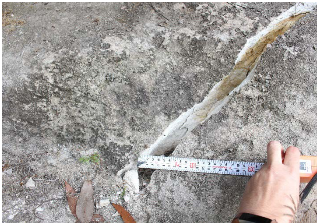
Plate 5: Subsidence cracking at the western end of the shelter.
