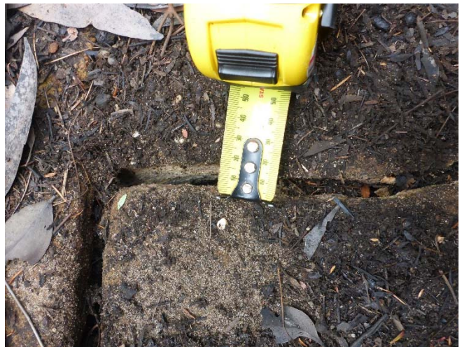
Photo 4: DA3B_LW14_018, looking at the width of the fracturing. Taken 20/02/2019.
