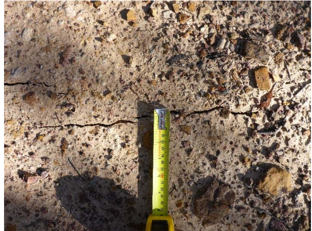
Photo 2: Impact DA3B_LW14_001, largest crack width. Taken on 3/7/18.
