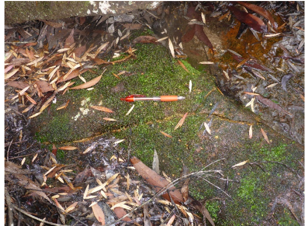
Photo 9: Fracturing at base of step. Taken on 21/01/2019.
