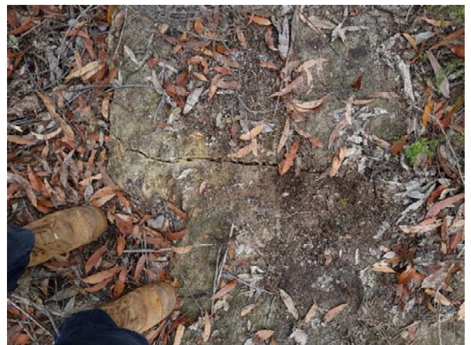
Photo 7: DA3B_LW14_028, looking at a section of rock fracturing. Taken 10/05/2019.
