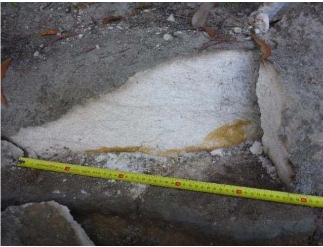
Photo 3: DA3B_LW14_024, looking at the area of the rockfall. Taken 09/04/2019.
