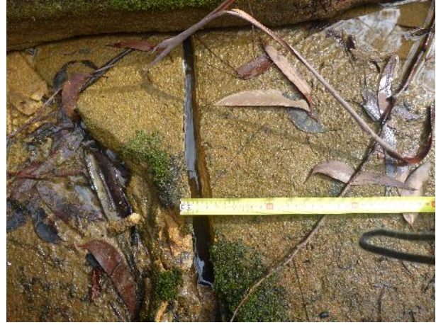
Photo 8: Impact DA3b_LW13_045. Taken on 8/07/18.
