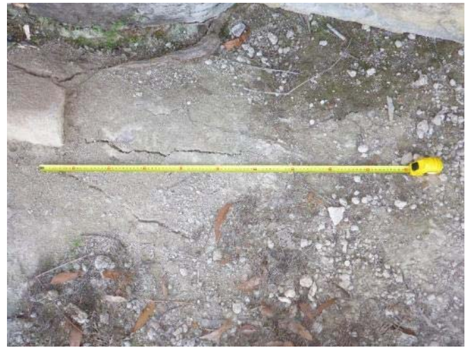
Photo 4: DA3B_LW14_024, looking at a section of soil cracking. Taken 09/04/2019.
