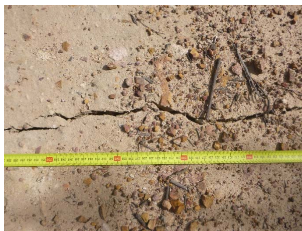
Photo 2: Impact DA3B_LW14_004. Taken on 13/08/18.
