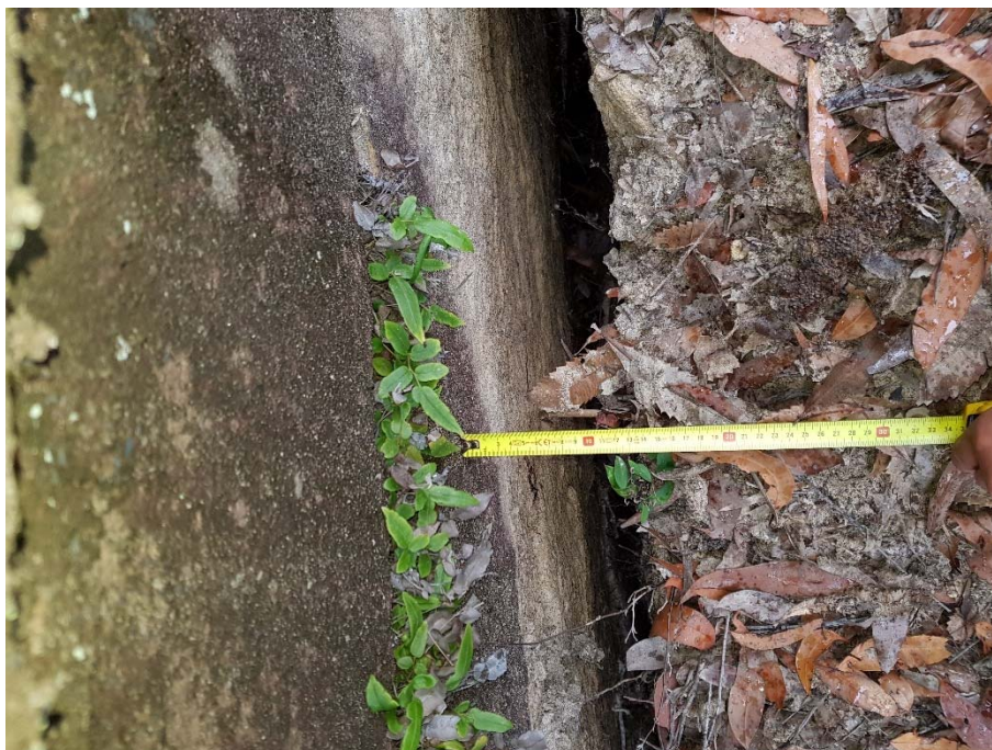
Photo 1: DA3B_LW14_026 , looking at the width of the fracturing. Taken 10/05/2019.
