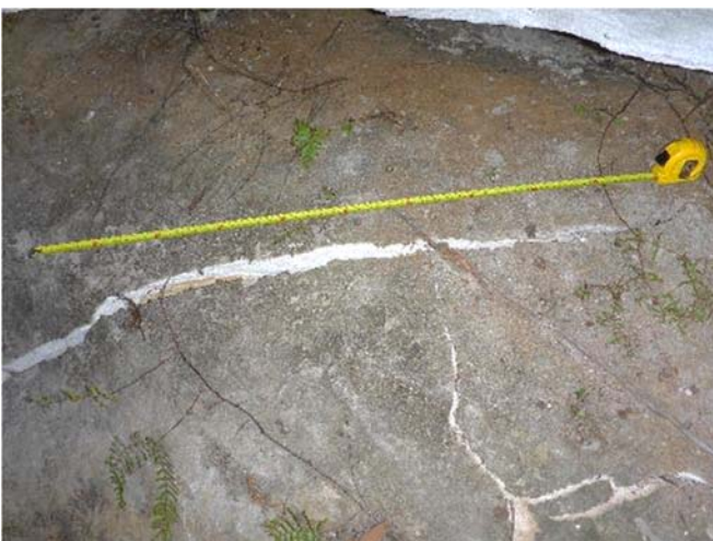
Photo 1: DA3B_LW14_024 , looking at a section of rock fracturing. Taken 09/04/2019.
