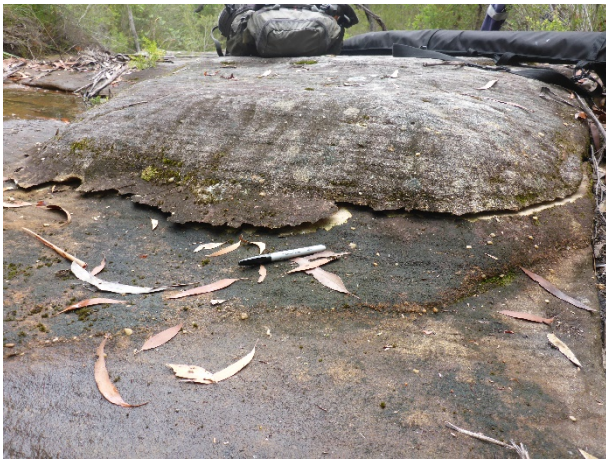
Photo 1: Circular fracture and uplift on rockbar. Taken on 21/01/2019.
