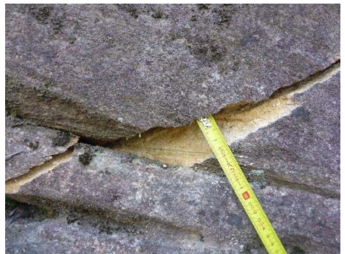
Photo 6: DA3B_LW14_025, looking at the width of the rock fracturing. Taken 09/04/2019.
