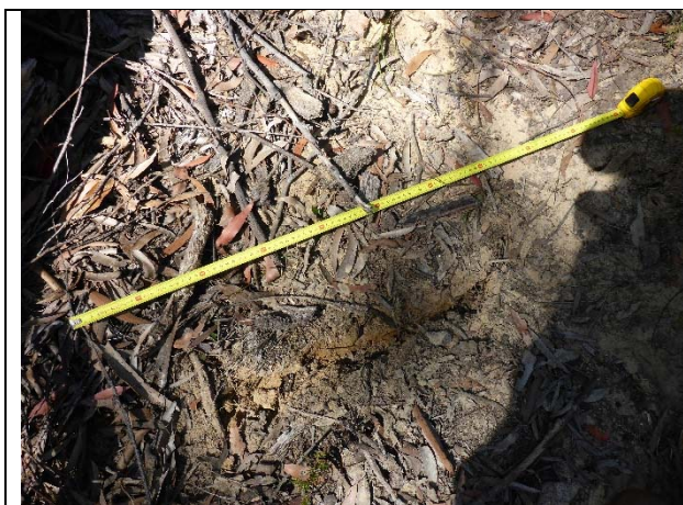
Photo 1: Impact DA3B_LW14_014, soil cracking. Taken on 13/11/2018.
