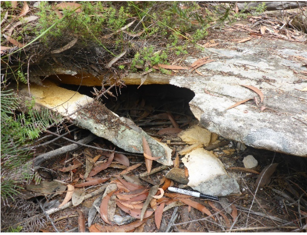
Photo 10: Fracturing and dislodged rock segment to incised step. Taken on 21/01/2019.
