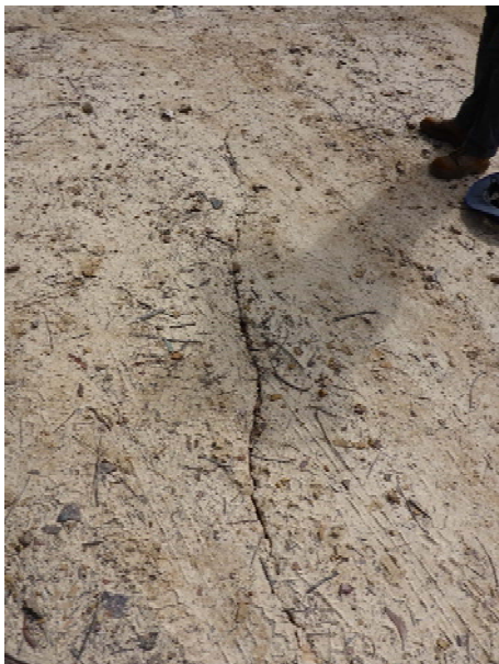
Photo 9: Impact DA3B_LW14_008. Taken on 28/08/18.
