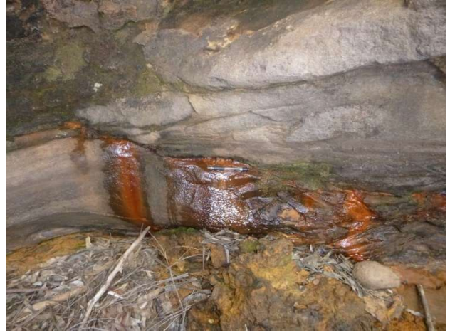
Photo 4: DA3B_LW13_043, looking at iron staining. Taken on 6 December 2018.
