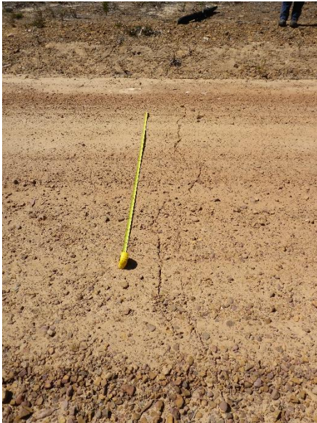
Photo 5: Impact DA3B_LW14_012. Taken on 16/09/18.
