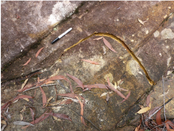
Photo 3: Fracturing to rockbar. Taken on 21/01/2019.
