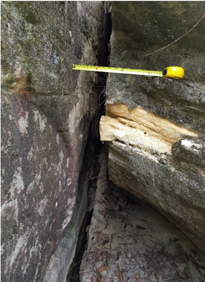
Photo 2: DA3B_LW14_026, section of rock fracturing and displacement. Taken 10/05/2019.
