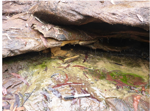
Photo 4: Fracturing with flow diversion across small step on rockbar. Taken on 21/01/2019.
