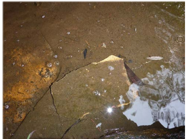
Photo 32: DA3B_LW13_042, looking at a section of new rock fracturing. Taken 01/04/2019.
