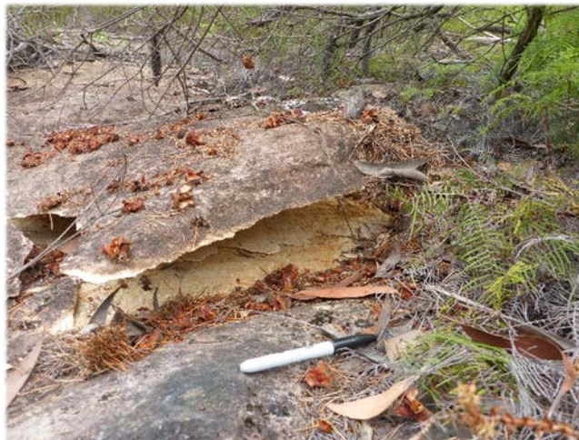
Photo 19: DA3B_LW14_019, looking at a section of uplift. Taken 20/02/2019.
