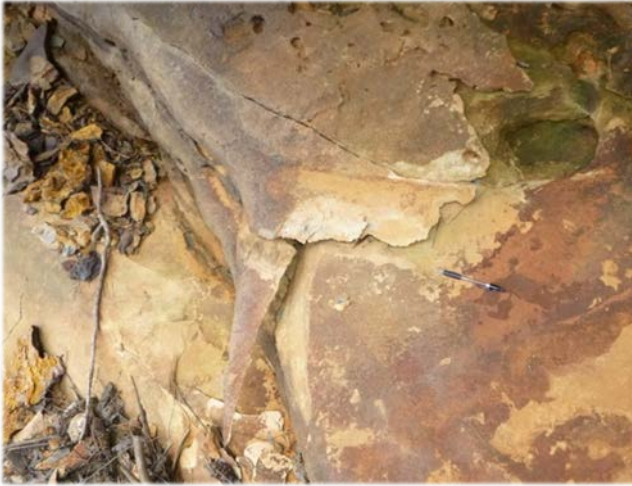
Photo 7: DA3B_LW13_043, looking at a section of rock fracturing and uplift. Taken 6/12/2018
