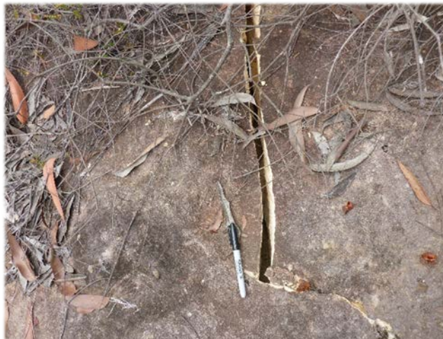
Photo 20: DA3B_LW14_019, looking at a section of rock fracturing. Taken 20/02/2019.
