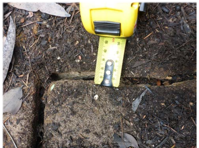
Photo 18: DA3B_LW14_018, looking at the width of the fracturing. Taken 20/02/2019.
