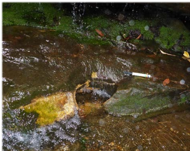
Photo 11: DA3B_LW13_046, looking at the extent of the rock fracturing. Taken 01/04/2019.
