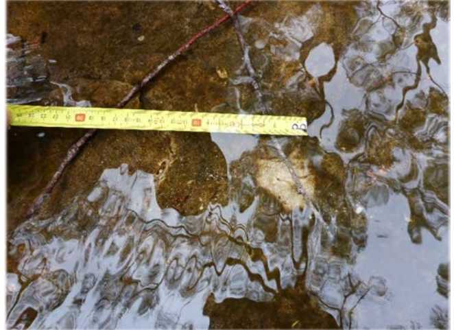
Photo 28: DA3B_LW14_023, looking at a section of rock fracturing. Taken 01/04/2019.
